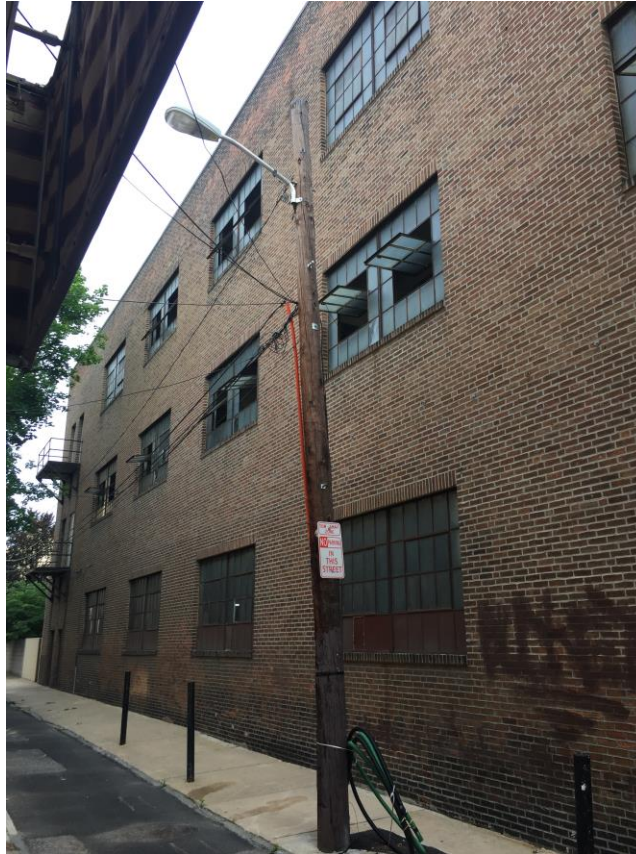
3. South elevation, view NW, from Addison St.; note fire escape landings at the west corner and operable pivot windows in industrial sash.
