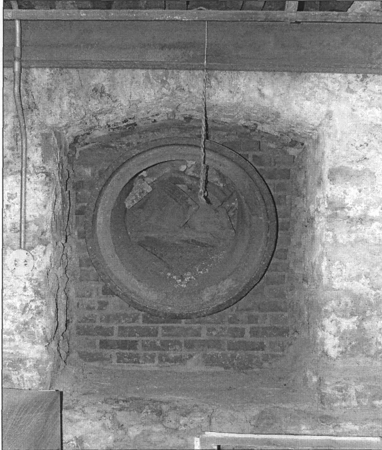
Figure 7: tile steam heat pipe, Jackson Street, building #13 (photo by J. Jacobsen, September 2007)
