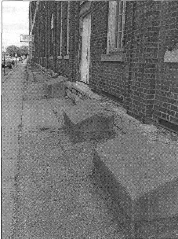
Figure 5: infilled basement windows and exterior window well, building #9, view north (photo by J. Jacobsen, September 2007)
