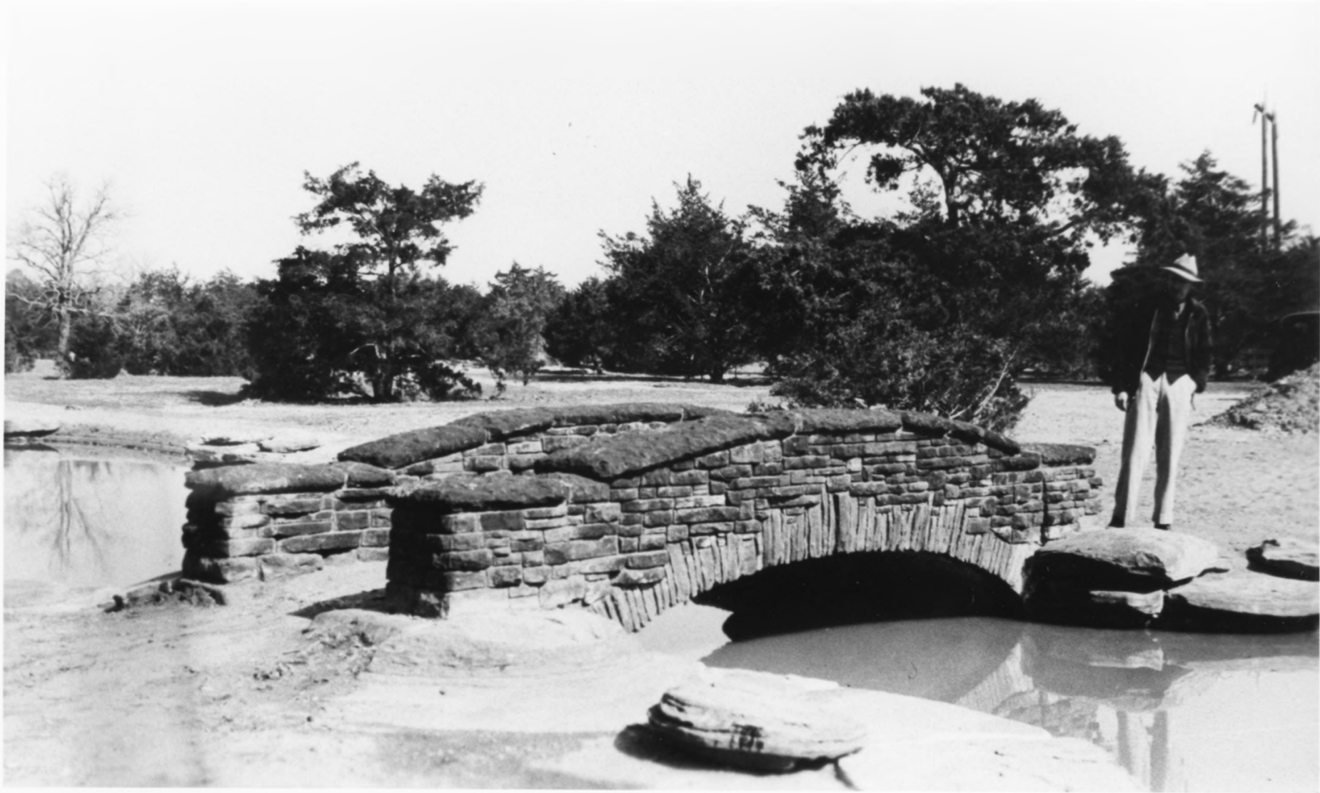
BASTROP STATE PARK Bastrop vic., Bastrop County, Texas Ornamental Bridge, Golf Course Photo: National Archives, ca. 1935
