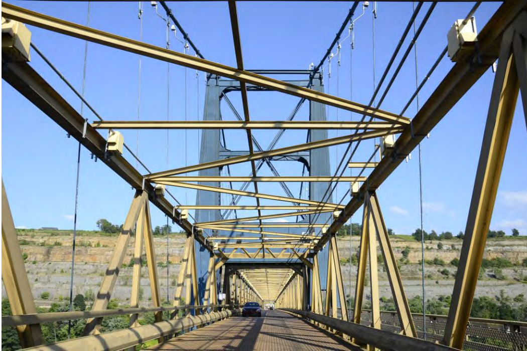
Photo 11: Market Street Bridge, Detail of the western side of the Ohio tower, facing east
