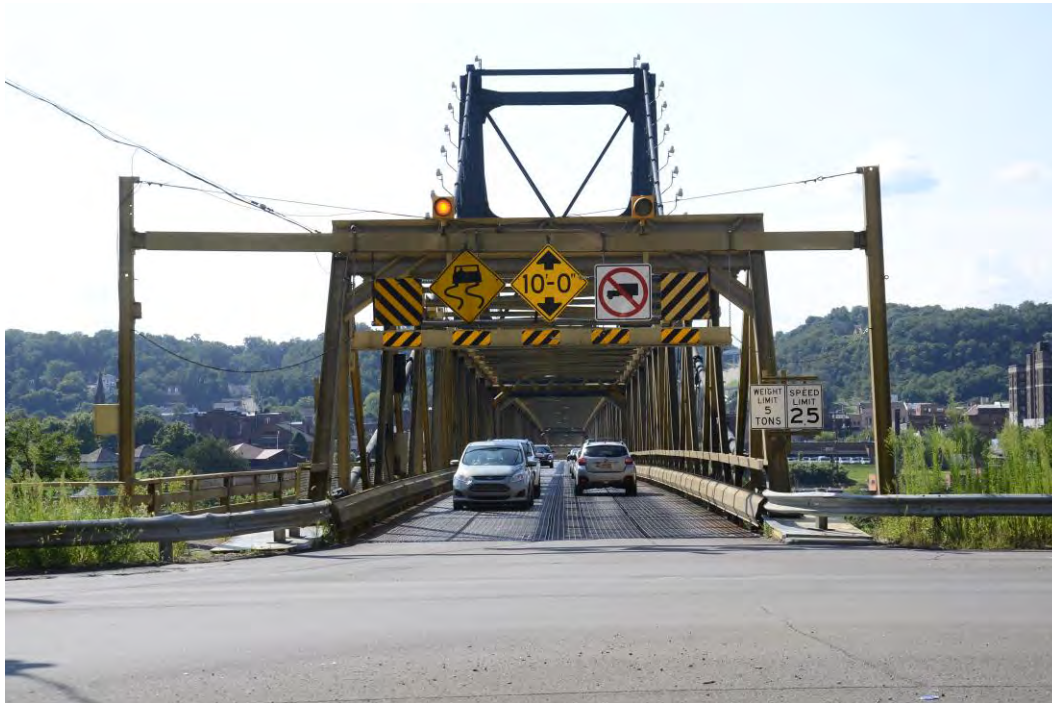
Photo 9: Market Street Bridge, approach on the WV (eastern) side of the river, facing west
