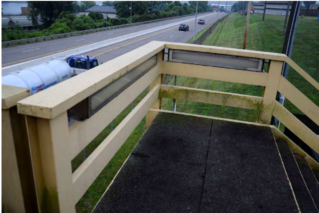
Photo 7: Market Street Bridge, Handrail & Stair landing, Note lighting under Handrail Cap, facing South
