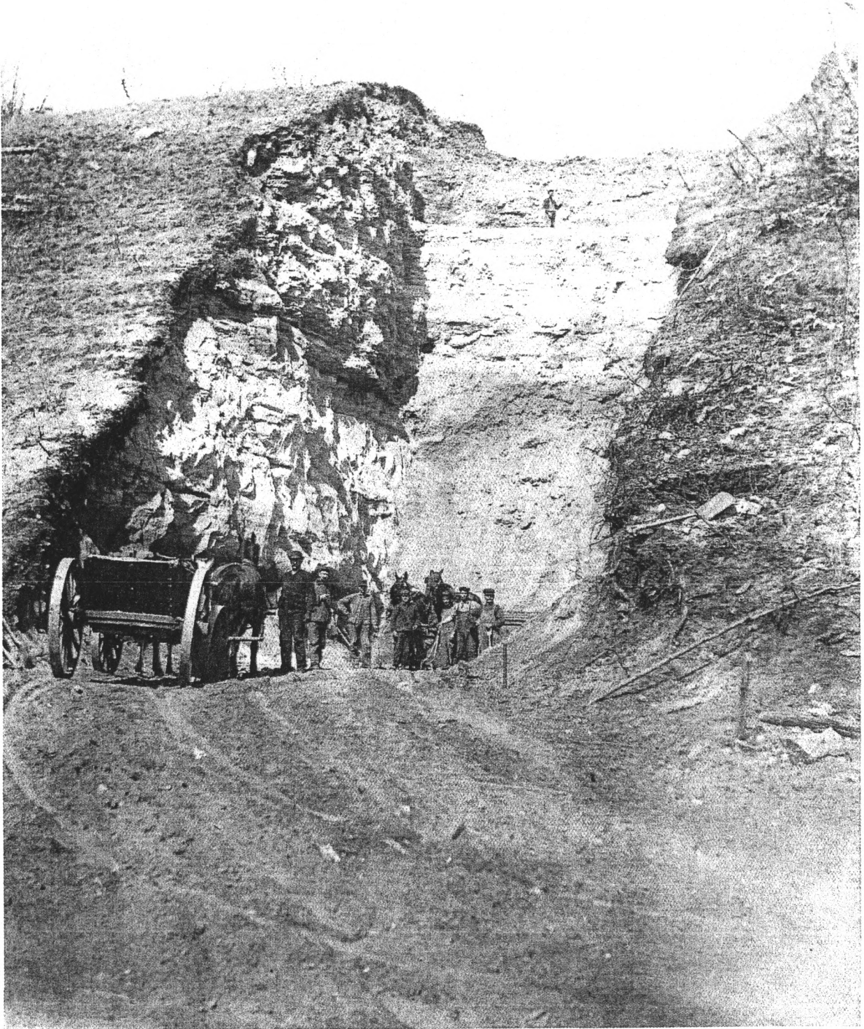
Mindoro Cut construction, Summer 1908, collection of John and Joan Dolbier, La Crosse County, WI
