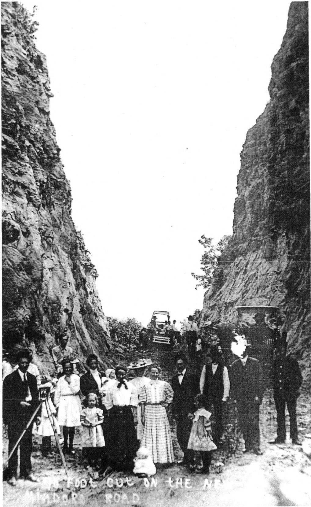
Mindoro Cut construction, Summer 1908, collection of John and Joan Dolbier, La Crosse County, WI
