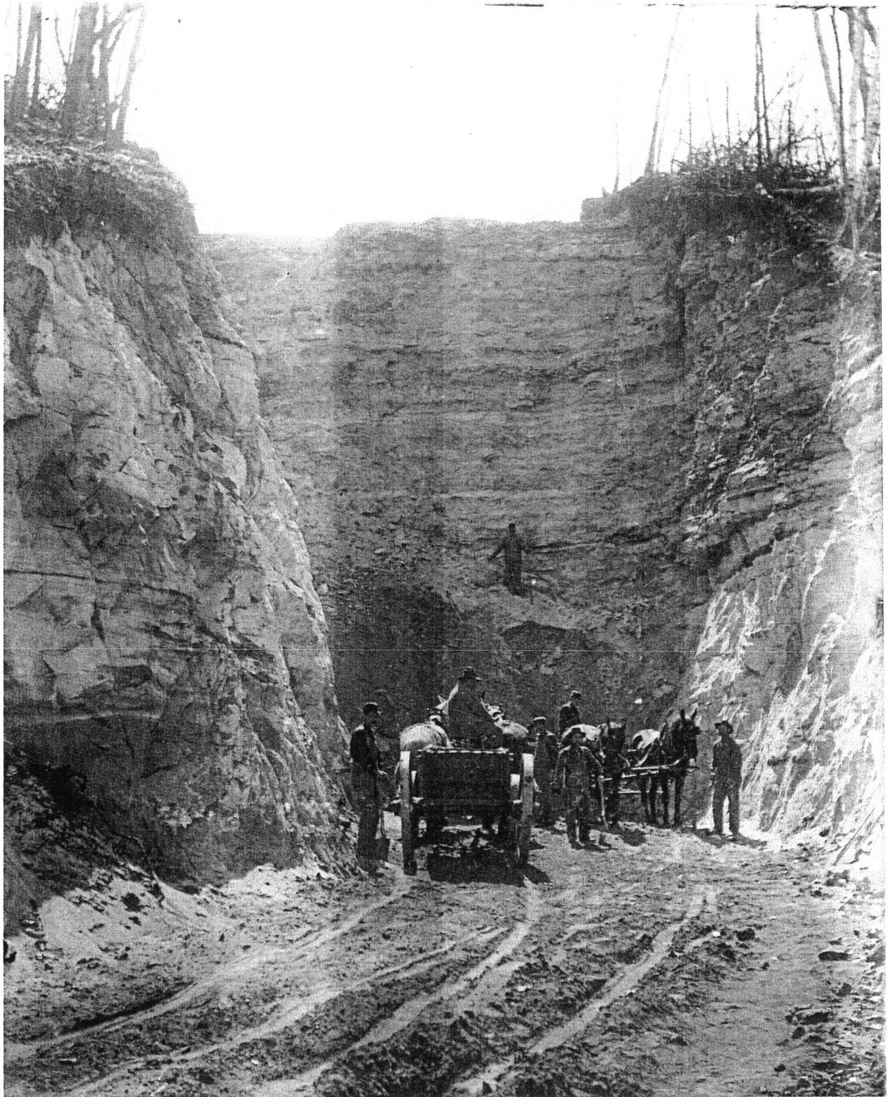
Setting dynamite during Mindoro Cut construction, summer 1908, collection of John and Joan Dolbier, La Crosse County, WI
