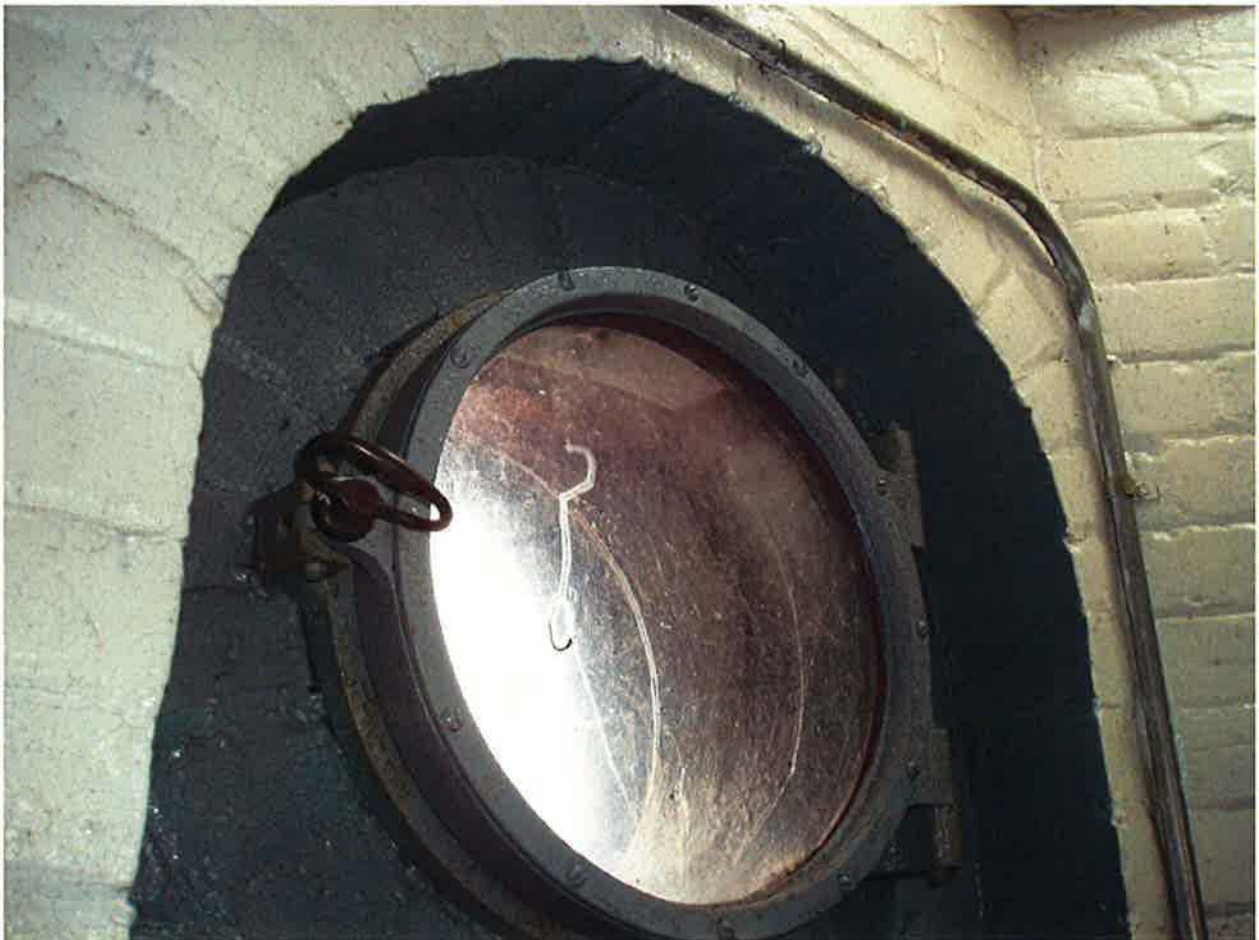
Photo 5. Light tower interior, second story port-light.
