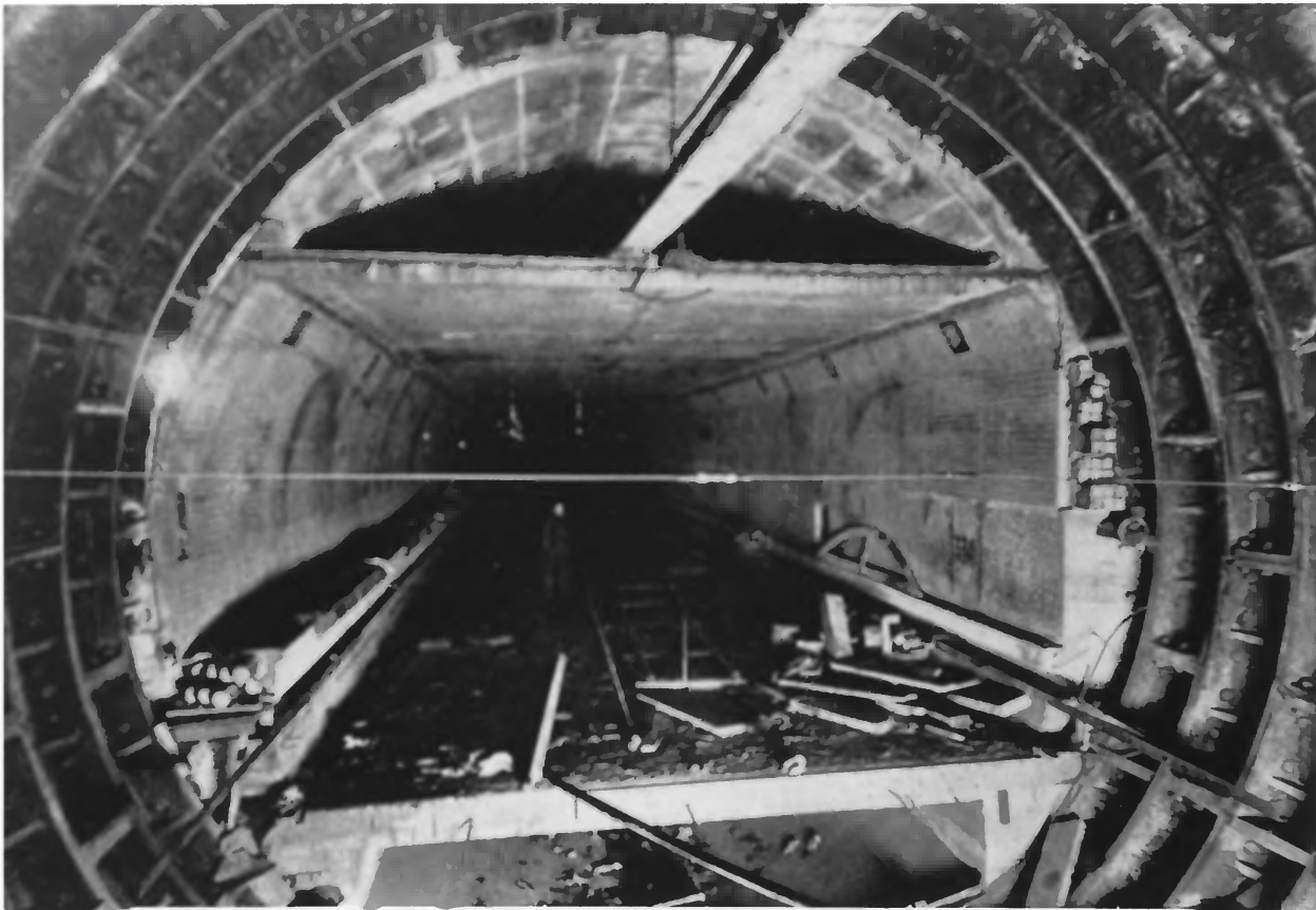
Photograph #1 Holland Tunnel New York County, NY & Hudson County, NJ Concrete Construction Within Cast Iron Tunnel Lining Gray's, The Eighth Wonder , 1927
