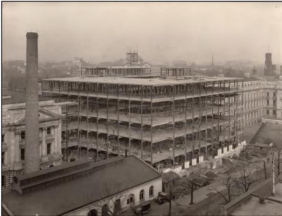
Figure 20: Center block under construction, south court, December 1928 Source: National Agriculture Library, USDA Construction Photos
