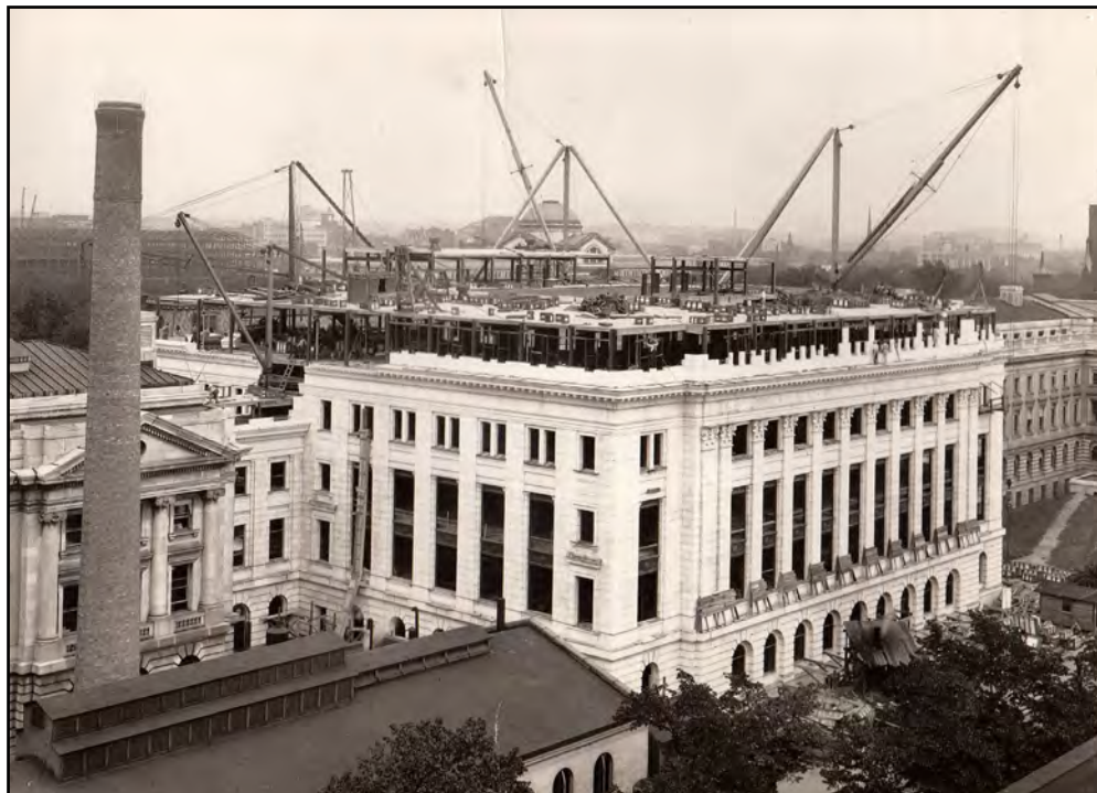
Figure 23: Center block under construction, south court, July 1929 Source: National Agriculture Library, USDA Construction Photos
