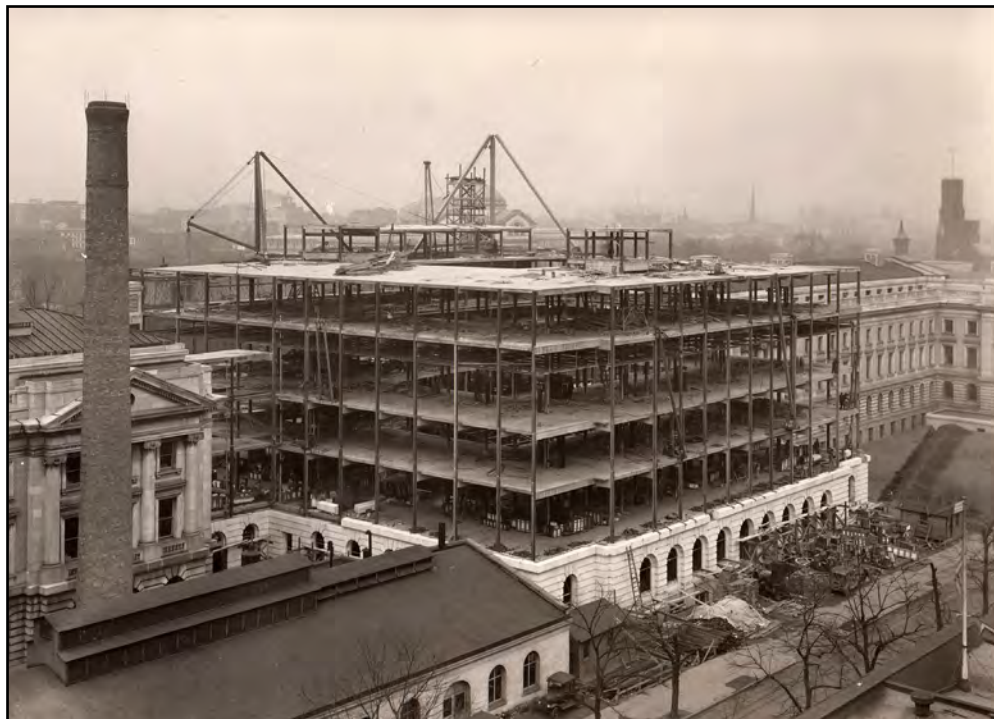
Figure 21: Center block under construction, south court, March 1929 Source: National Agriculture Library, USDA Construction Photos
