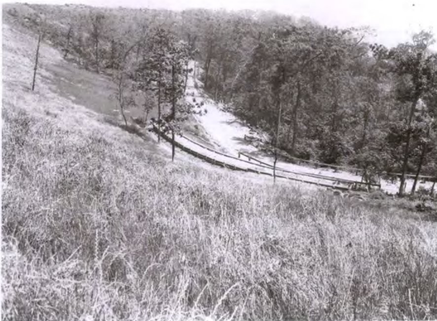
NJ_Monmouth County_Navesink Military Reservation_H64. Access Road A, Retaining Wall, view east, c1944, GATE
