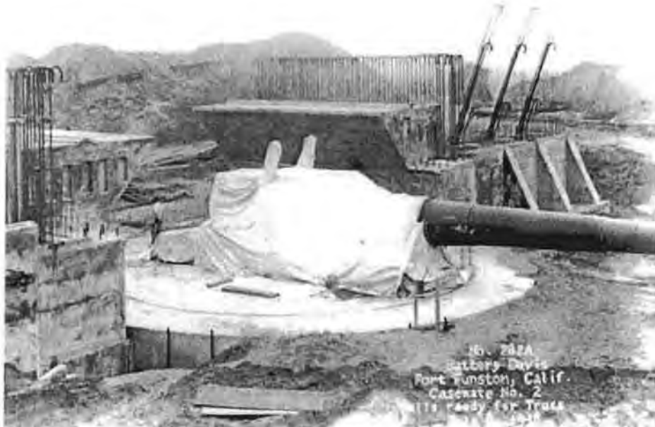
20. Construction of central traverse magazine in 1938, at Battery Richmond P. Davis. NARA Photo
