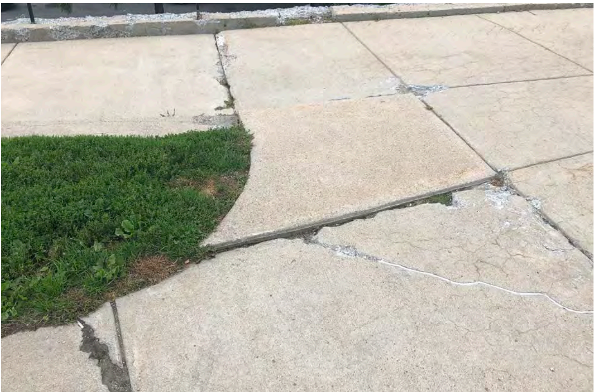
(top and bottom) Figures 3-28 and 3-29: Sample conditions of walkway intersections where the worst of the settling and cracking is evident
