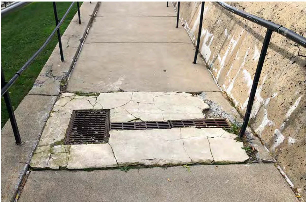
(top left and right) Figures 3-33 and 3-34: Ramp segments showing the spalling and delamination of walkway
