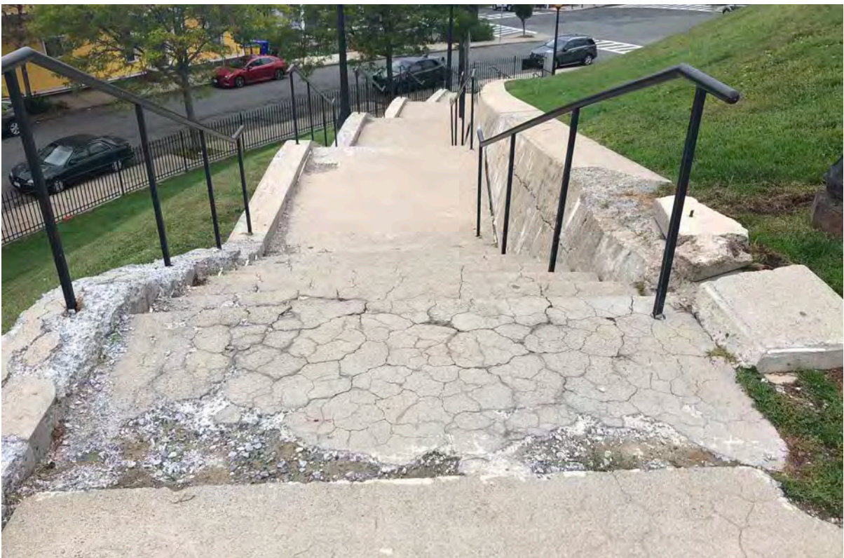
(top and bottom) Figures 3-38 and 3-39: Sample conditions of retaining walls and landings
