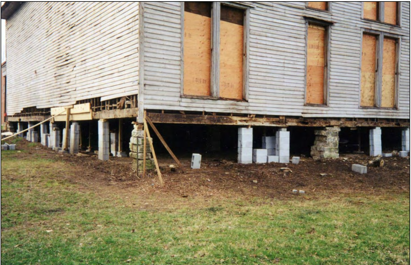
Figure 11: Renovation of the Sutton Store in 2000, View of the north elevation and the repair of the stone foundation using concrete blocks. Photo courtesy of Historic Granville, Inc.
