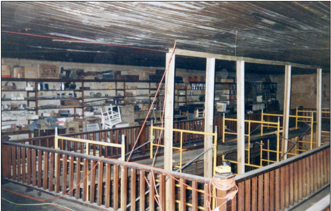
Figure 8: Renovation of the Sutton Store in 2000, View of the Main Sales Room from the Second Floor Balcony. Photo courtesy of Historic Granville, Inc.
