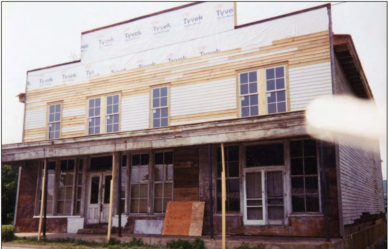
Figure 10: Renovation of the Sutton Store in 2000, View of the façade. Photo courtesy of Historic Granville, Inc.
