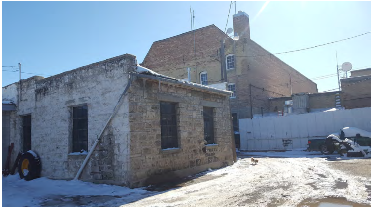
City Shop and Storage Garage, view to the south, north and west elevations.
