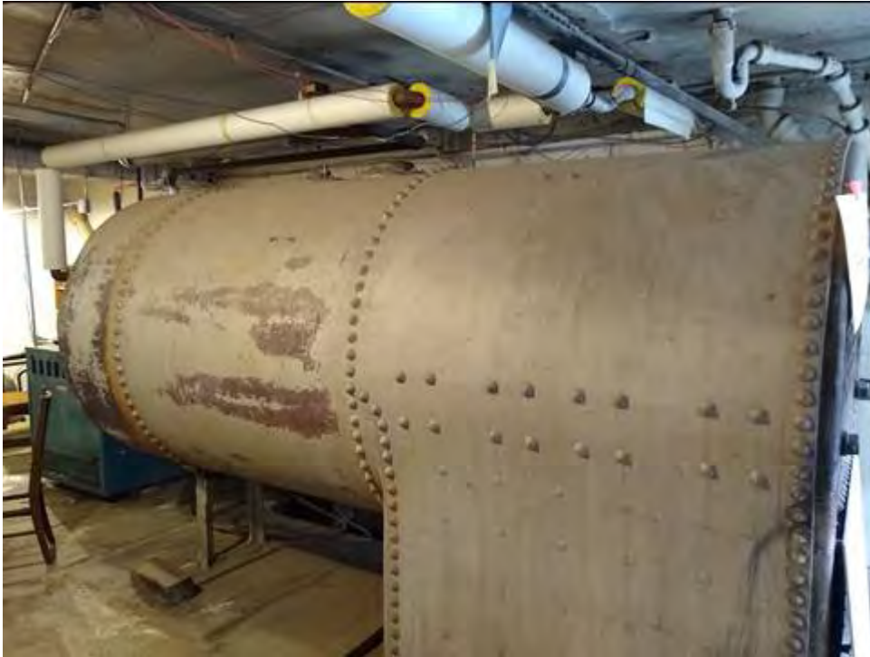
Dillon City Hall, boiler
