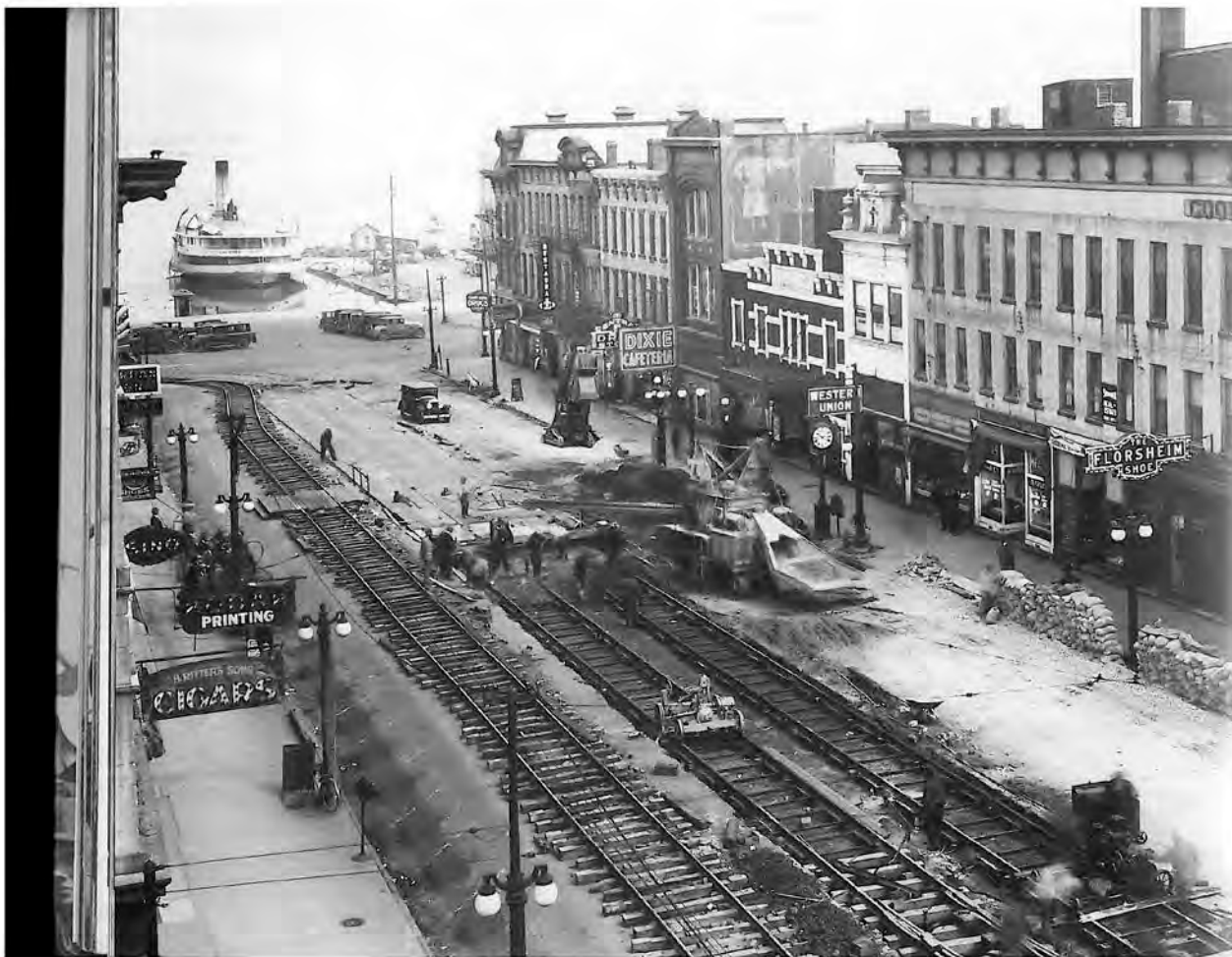
Figure 5: Laying streetcar tracks on Columbus Avenue - April 24, 1929 Image courtesy of Face of Firelands publication
