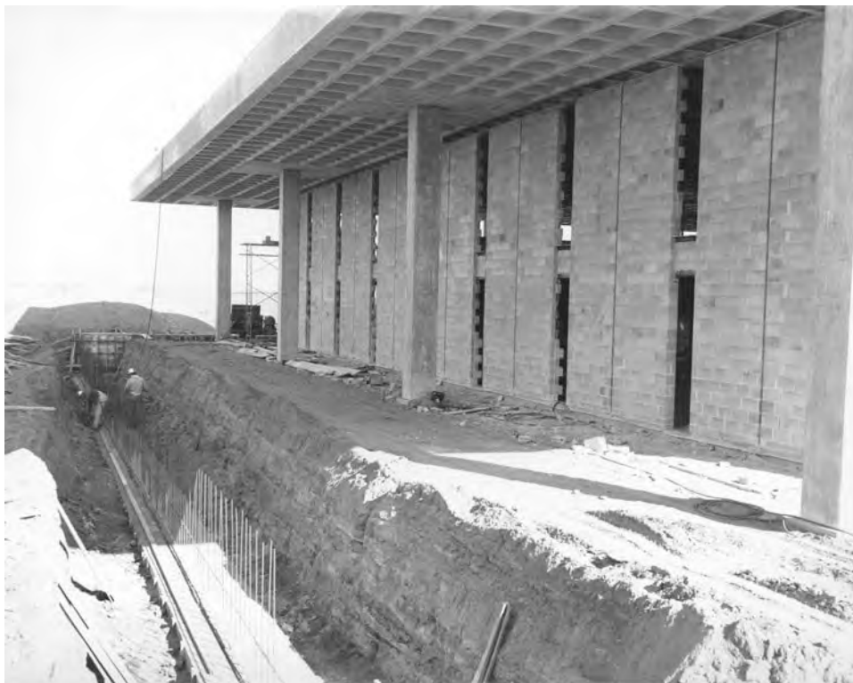
Figure 4: Construction photograph showing CMU wall construction and preparation of museum plinth. (Stuhr Museum of the Prairie Pioneer)
