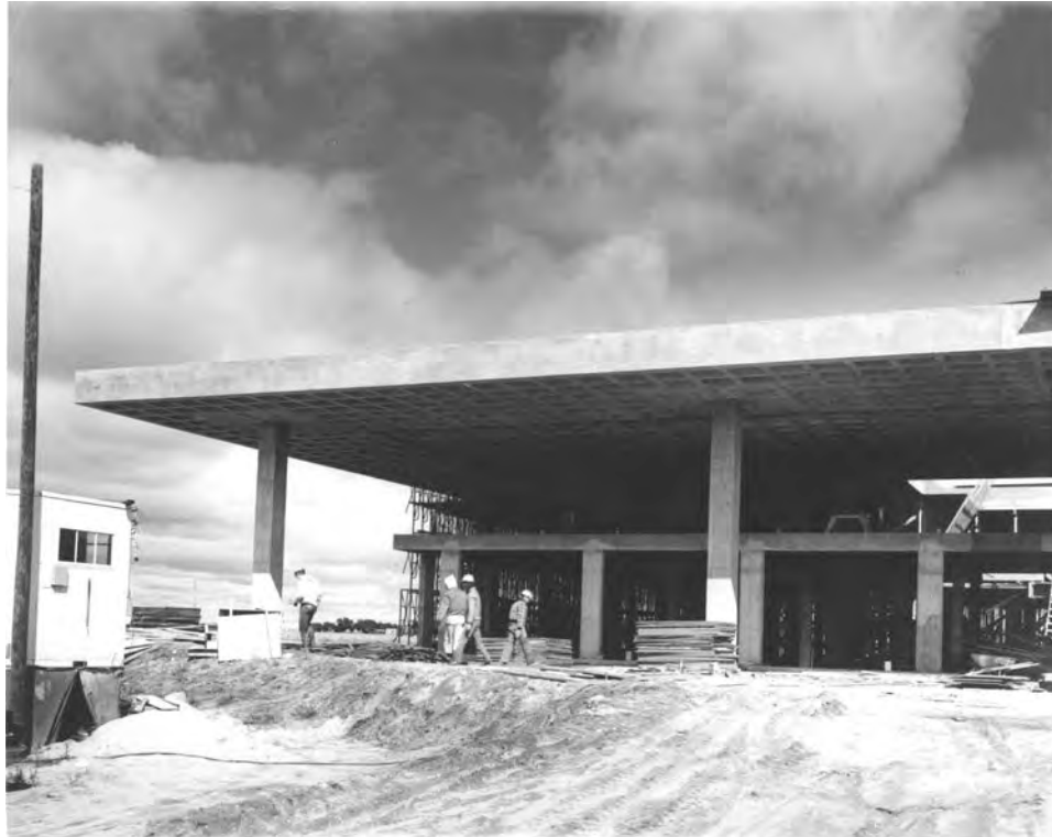
Figure 3: Stuhr Museum construction, 1967. Visible is the waffle slab roof and concrete structure. (Stuhr Museum of the Prairie Pioneer)
