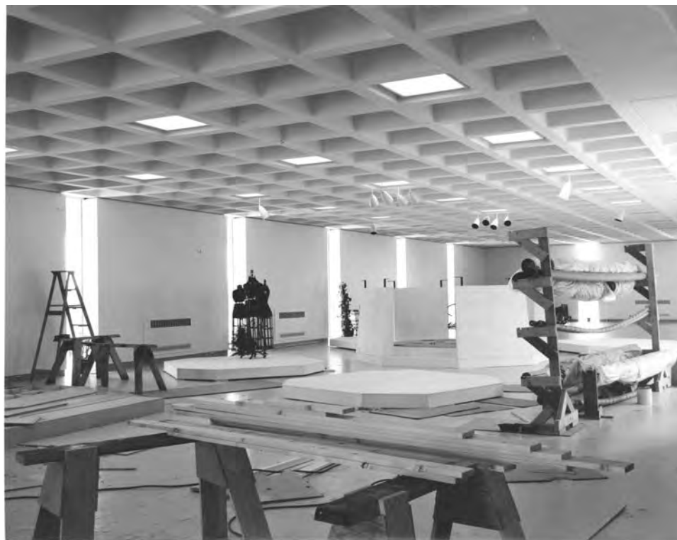
Figure 7: Second floor gallery space under construction. (Stuhr Museum of the Prairie Pioneer)
