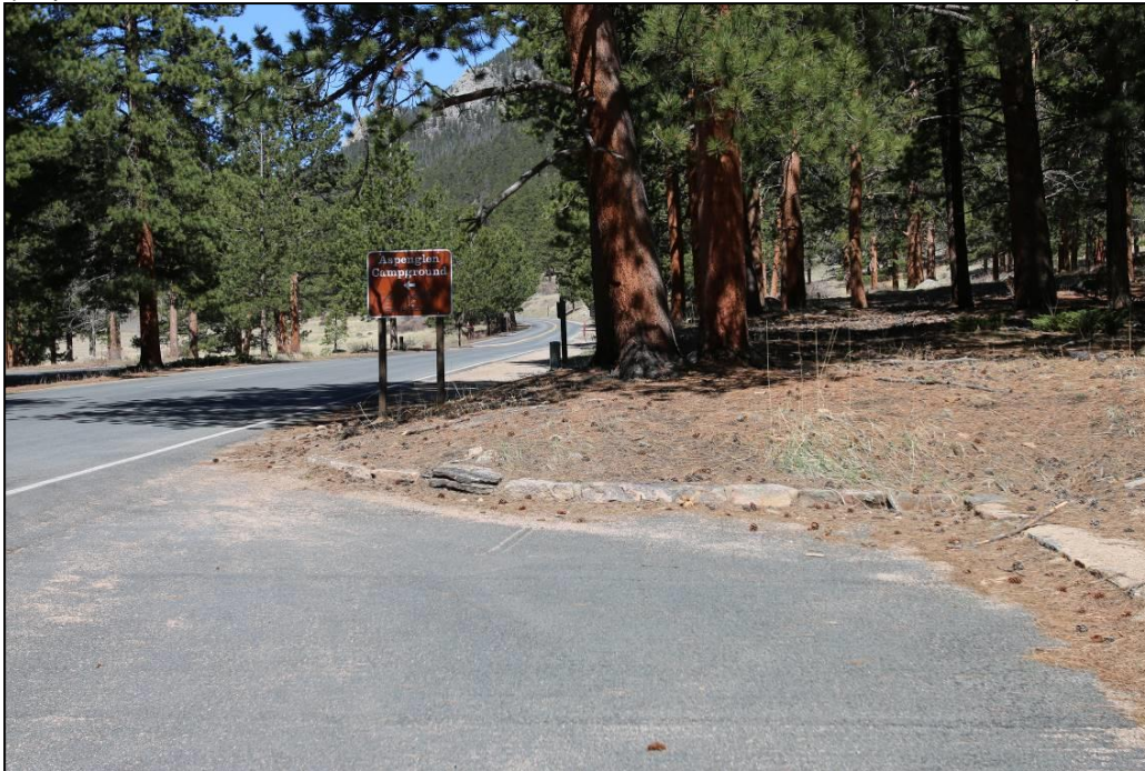
Photograph 11. Representative section of the masonry curbing at the 1933-1934 parking area at the site for the former checking station (Building 20), facing northwest.
