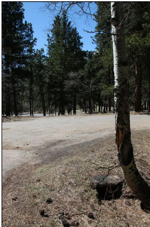
Photograph 24. View of the drainage culvert near the garage and woodshed (Building 169), facing southwest.
