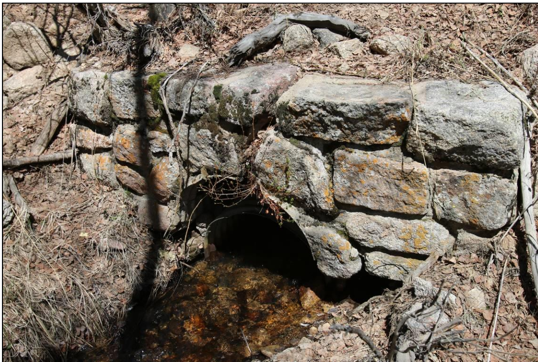
Photograph 25. View of the pipe culvert with stone headwalls on Bighorn Creek, facing south.
