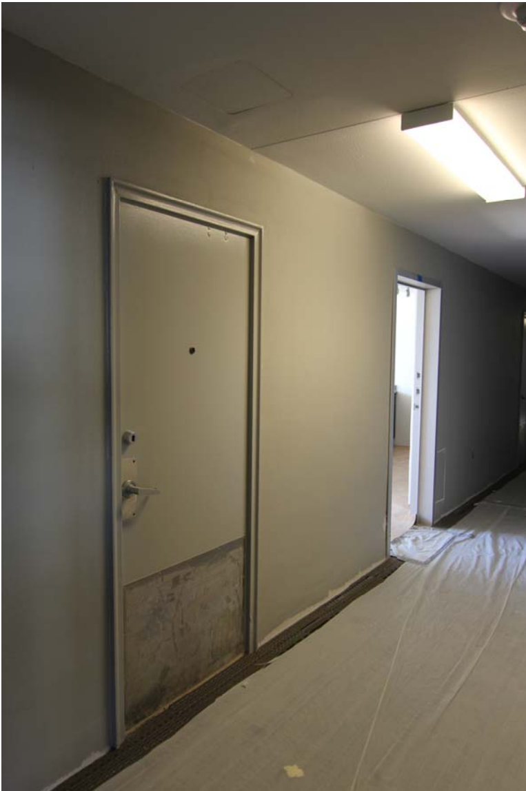
Photo 9 - View of a historic door opening with original metal door frame, fixed newer (c. 1973) door and hardware. Camera facing Northwest.
