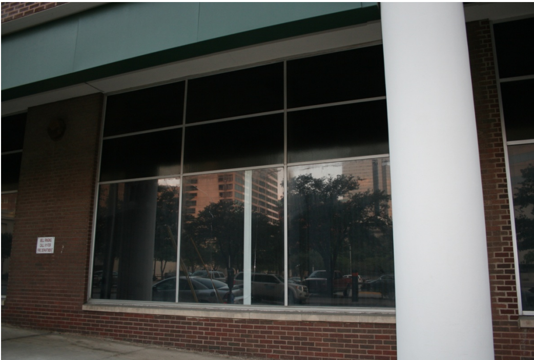
Detail of aluminum storefront at Burnett Street; Camera facing West. Much of the original aluminum storefront remains in place. Green signband dates from 1973 alterations.
