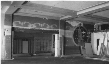
Figure 8 Current photo of the north wall (party wall), looking through an opening made between the former theater auditorium and the old City Hall next door in order to join the two spaces for a past retail use. Note the steel I-beam header installed between two interior pilasters. The decorative painted swirls may be inspired by the modernistic plaster waves appearing at the top of the pilasters just below the ceiling. Note also the wall mural to the right of the opening. Tallgrass Historians L.C. photograph, 2007.
