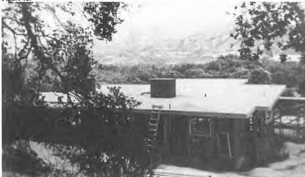
Photograph of house under construction, view facing northwest, 1949, courtesy of Theodore Thomas, Jr.
