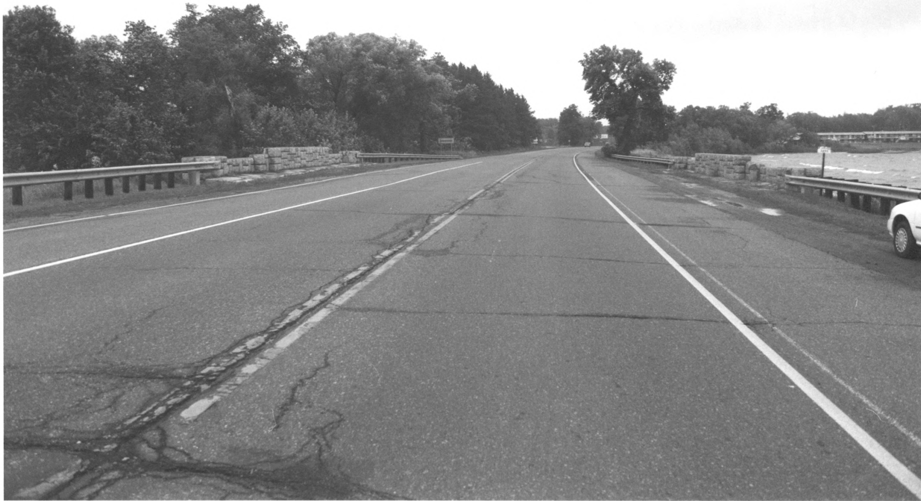
Bridge no. 3355 U.S. Highway 169 over Whitefish Creek, Kathio Township Mille Lacs Co., Mn 013081-19A/20
