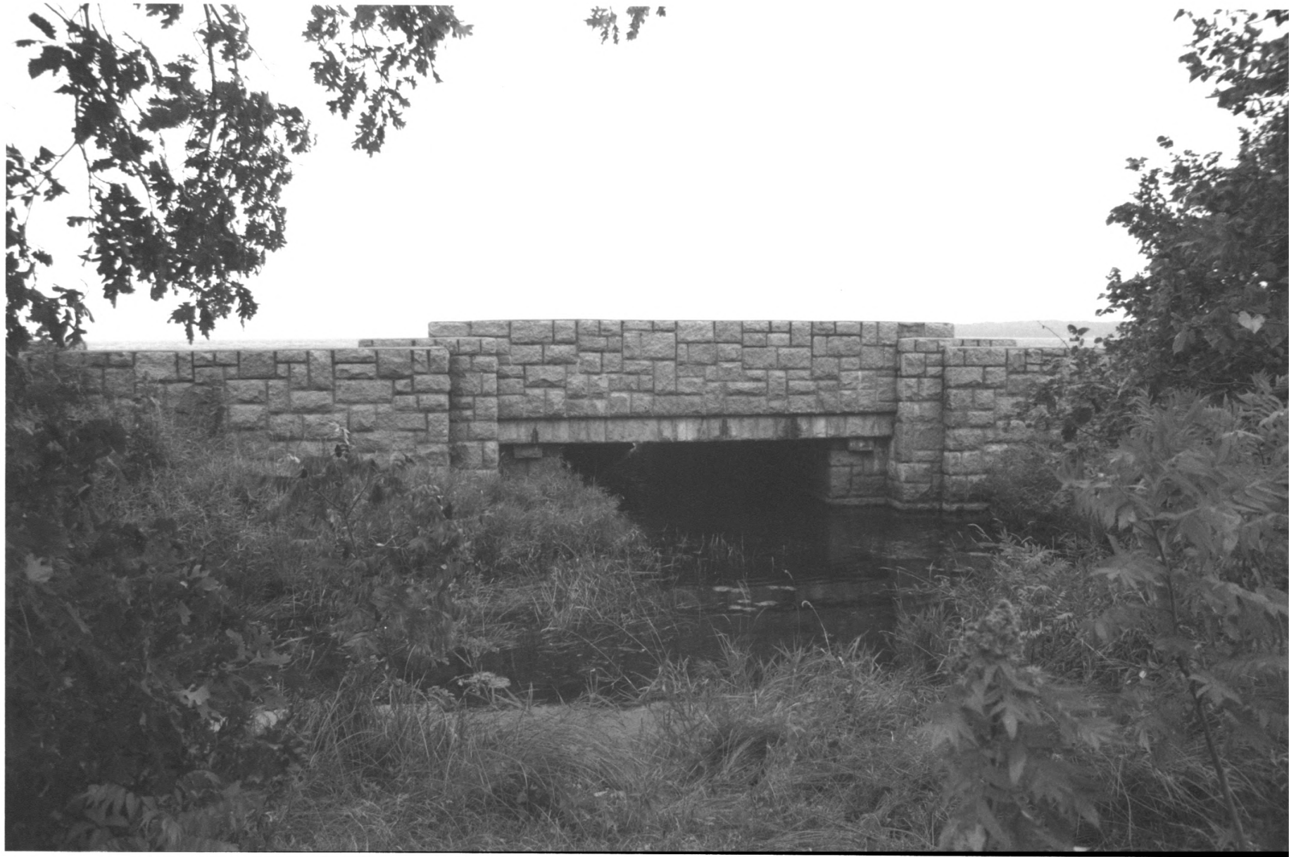
Bridge no. 3355 U.S. Highway 169 over Whitefish Creek, Kathio Township Mille Lacs Co., Mn 013081-22A/23
