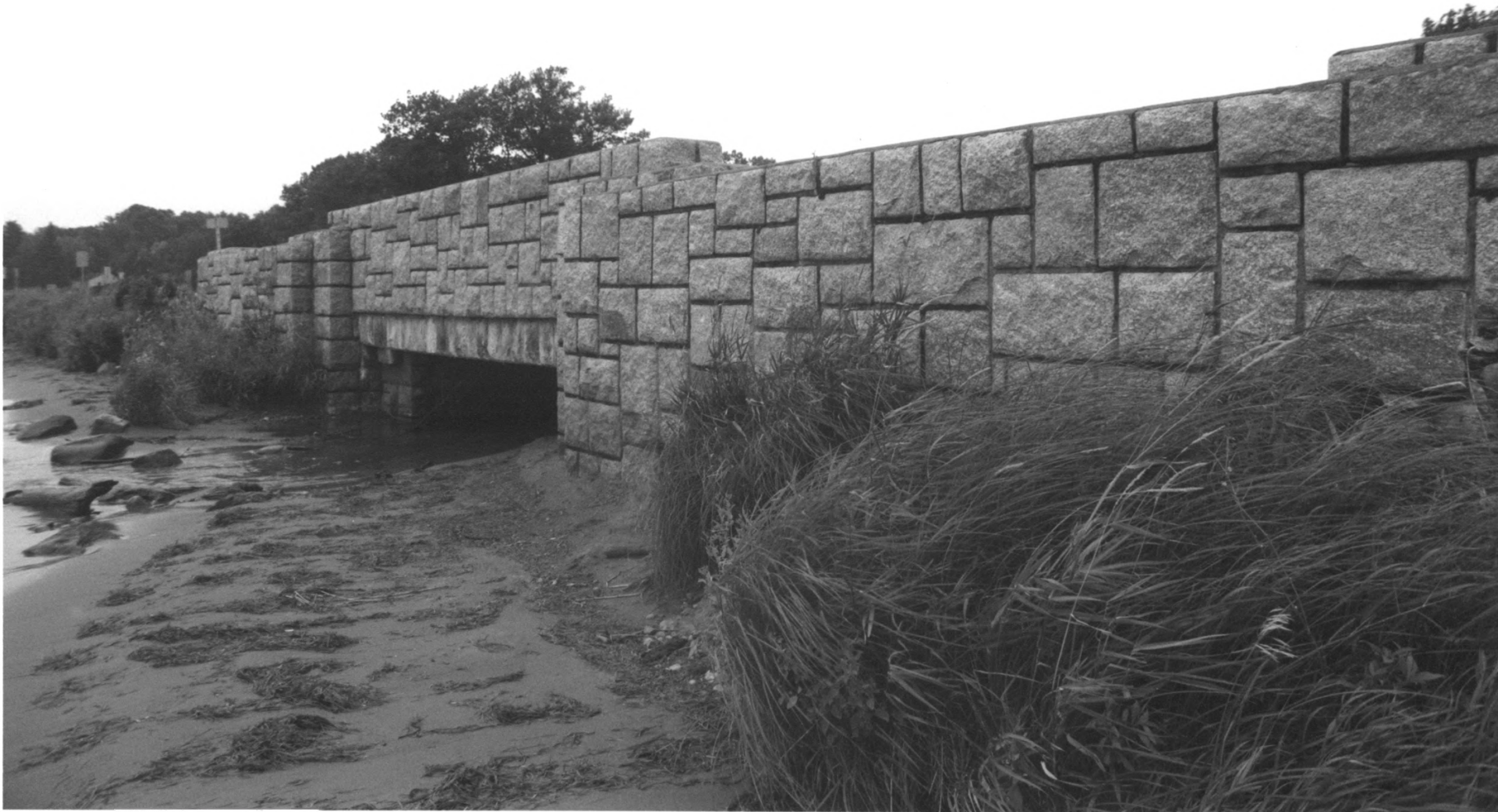
Bridge no. 3355 U.S. Highway 169 over Whitefish Creek, Kathio Township Mille Lacs Co., MN 013081-21A/22
