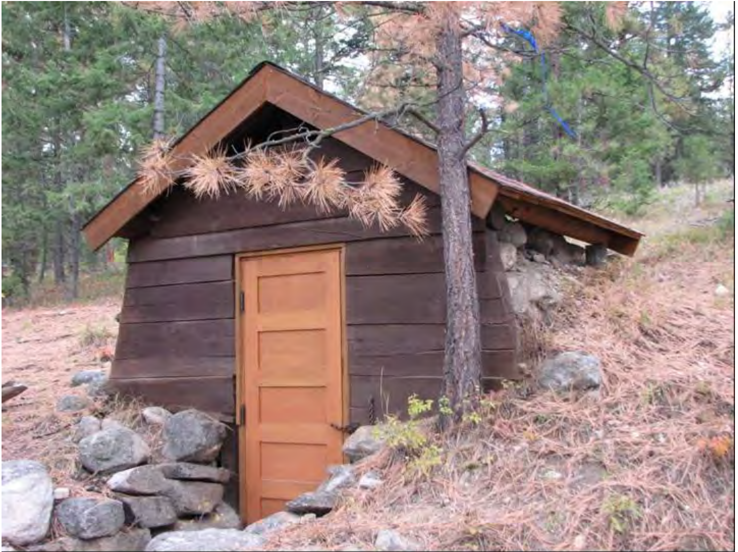
Photo 0010 Hayward Lodge ice house: looking northwest to the front (south) and east walls.
