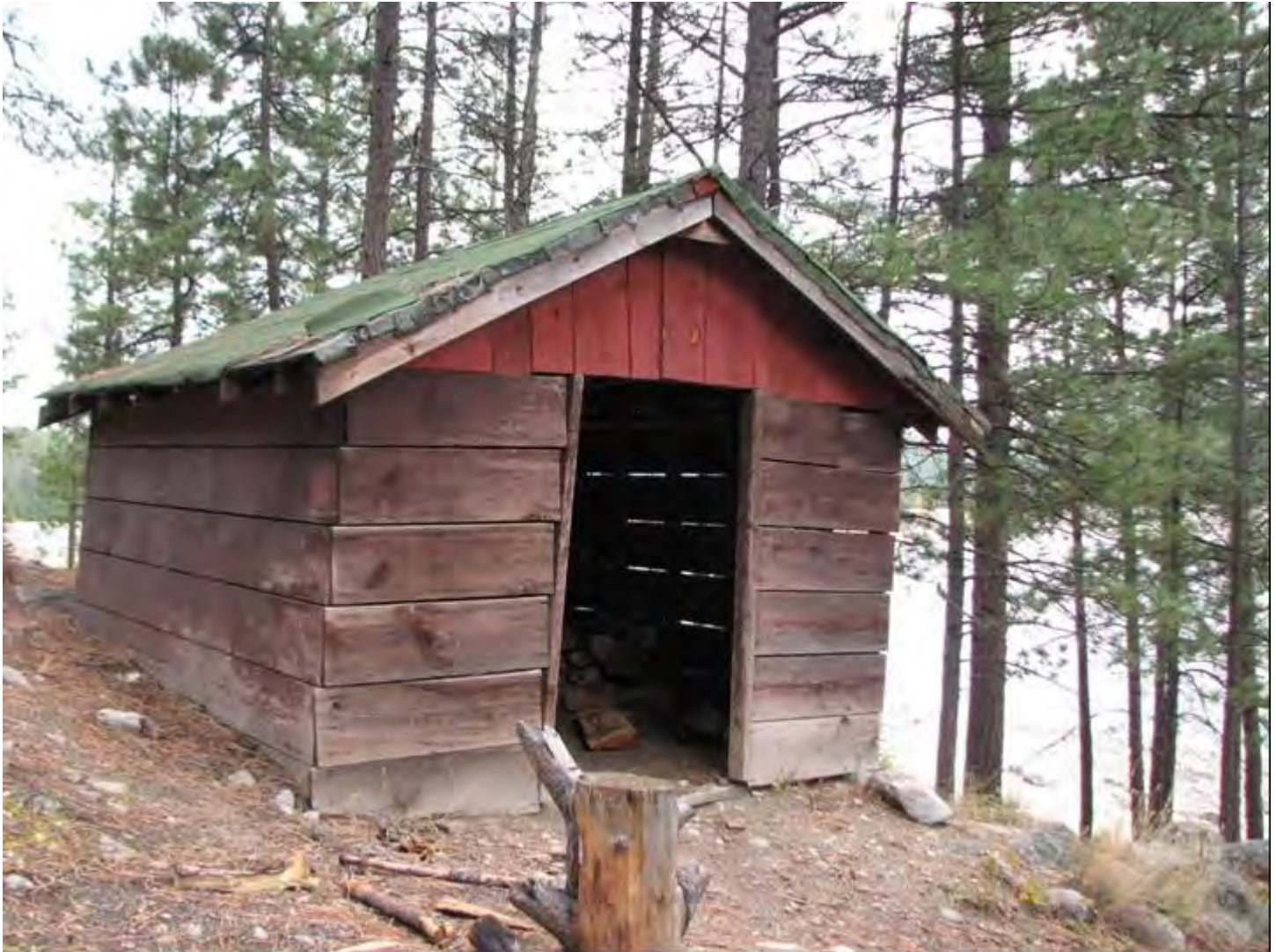
Photo 0014 Hayward Lodge wood shed: looking southeast to the front and side walls.
