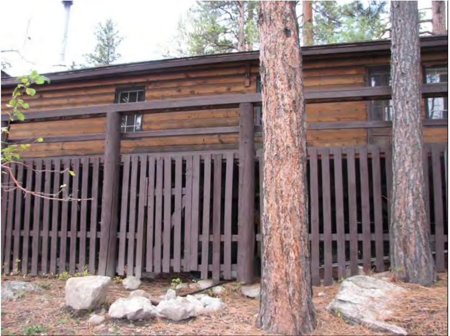
Photo 0004 Hayward Lodge: south wall of the east wing showing the enclosed area below the deck.
