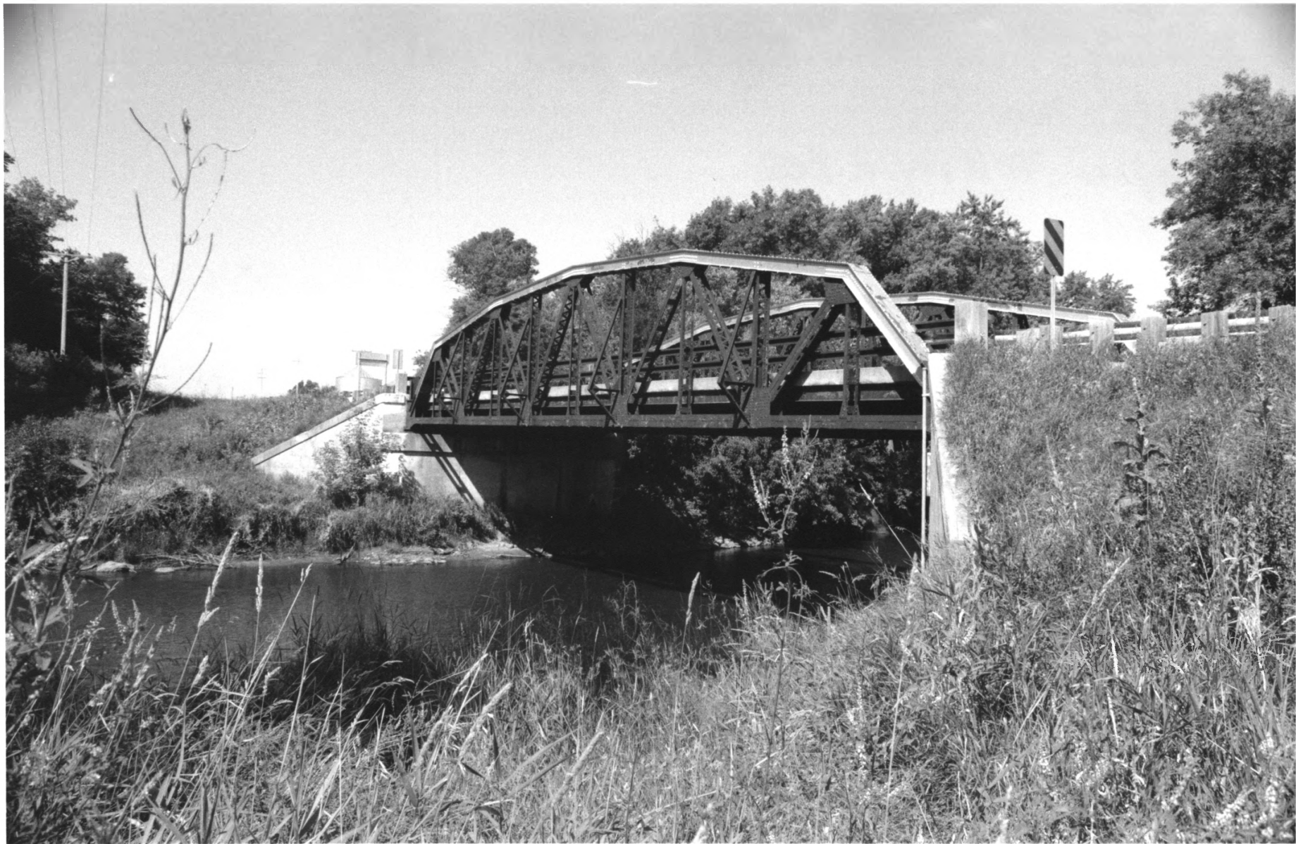
Bridge no. 5388 Mn Highway 24 over North Fork Crow River, Forest City Township Meeker Co., Mn 013059-6
