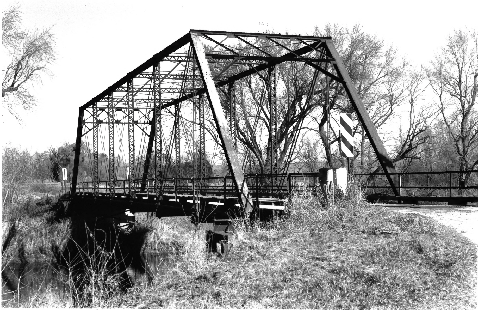
Bridge no. 40980 Co. Rd. 190 over the north fork of Crow River Meeker Co. 012208- 12A/13
