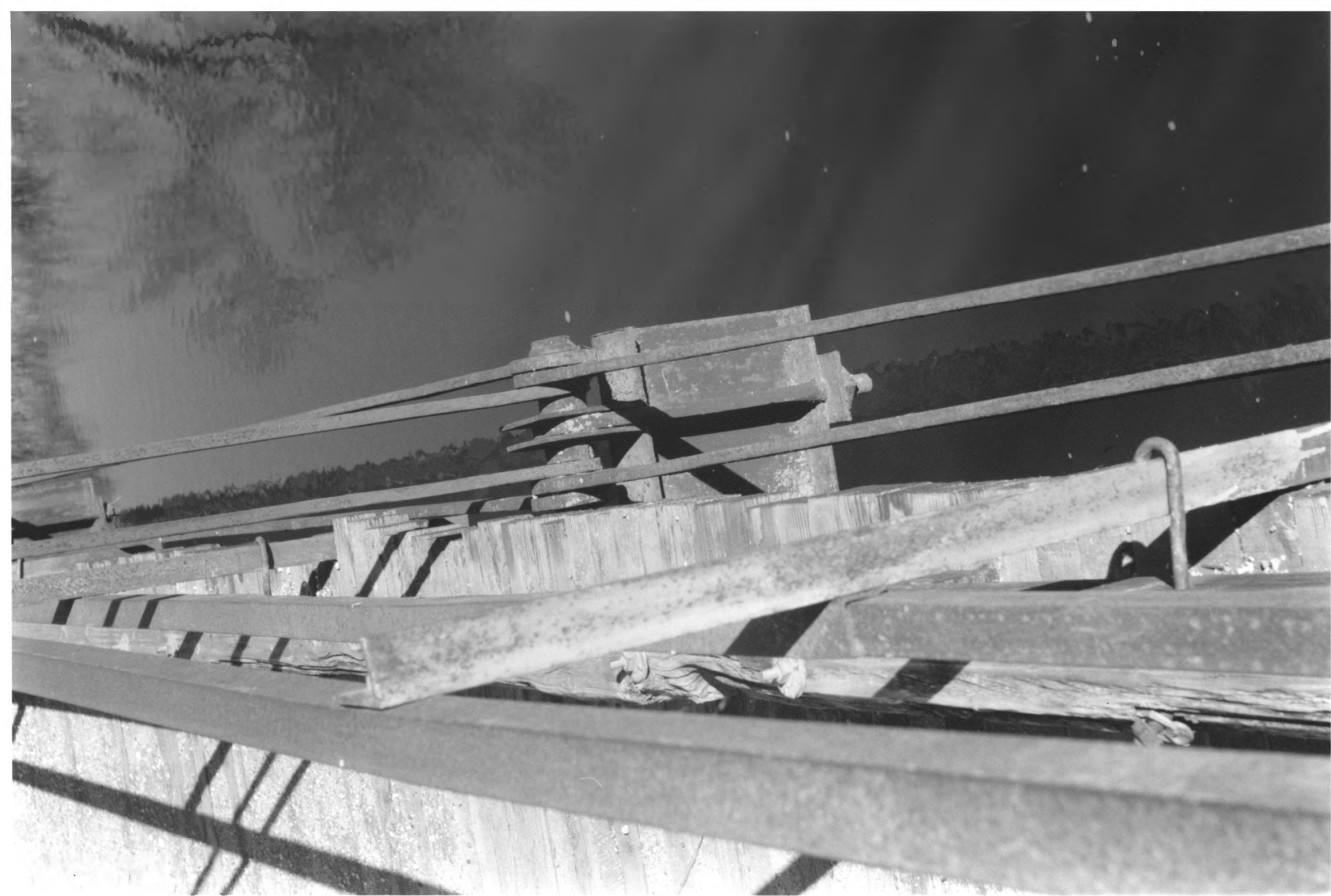
Bridge no. 90980 Co. Rd. 190 over The north fork of Crow River Meeker Co. 012208-1A/2
