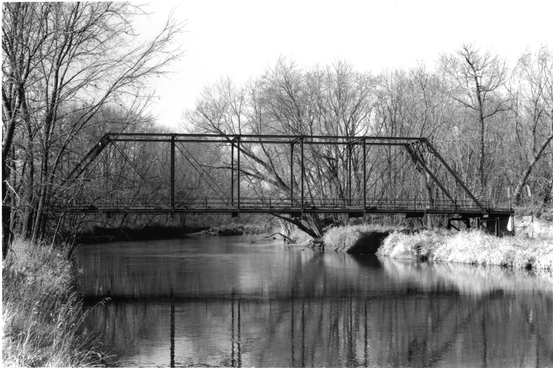
Bridge no. 90980 Co. Rd. 190 over The North fork of Crow River Meeker Co. 012208-14A/15
