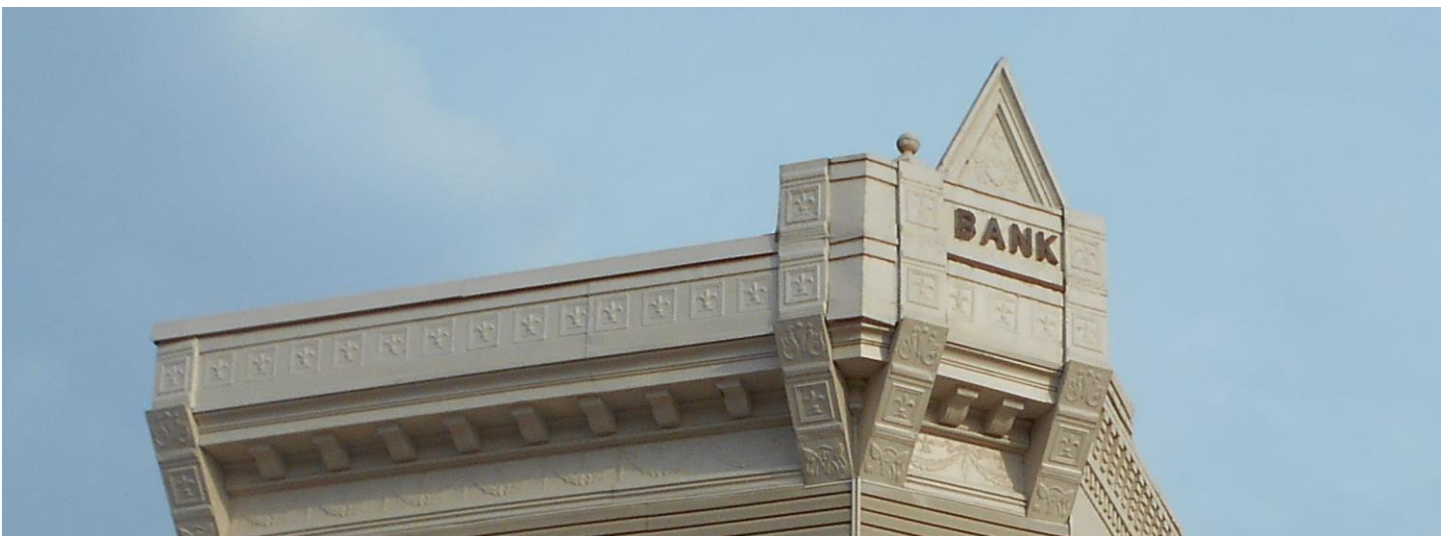
Figure 4 Farmers Savings Bank (101 4 th St. W.) has both metal and brick cornices. Tallgrass Historians LC, 2015
