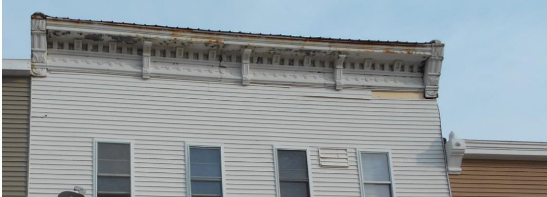
Figure 7 The turn-of-the-century Downer & Derby store building's ornate cornice (109 4 th St. W.) is pressed metal that is showing some rust. Tallgrass Historians LC, 2015
