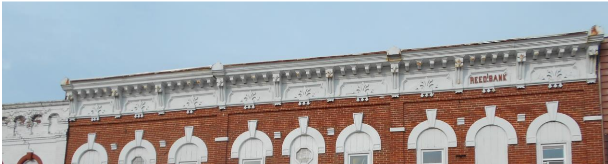
Figure 8 The south three bays of the Reed Building(313-315-317 Cedar St.) also have pressed metal cornices . Tallgrass Historians LC, 2015
