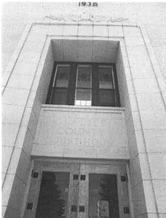
MT_GlacierCounty_GlacierCountyCourthouse_002 Glacier County Courthouse, detail of north elevation main entry, view to south.
