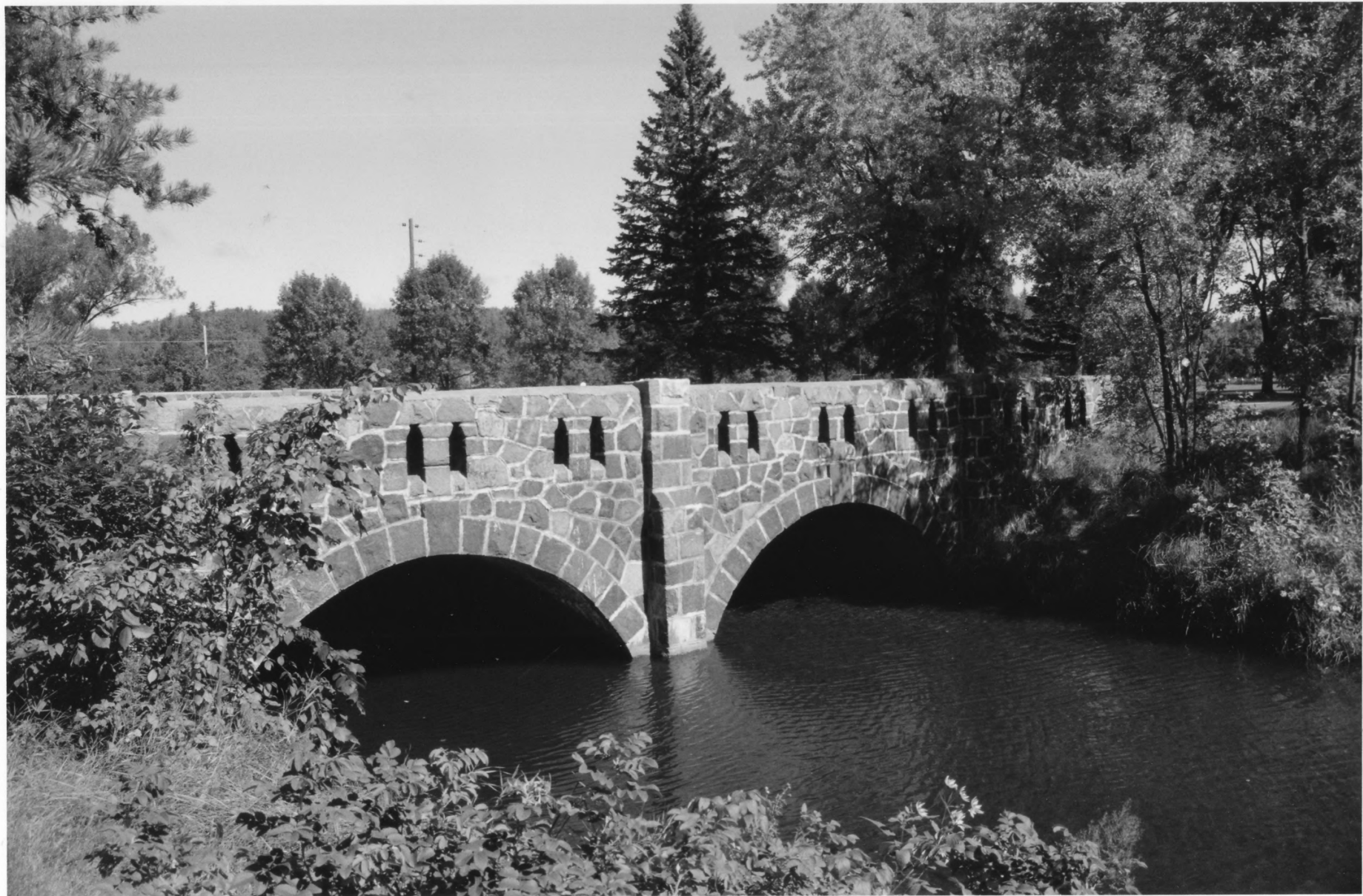
Bridge no. 5757 Mn. Hwy. 23 over Mission Creek, Duluth St. Louis Co., Mn 013072-10
