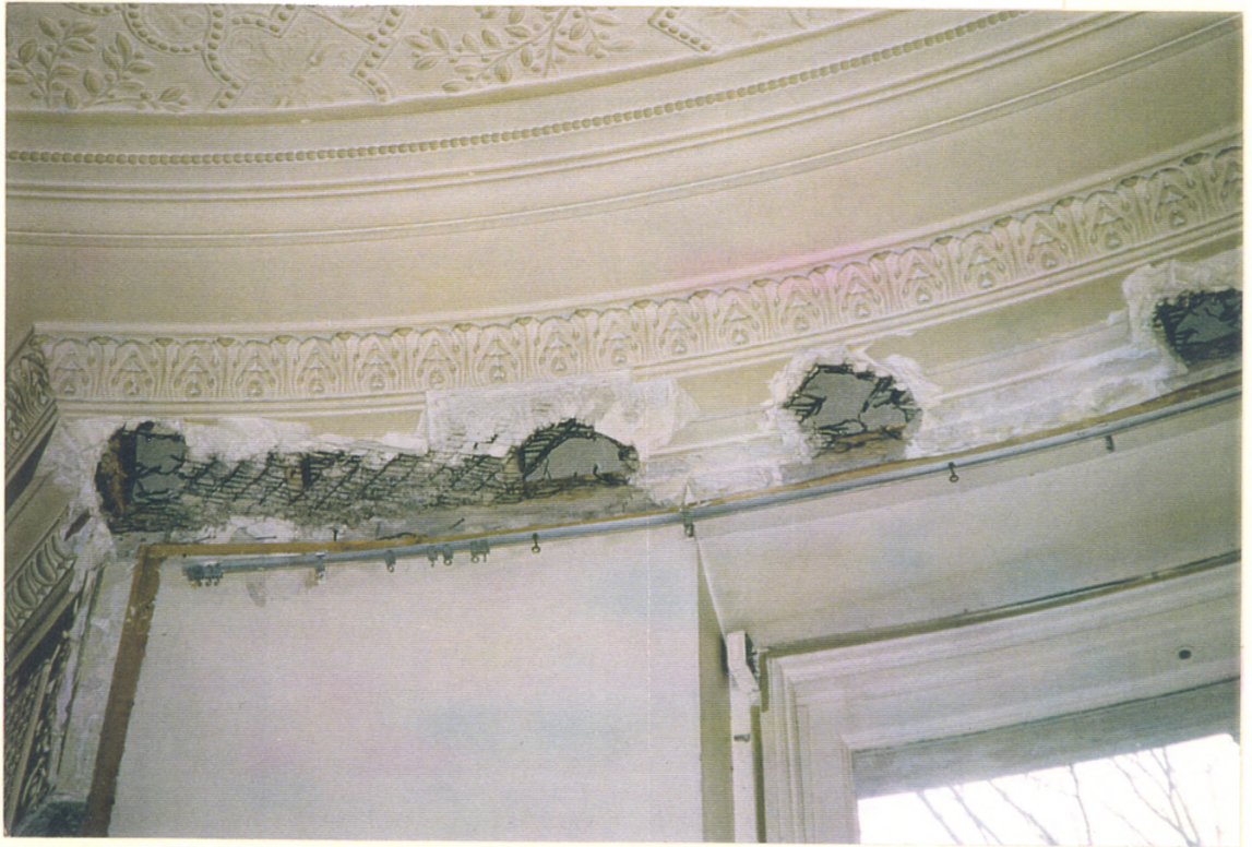
BAYRIDGE RESIDENCE First Floor Drawing Room Crown Molding (Damaged by False Ceiling Placed by Previous Owners)
