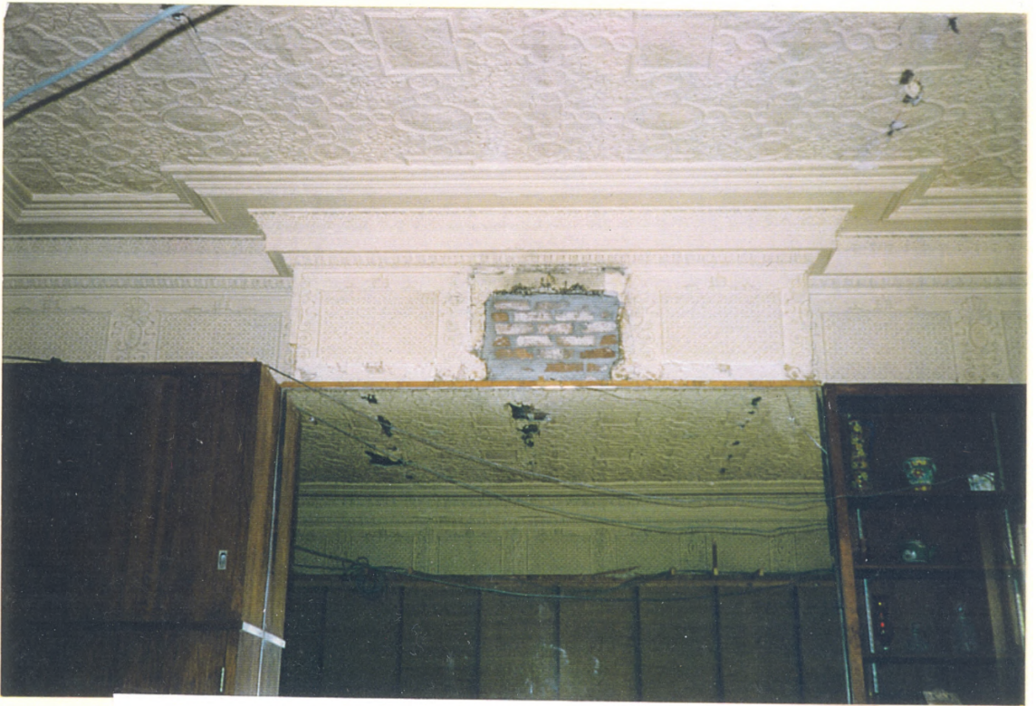
BAYRIDGE RESIDENCE First Floor Drawing Room (Closets & Mirror Installed by Previous Owners)
