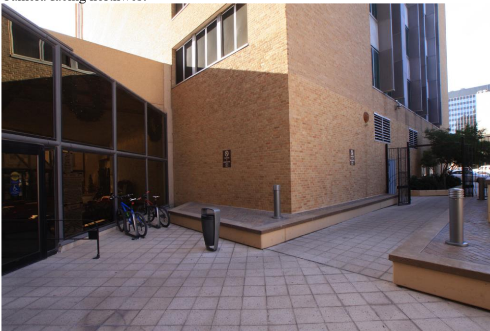
Photo 13 Ground floor at southeast corner (connection to hyphen on left) Camera facing northwest
