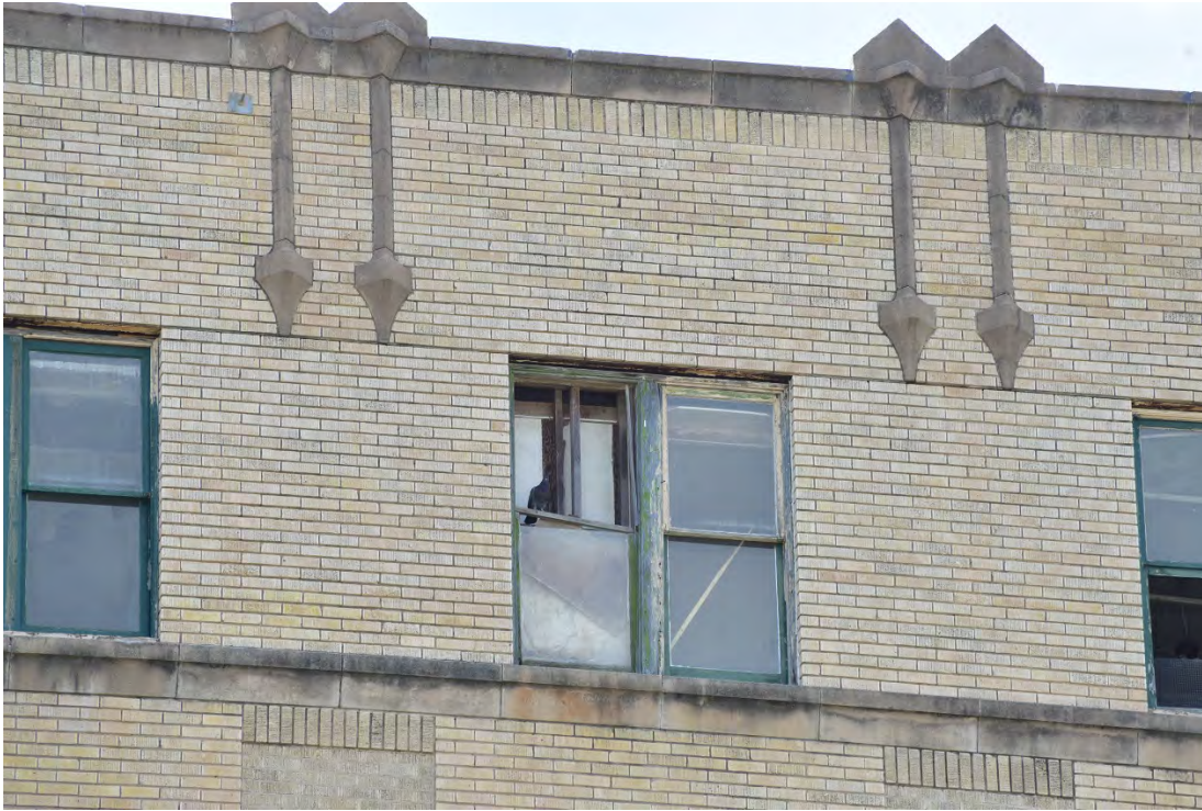
Photo 5. East elevation, detail of masonry at ninth floor column capitals and parapet ornament, view west.
