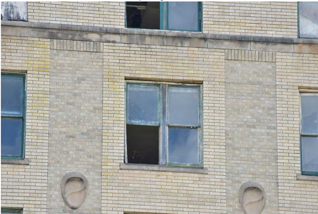
Photo 6. East elevation, detail of masonry at eighth floor, columns and cartouches, view west.
