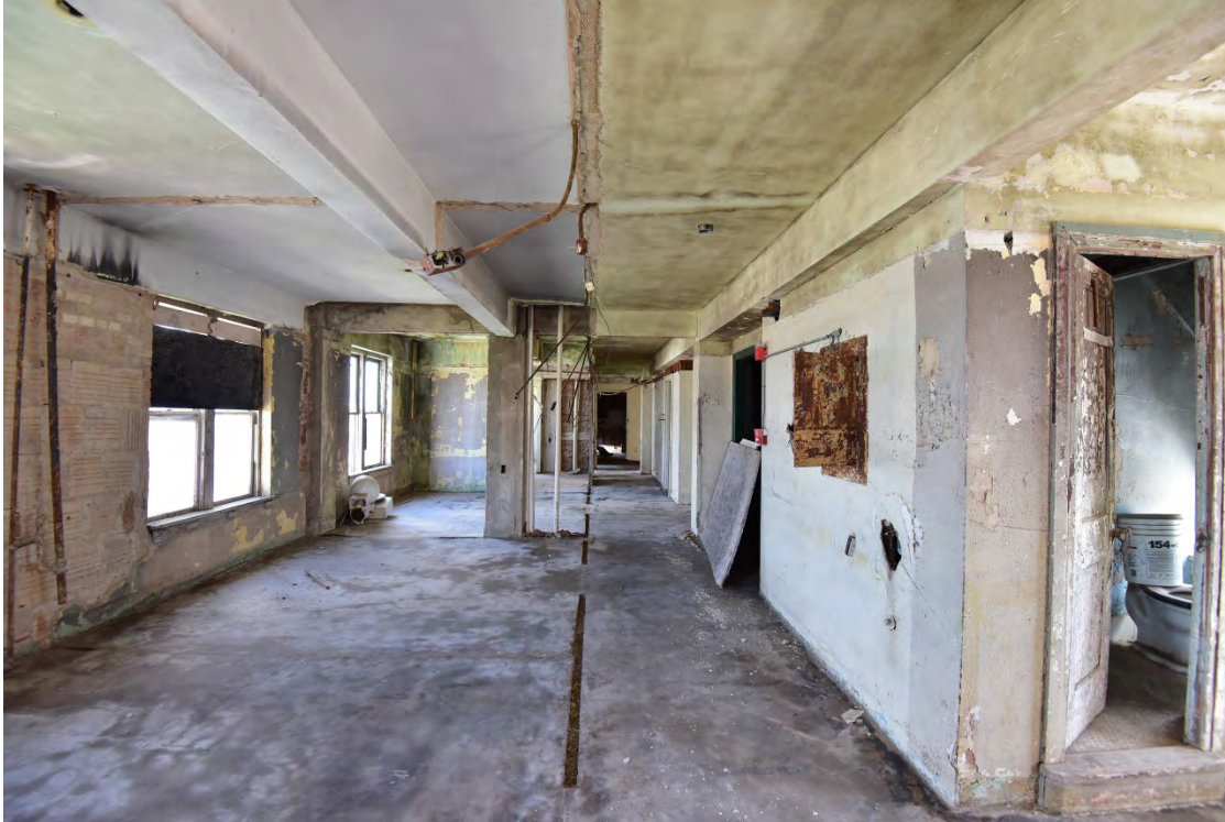
Photo 15 Seventh Floor, view south. This floor shows historic partitions (right) and layout alterations (left).
