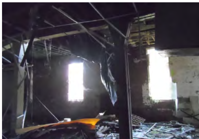
Partially collapsed East Addition
