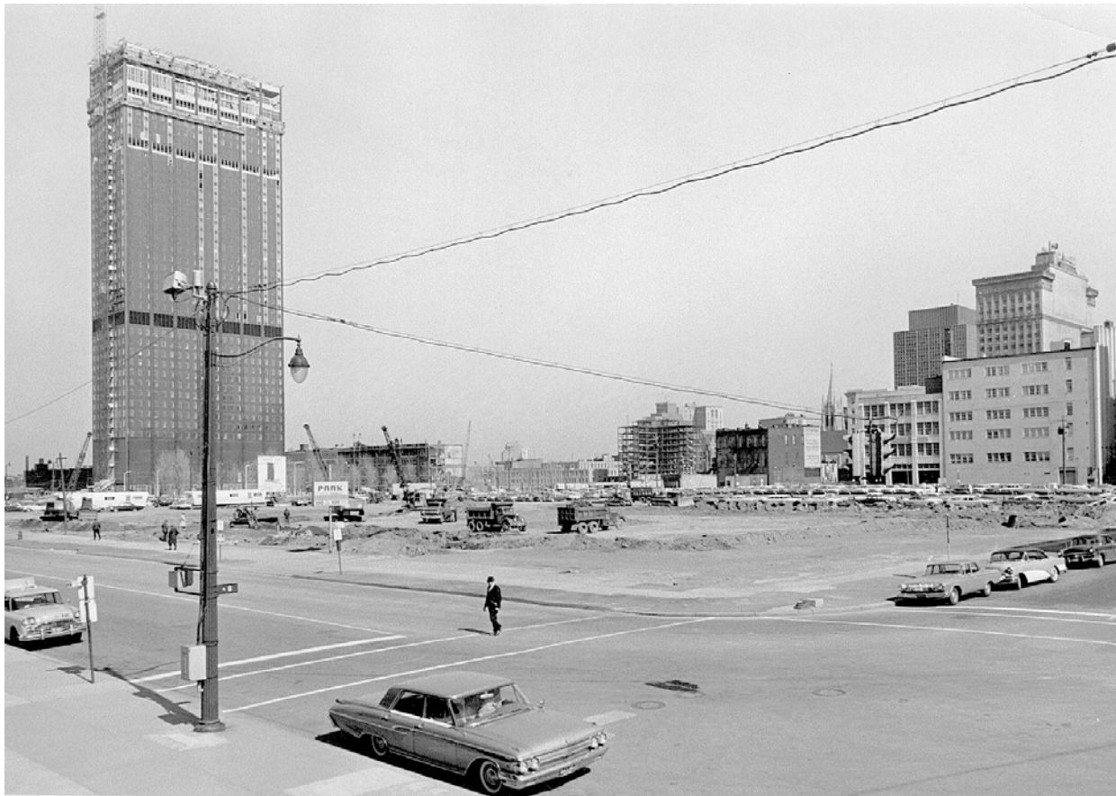
FIGURE 14 – Erievue Tower construction with existing buildings in background, April 24, 1964, view looking southeast; Photo A27903, Cleveland Public Library Photograph Collection.
