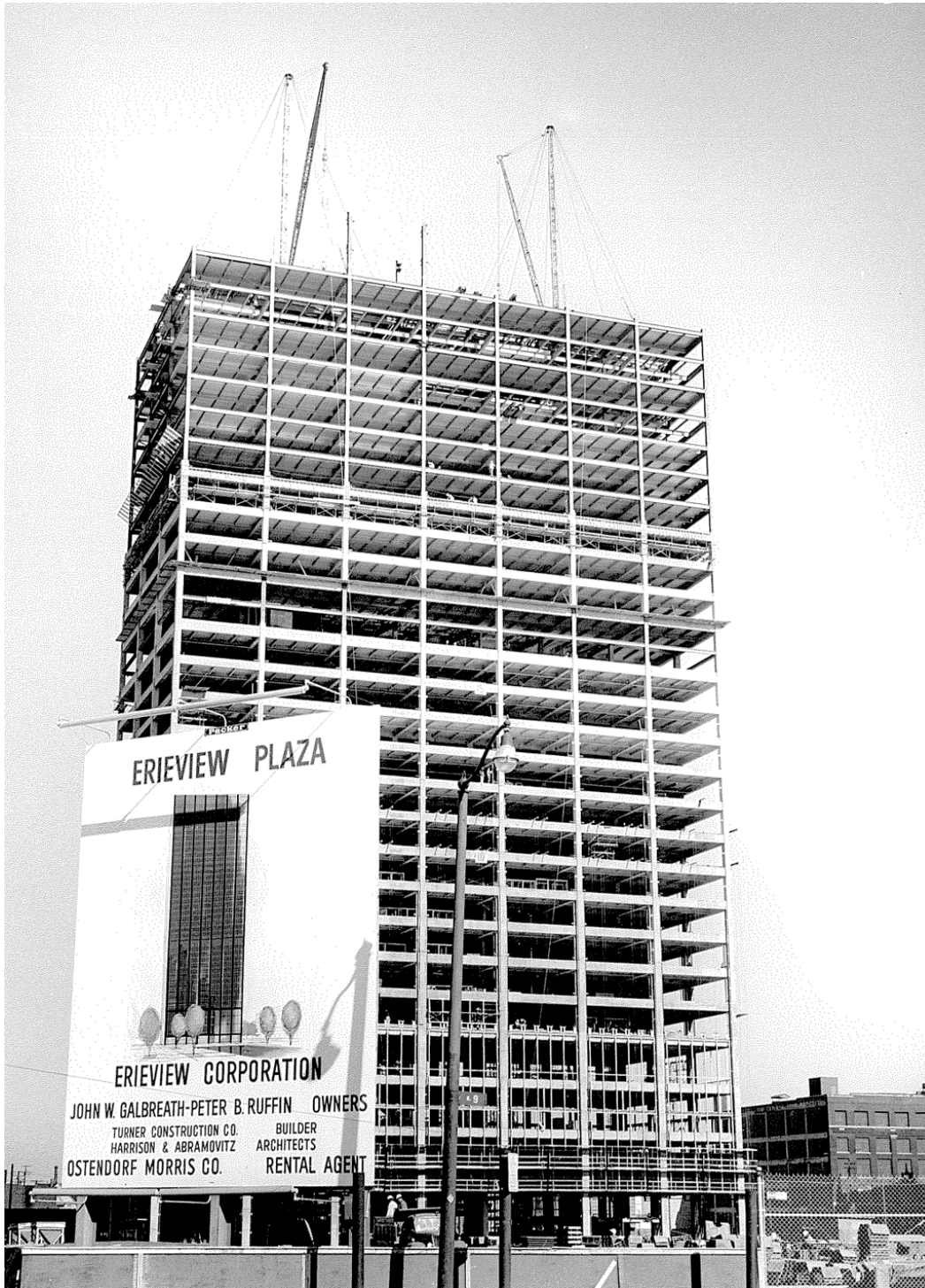
FIGURE 12 – Erievew Tower construction with project sign, October 16, 1963, view looking east; Photo 288-3, Cleveland Public Library Photograph Collection.
