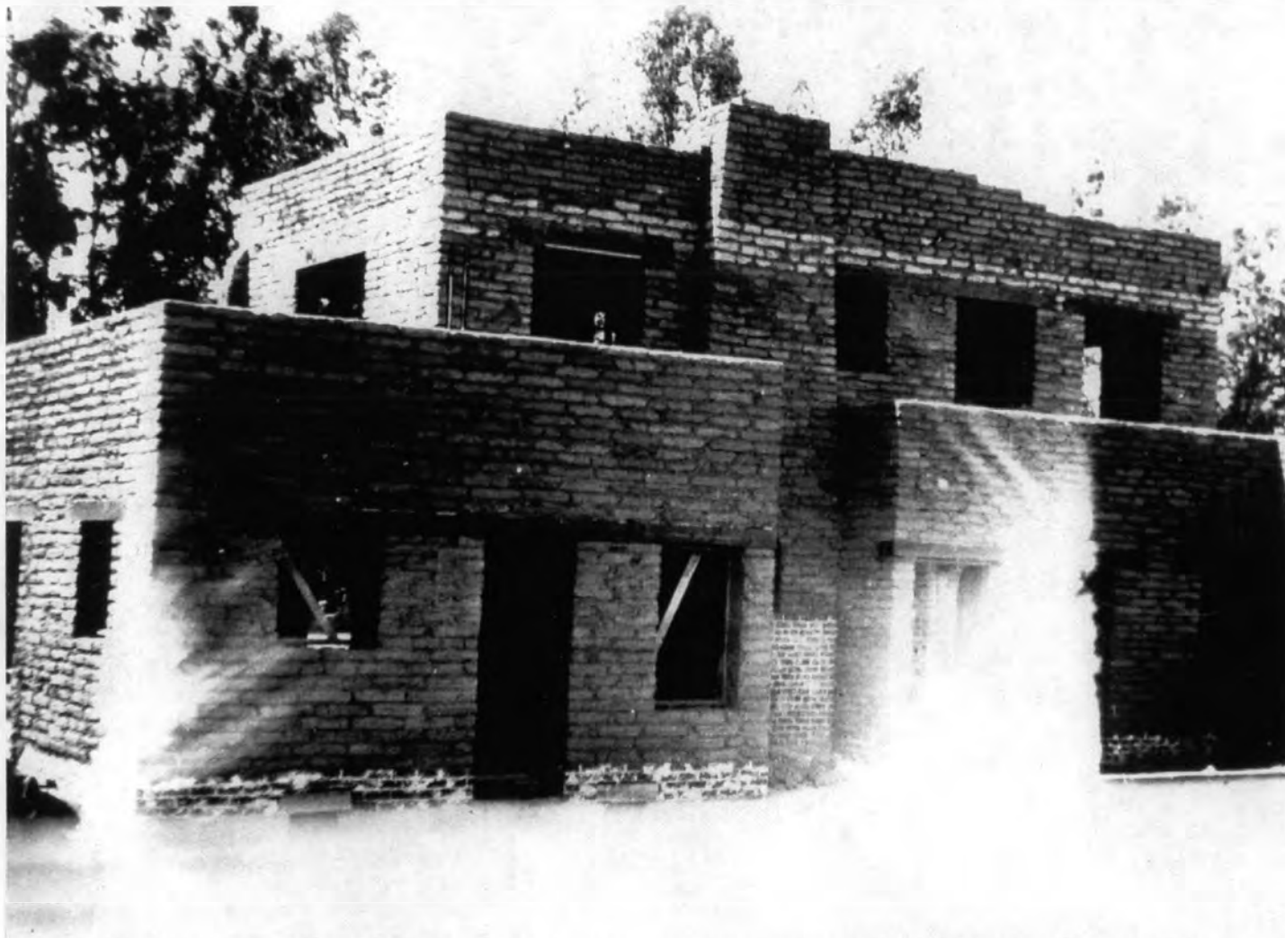
Figure 2. Louis J. and Gertrude Lee Bohn House, rear facade under construction, ca. 1929. Courtesy of the City of Phoenix Historic Preservation Office.
