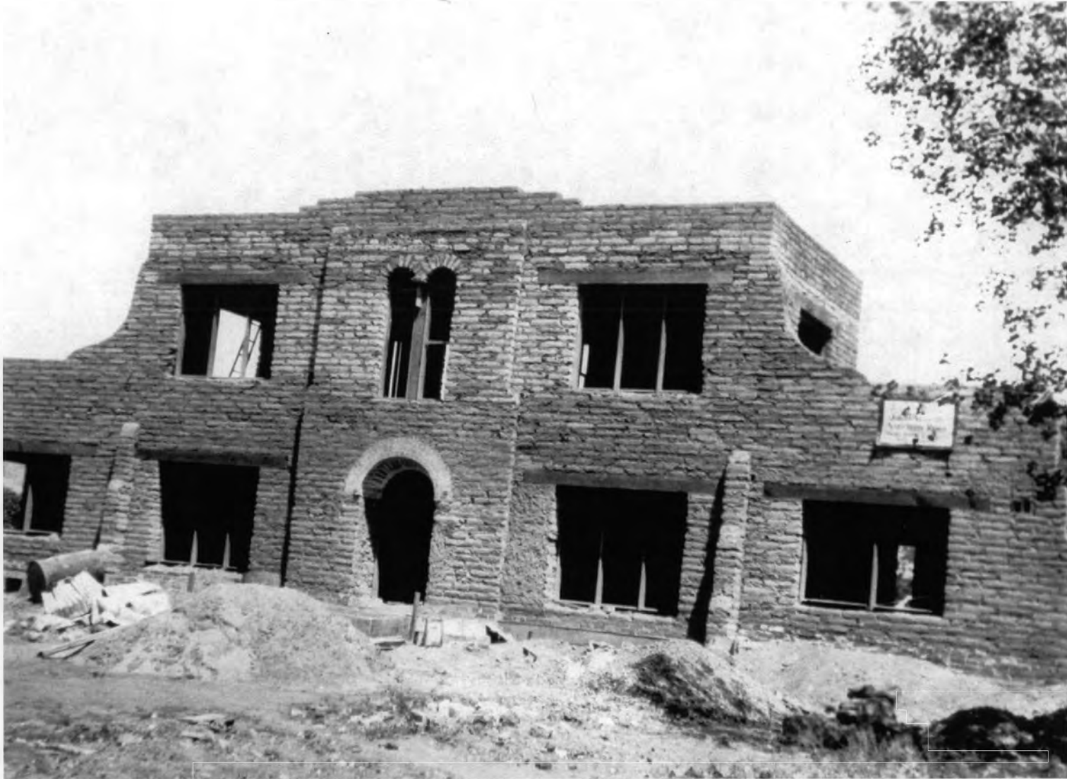
Figure 1. Louis J. and Gertrude Lee Bohn House, front facade under construction, ca. 1929. Courtesy of the City of Phoenix Historic Preservation Office.
