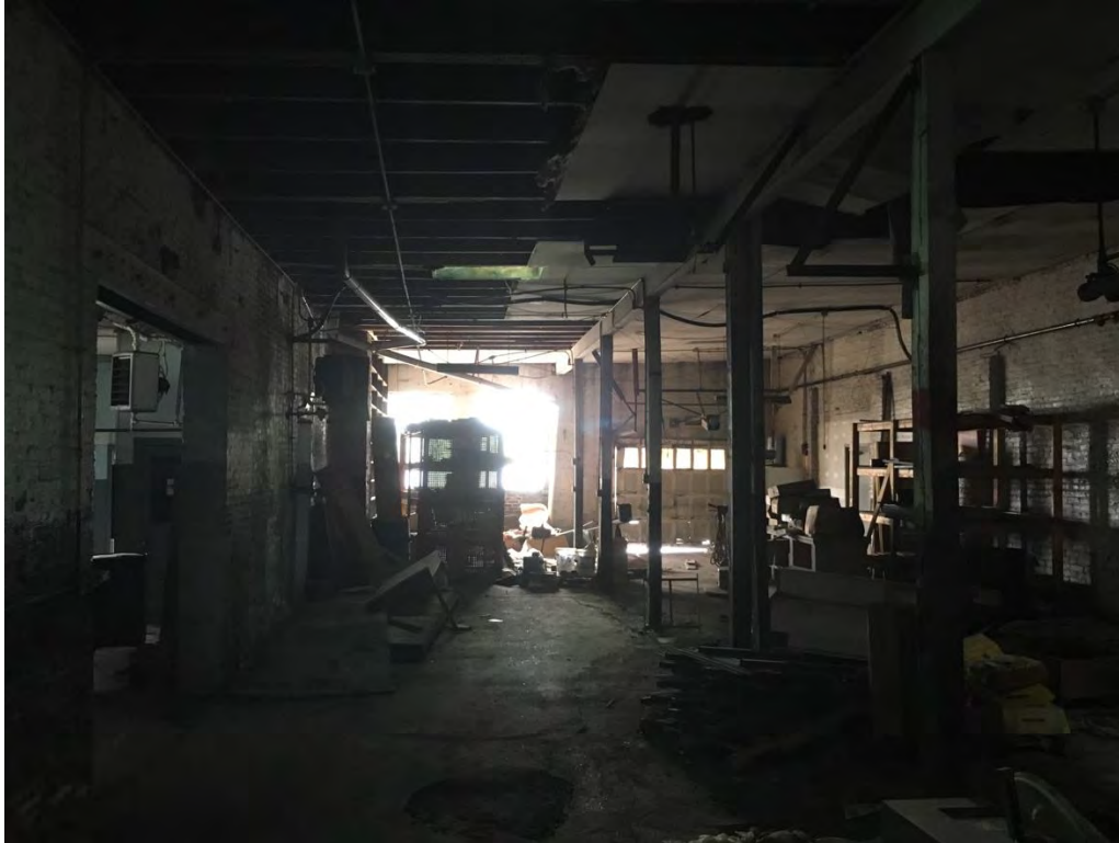
4 of 19: Warehouse space on the first floor, facing north, in the east portion of the building.
