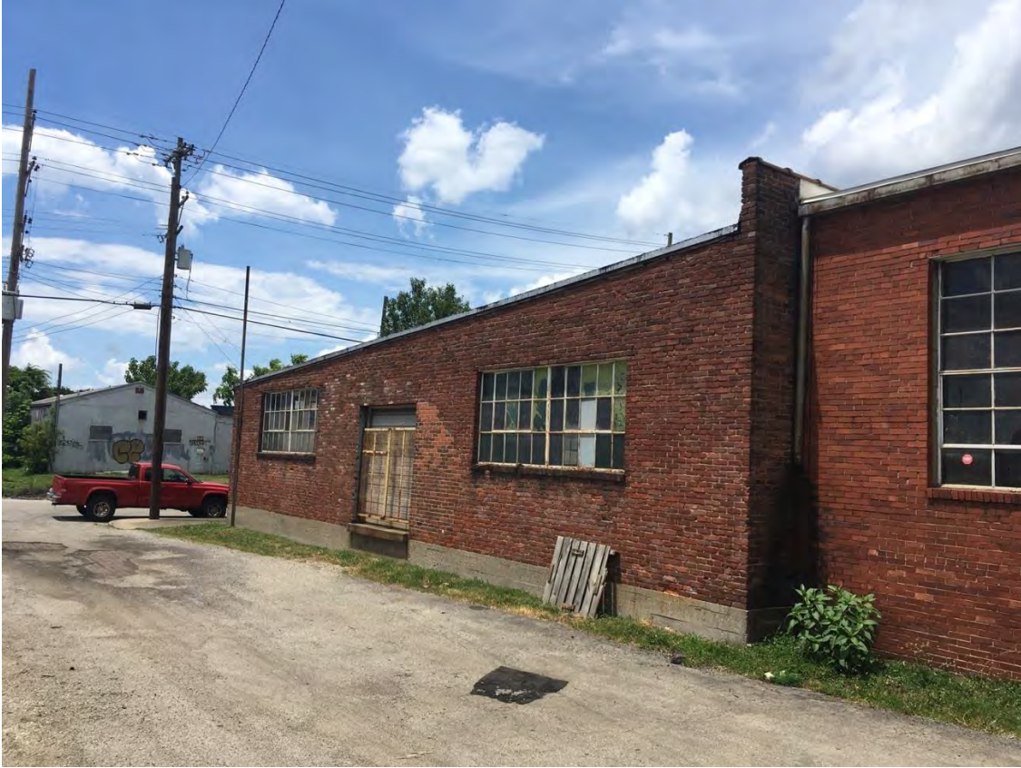
The rear façade, as seen from the alley behind the buildings, facing west toward 13 th Street.
