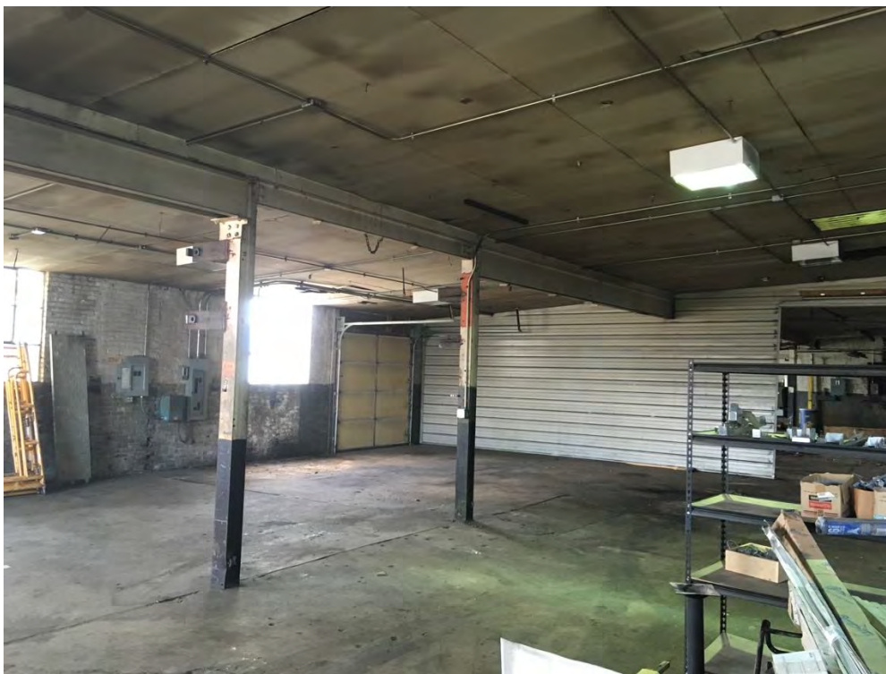
15 of 19: The rear storage space, facing northwest from near the back corner.
