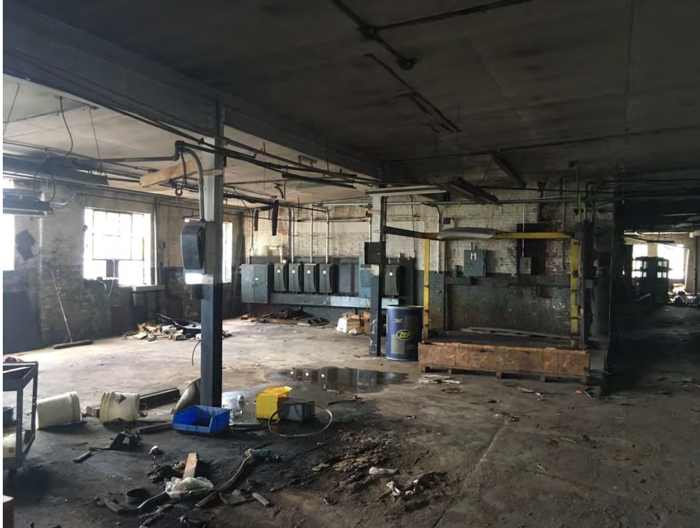
6 of 19: Warehouse space at the mid-point of the first floor, facing north.
