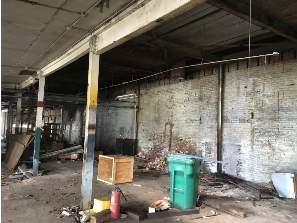
8 of 19: Warehouse space at the mid-point of the first floor, facing northeast.
