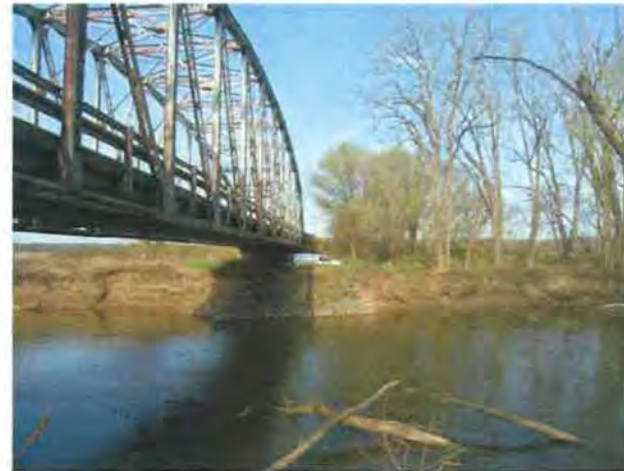
Photo 30: View of the western bank of the Eel River under the bridge.
