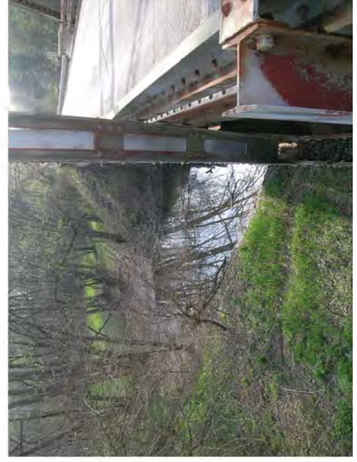
Photo 20: Looking at a ponded area near the eastern abutment.
