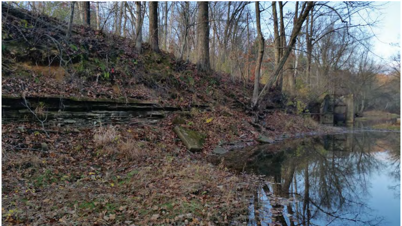
Photo 16: East bridge looking downstream (southwest) at south bank bluff and old dam
