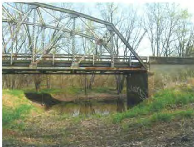
Photo 27: Looking north at the floodplain and ponded area adjacent to the eastern abutment.
