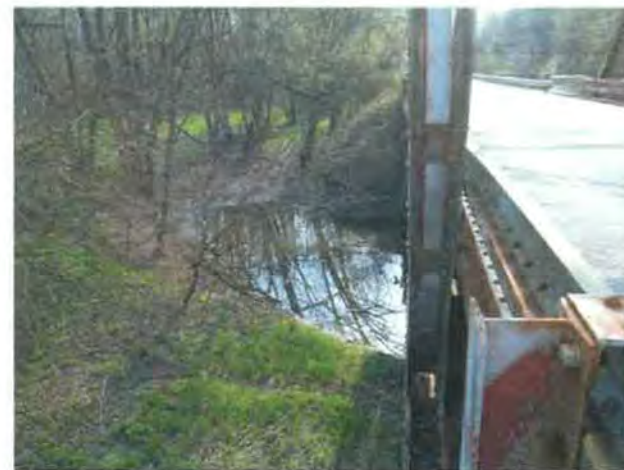
Photo 20: Looking at a ponded area near the eastern abutment.
