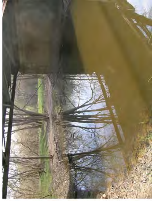
Photo 28: View (2) of the ponded area.
