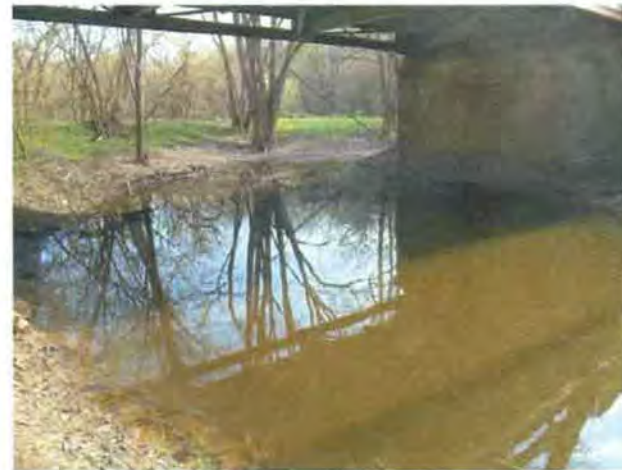
Photo 28: View (2) of the ponded area.
