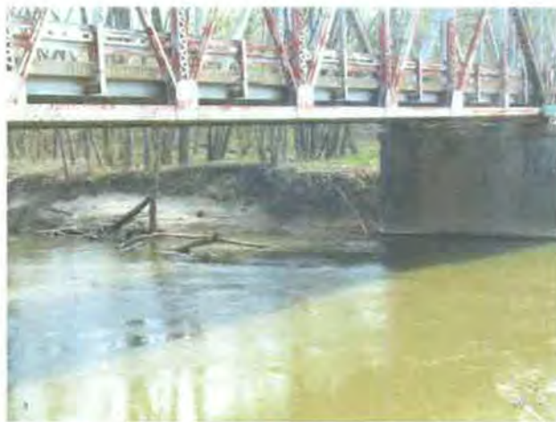
Photo 31: View of the NE bank of the Eel River under the bridge.
