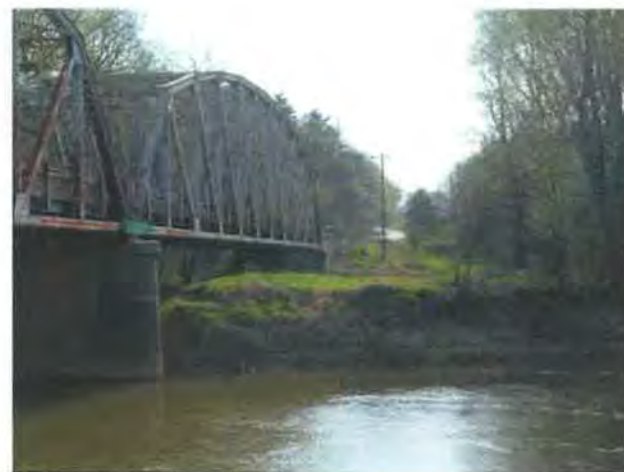
Photo 32: View of the SE bank of the Eel River under the bridge.
