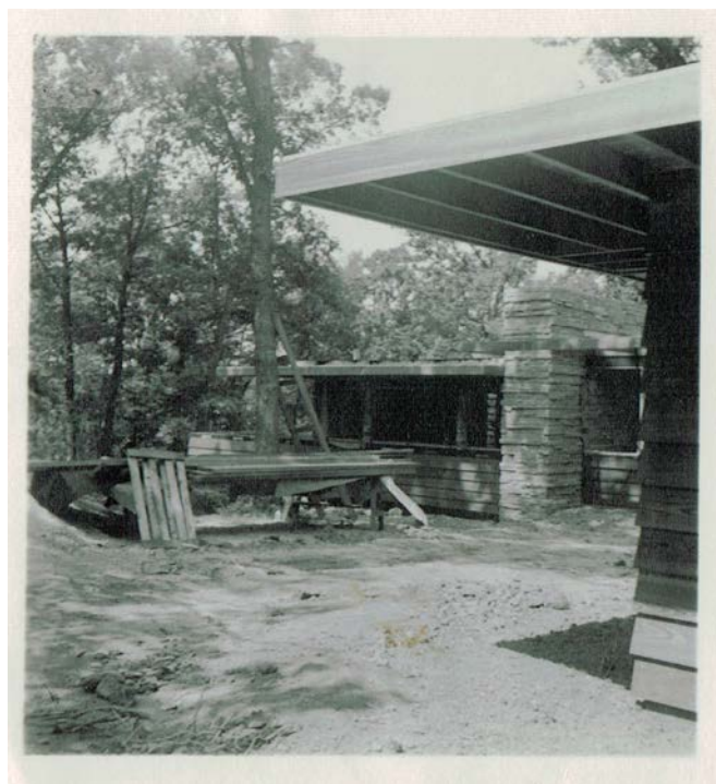
Figure D: House under construction, view north from corner of bedroom wing toward family wing (1942)
