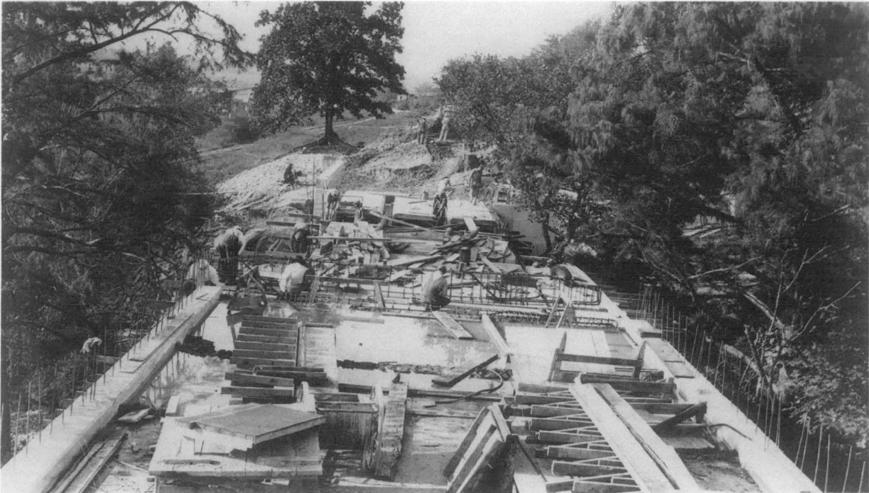
Figure 2: Construction of the Marr's Creek Bridge in Pocahontas, 1934. Courtesy Arkansas Highway and Transportation Department-Bridges Division.
