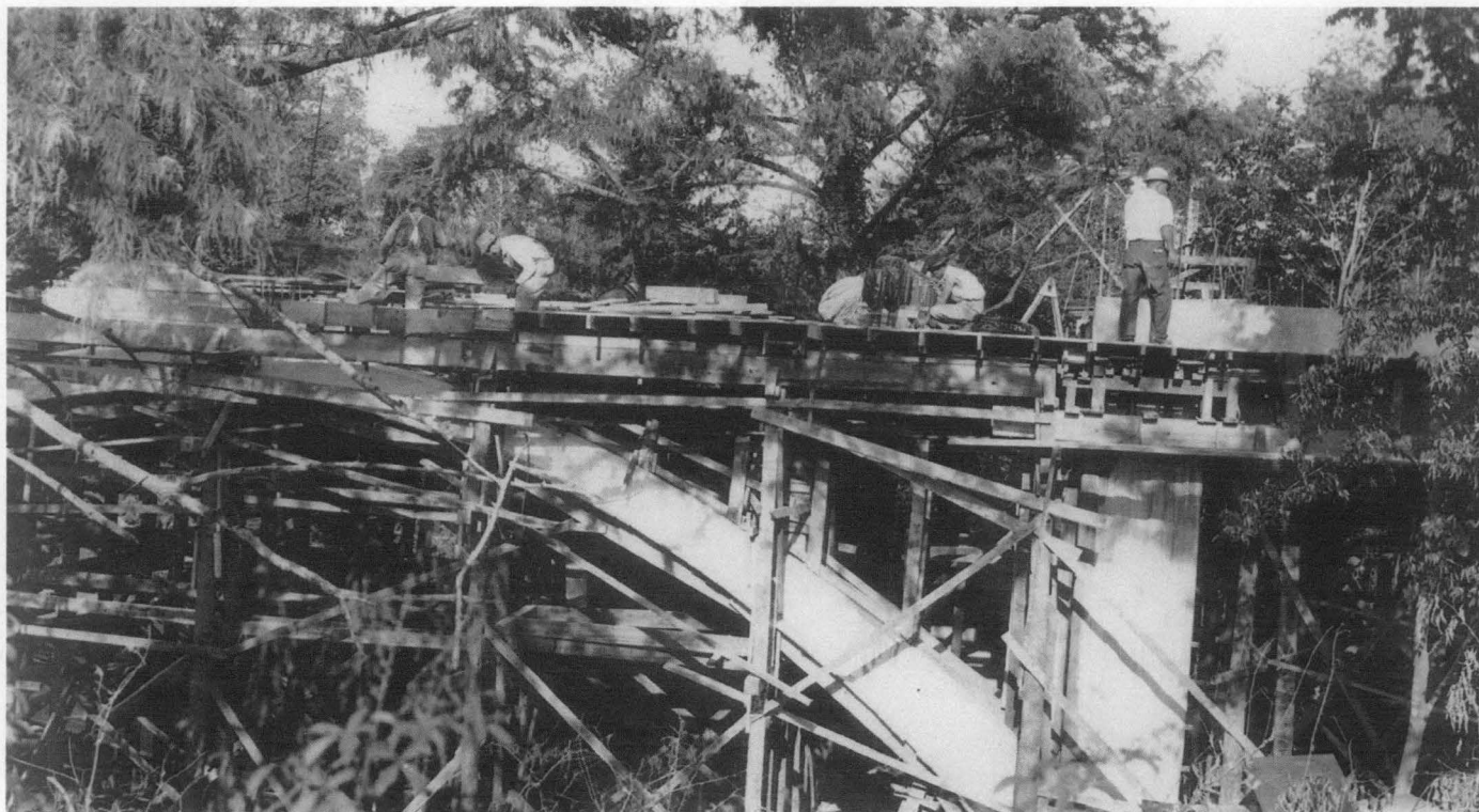
Figure 4: View of the construction of the open spandrel arch on the Marr's Creek Bridge in Pocahontas, Randolph County, AR. Courtesy Arkansas Highway and Transportation Department-Bridges Division.
