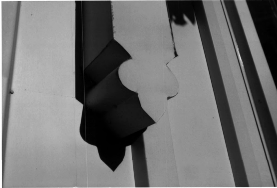
Photo 14. Detail near west door on south elevation, showing the shaping of aluminum to fit the wood part.
