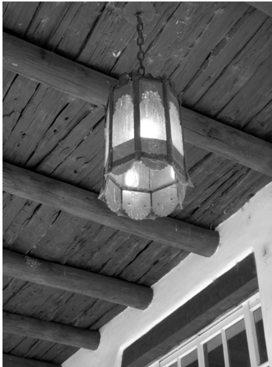
31 of 40. Interior, south portal, wrought-iron and punched-tin lantern designed by Meem.
