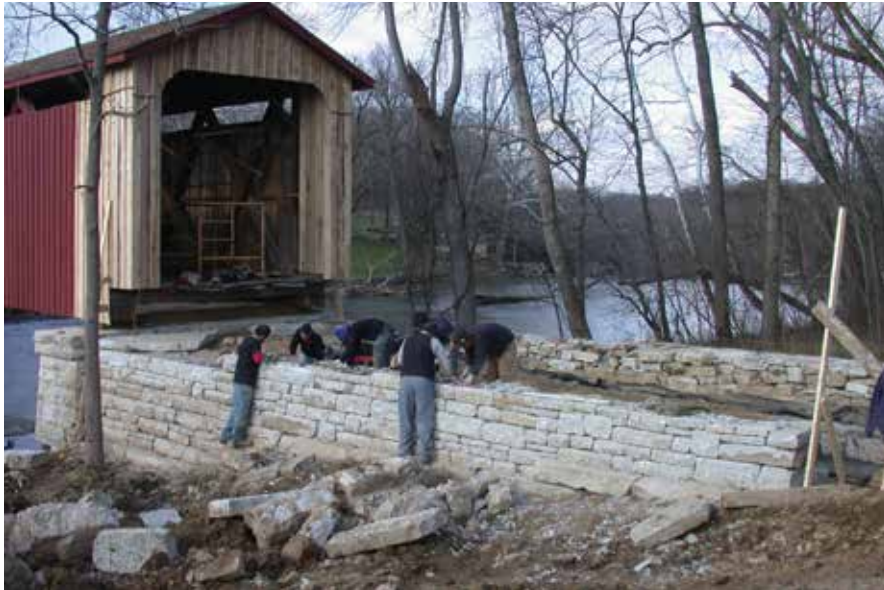
Figure C2.10 Dry-laid wingwalls under construction. The reconstructed bridge portal is complete except for paint. The top of the falls is visible in the background. McAlister Stone LLC, January 2005.
