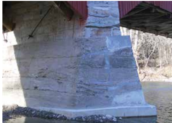
Figure 3.4c-d Structural failure due to cracking in the center pier at Deers Mill Bridge, IN. The crack was patched and a new concrete apron poured underneath to stabilize the pier.
