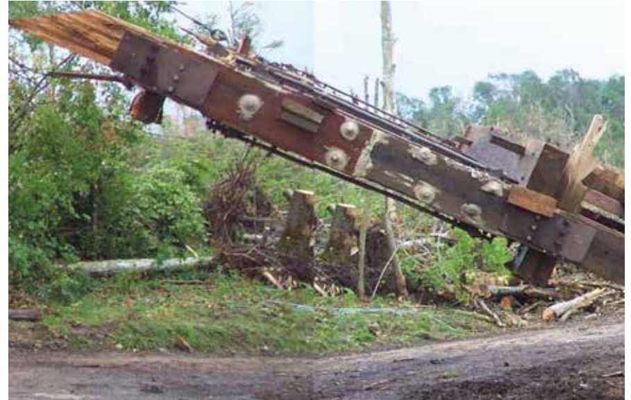
Figure C9.6 Pulling the bridge out of the water. Previous repairs included liberal use of epoxy adhesives, making it impossible to reuse these lower chord timbers. James Barker, J.A. Barker Engineering, Inc., 2008.
