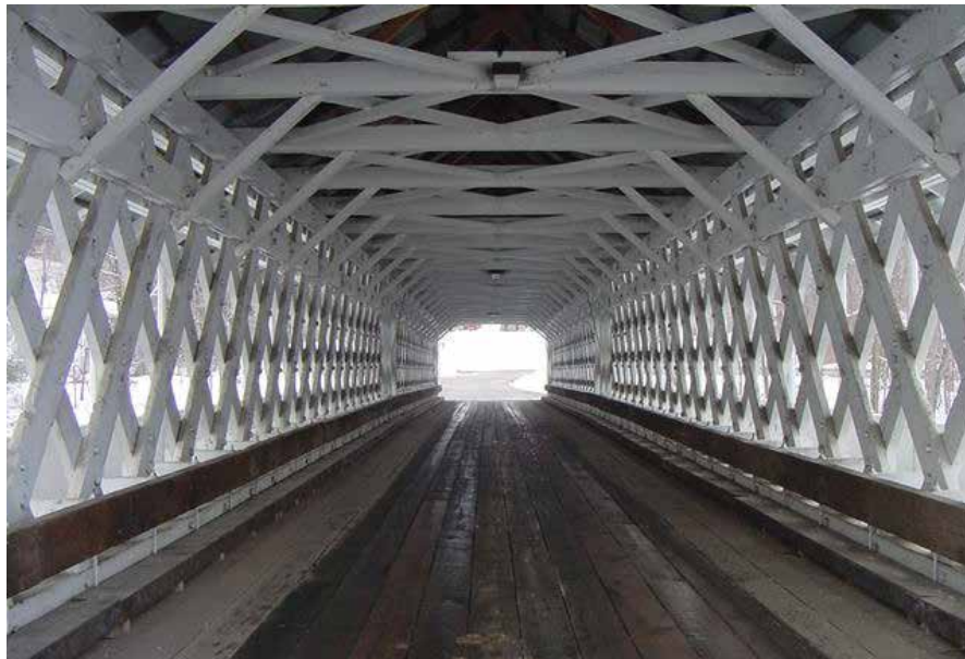
Figure C1.5 Interior view of trusses, deck and unpainted 4" x 12" bridge guardrail. Sean T. James, 1998.
