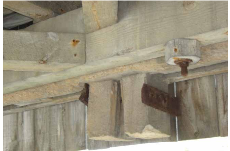
Figure C10.7 Typical split tail end of verticals at Node N12 (north truss). Josif Bicja, August 2007.
