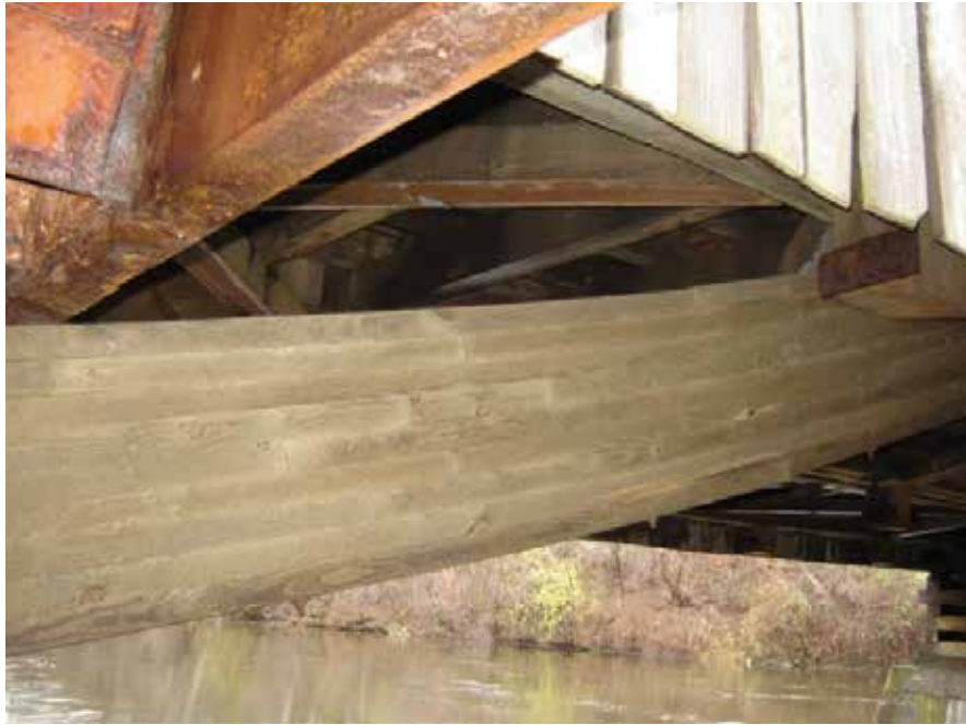
Figure C10.4 Buckling of west end of the south arch. Sean T. James, November 2006.
