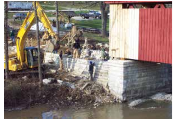
Figure 3.3e-f Reconstructing the dry-laid wing wall behind the abutment at Cataract Bridge, IN. The reconstructed wall matches the original in composition, color and texture, while improving its strength.
