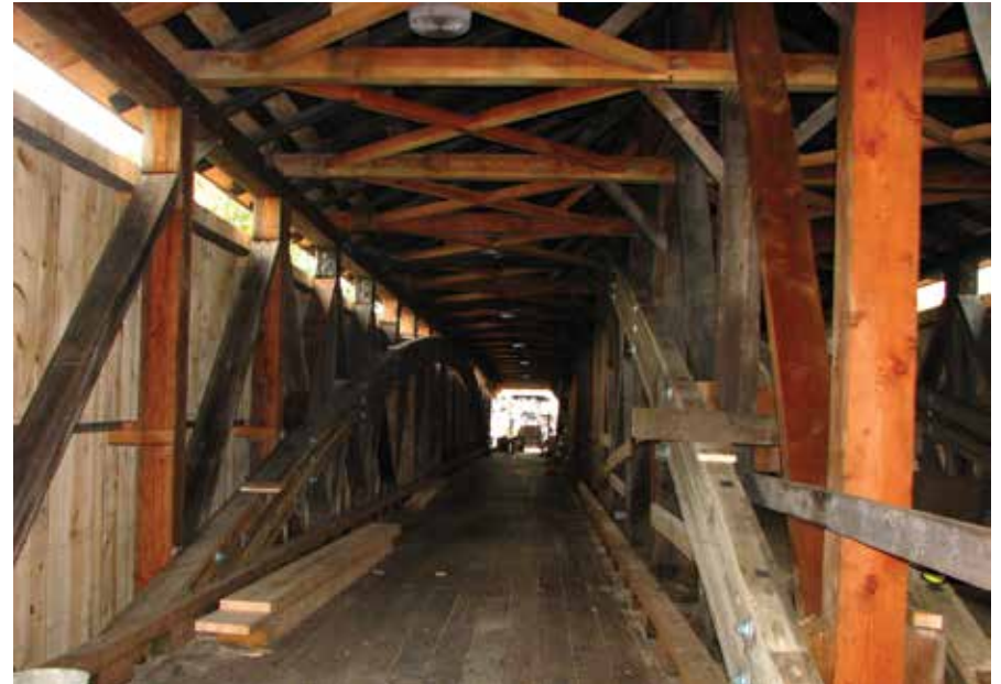
Figure C10.21 New upper lateral bracing and arches on eastbound barrel. William Caswell, September 2012.
