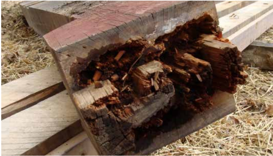
Figure C5.5 This photo of the top of a post shows the typical condition of truss members between joints. Timothy Andrews, 2009.
