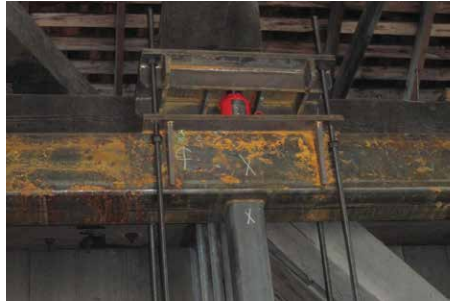
Figure C6.7 One of twenty 50-ton jacks on temporary steel truss used to lift the bridge to proper camber, 2013.
