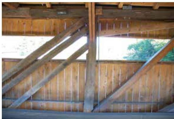
Figure 2.4c-d Top: Replacing in kind with traditional notched sway bracing, fastened with a nail. Below: Inserting replacement timbers in kind while preserving many of the original hand hewn braces at Taftsville Bridge, VT.
