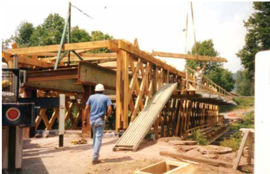
Figure C4.3 Prior to the start of the 2001 rehabilitation, a steel falsework system with adjustable work platforms was installed. This photograph shows the falsework and the installation of new tie beams. Delaware County Department of Public Works (DCDPW).
