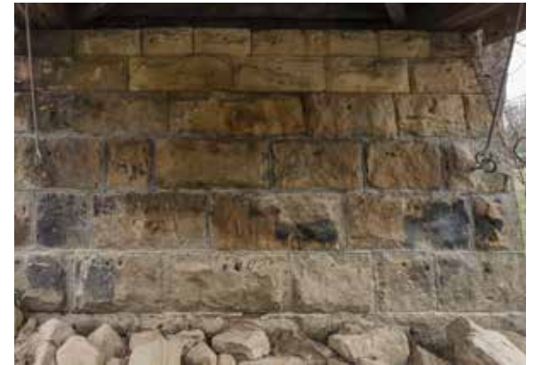
Figure 3.4e-f Chinking (filling joints with small stones) rather than the introduction of mortar is the proper rehabilitation method for a dry-laid wall. Below: Preserving the original stonework at Rinard Bridge, OH. The hold down rods (an original design feature) have been replaced in kind, which helps keep the bridge in place during a flood event.
