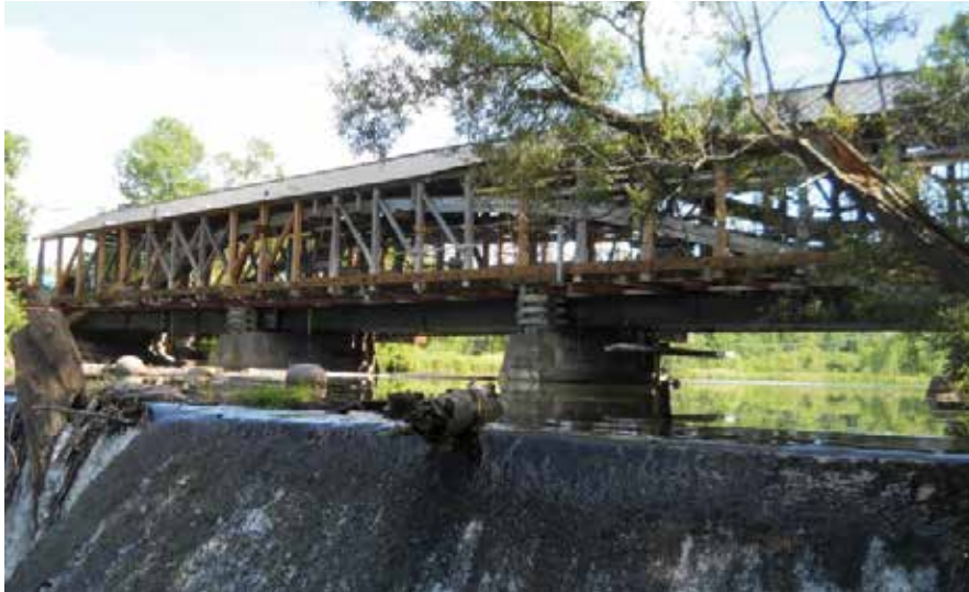
Figure C10.14 Downstream bridge elevation shored during construction, looking south. Two steel beams were installed on the underside of the bridge and fitted between timber cribbing at the piers. Josif Bicja, July 2012.
