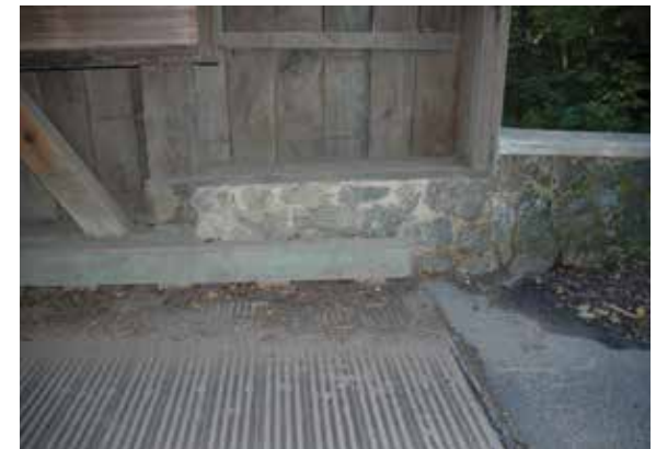
Figure 2.6e Diagonal decking found at Rinard Bridge, OH. Figure 2.6f Nail-laminated decking is typically not a historically correct treatment and should be replaced in most cases (unless it was the original decking system).
