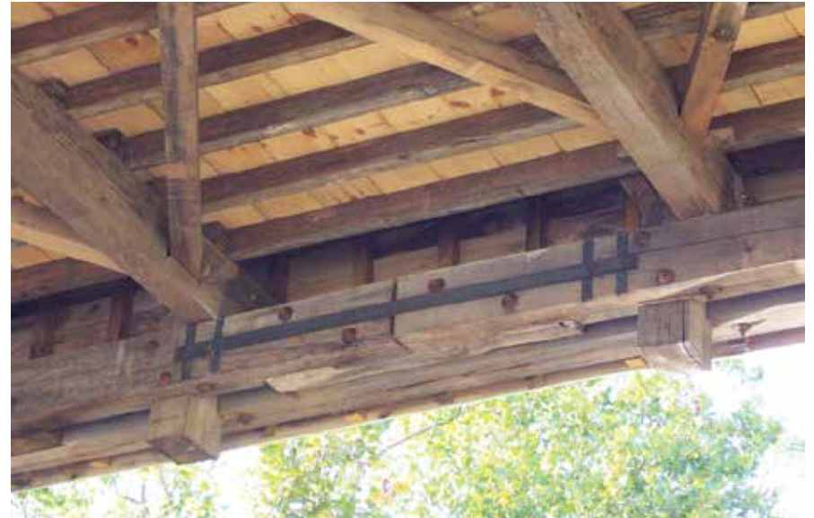
Figure C9.13 Steel strap and inlays reinforce a lower chord splice in the rebuilt bridge. James Barker, VS Engineering, Inc., 2014.
