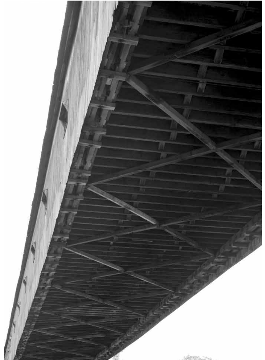
Figure C3.2 View inside bridge showing notched lattice truss, prior to being closed. HAER NH-8-10, Jet Lowe, 1984.
