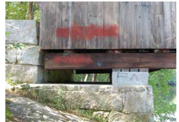
Figure 3.2e-f A circle of scour around a center pier at Medora Bridge, IN. Below, a bolster beam for a Town lattice truss at Henniker Bridge, NH. It sits on a granite pedestal, with spacer blocks below and on top, which allows for easy maintenance and good air circulation.
