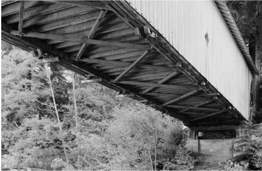
Bottom chords, lower lateral bracing, and floor joists support this Smith truss.
