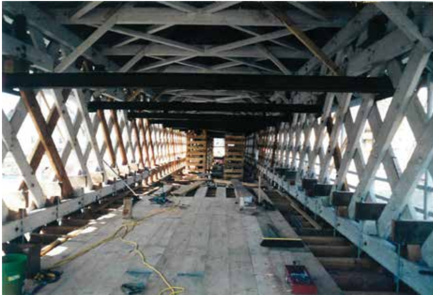
Figure C1.12 Installation of floor beams and decking; note steel needle beams supporting the top chord, spaced at every third lattice opening, 1998. Sean T. James, 1998.
