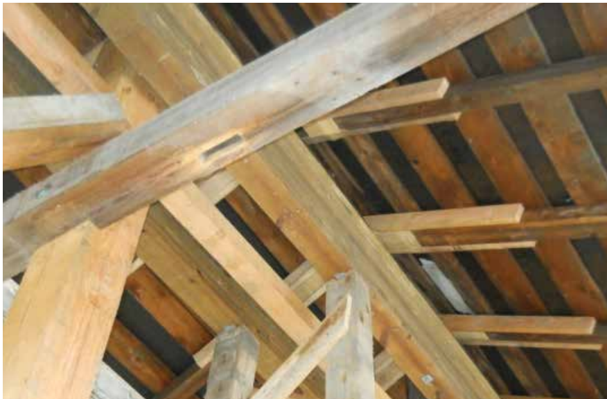
Figure C10.18 Typical sistered roof rafters. Josif Bicja, July 2012.
