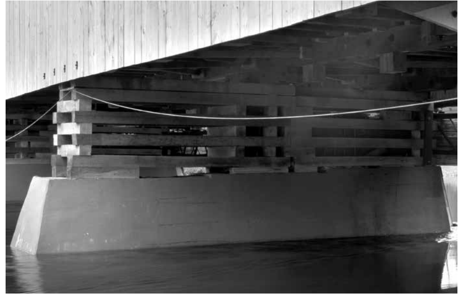
Replacement timber cribs sit atop concrete piers to support the Pulp Mill Covered Bridge, VT.
