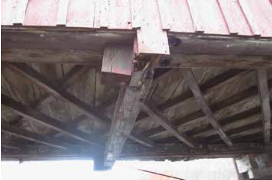
Figure C8.4 Lattice floor joist system, and lower tie beam added after original construction. SCLA.
