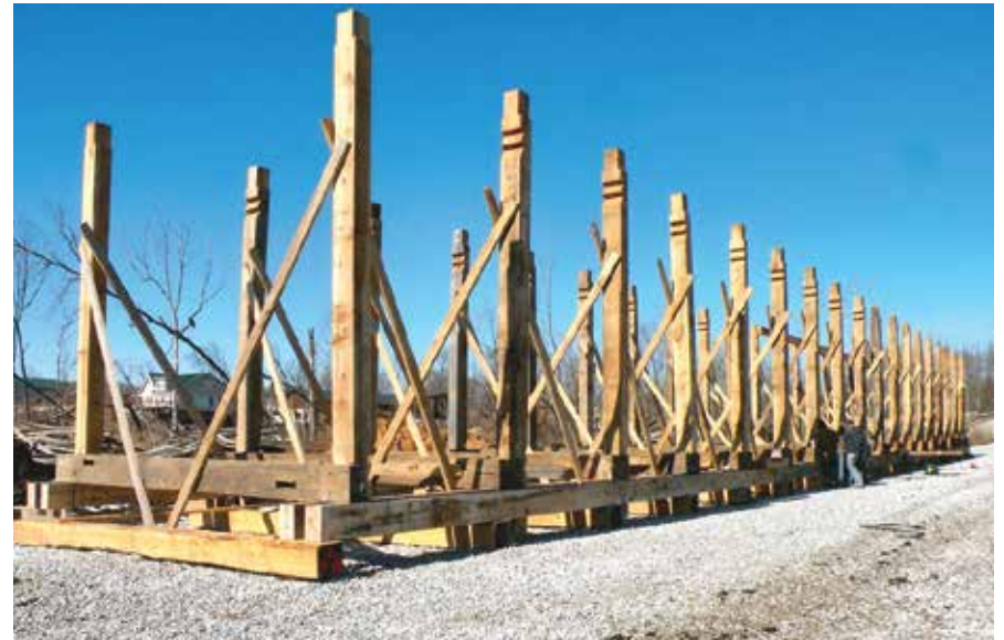
Figure C9.8 Start of framing for one span; blocking provides camber. Double notching visible at tops of posts. Arthur Gatewood, 2010.
