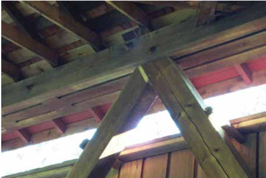
Figure C2.9 Trusses were jacked to restore camber, then held in that position by inserting shims at the top of truss compression diagonals, as shown here. J. A. Barker Engineering, 2004.
