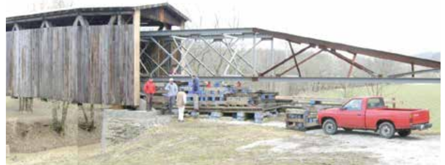
Figure C7.7 Panorama of steel truss inside of bridge, after camber was restored to 9". The center pier was removed after the truss was repaired. KTC, 2007.
