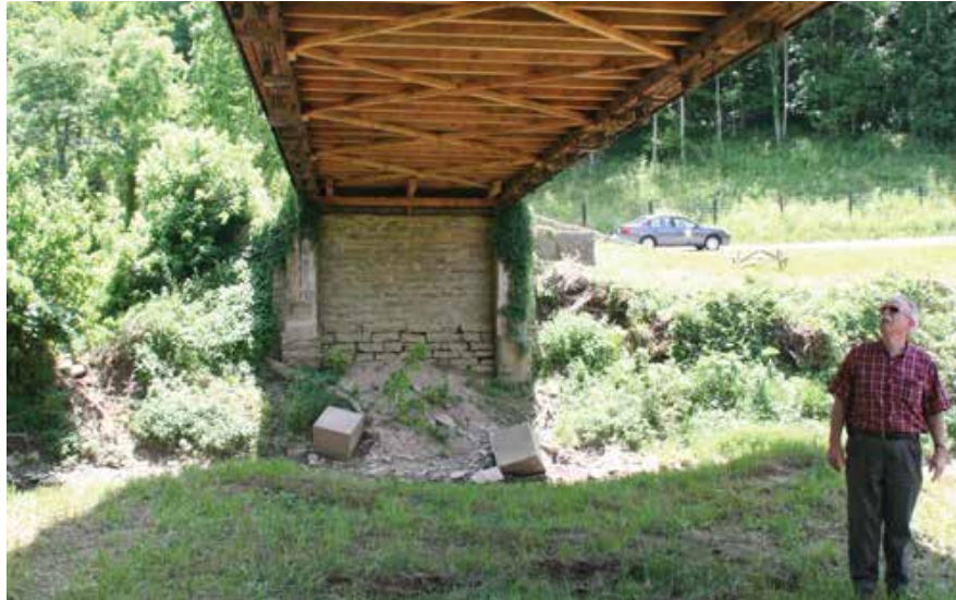
Figure C7.11 Patrick Kennedy inspects the rehabilitated lower chords and flooring system, Jen Spangler Williamson, 2010.
