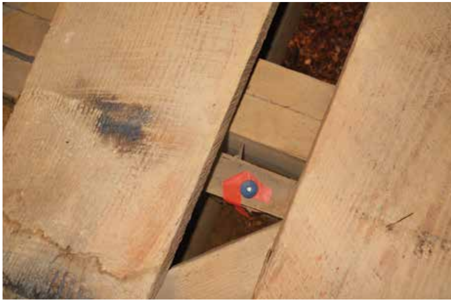
Figure C11.9 Span 1, near floor beam 2, showing separation between stringer 4 boards. TranSystems, 2012.
