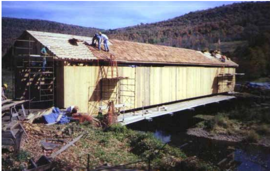
Figure C4.10 The metal roofing was replaced with traditional red cedar wood shakes, based on community preference. DCDPW.
