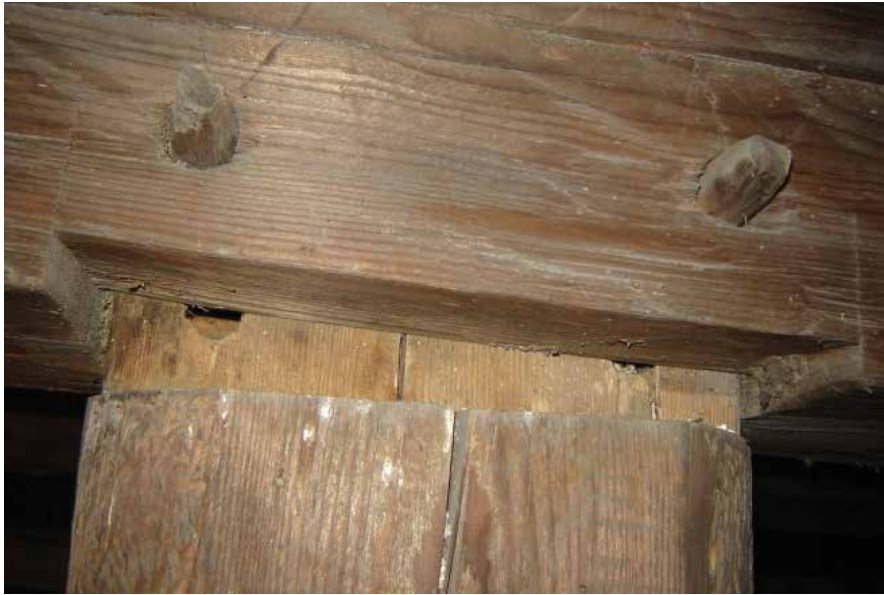
Figure C10.6 Truss vertical to top chord with failed connection at interior truss. Sean T. James, July 2007.
