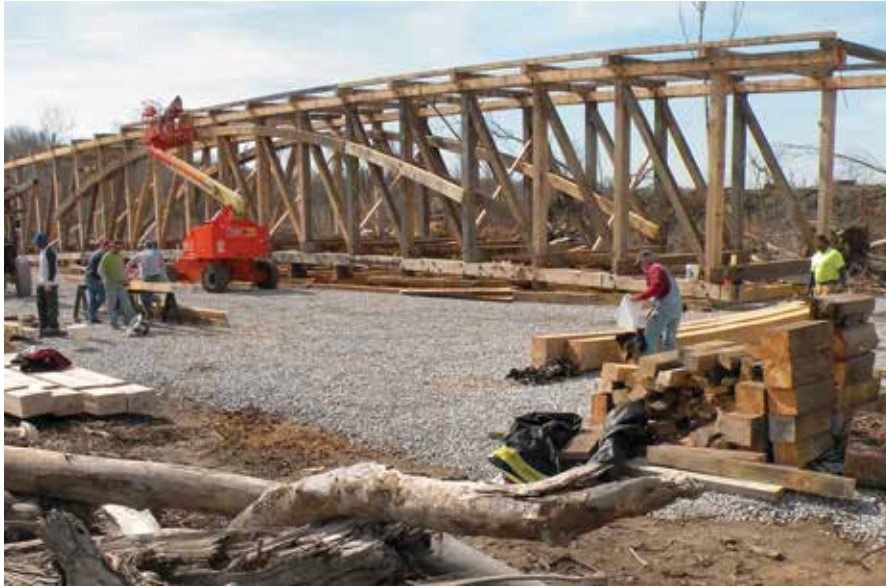
Figure C9.9 Start of framing for one span; blocking provides camber. Double notching visible at tops of posts. Arthur Gatewood, 2010.
