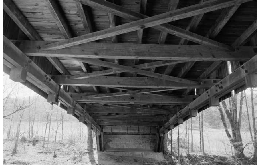
Stringer joists, laid parallel to the lower chords, sit atop the floor beams to support the deck.
