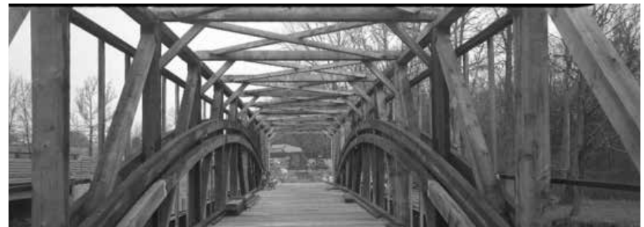
Figure C5.13 View of completed arches, trusses, bracing, and newly installed deck; awaiting curbing and sheathing. HAER MD-174-17, David Ames, 2010.
