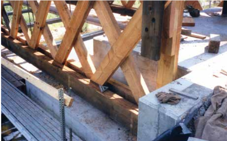
Figure C4.4 New concrete caps with pockets for longer trusses were installed on the abutments. DCDPW.
