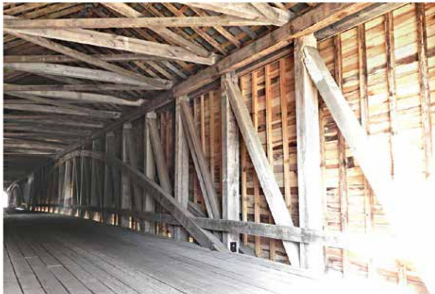
Figure C9.12 Bridge interior in 2011. Compare with Figures 3 and 4; all three were taken from the same place and looking in the same direction. Arthur Gatewood, 2011.
