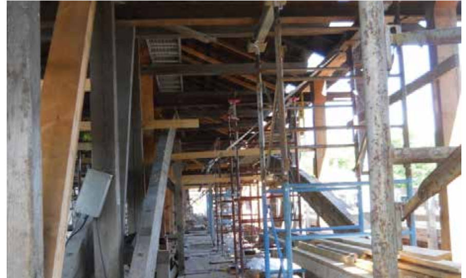
Figure C10.16 Temporary shoring system inside the bridge, looking east on eastbound barrel. Josif Bicja, July 2012.
