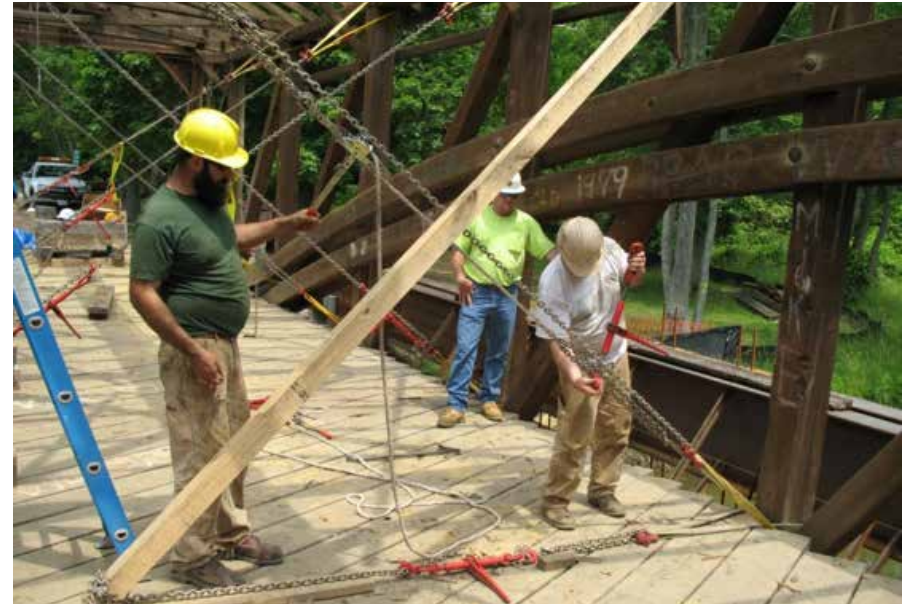
Figure C5.7 Cross chains installed to straighten the bridge in plan. Also note the deck planks are laid diagonally. The diagonal configuration was not original, and they were returned to a perpendicular arrangement later in the project. Jeremy Mauro, 2009.
