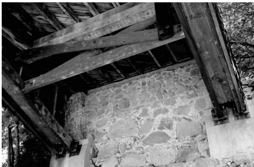
The stone facewall of an abutment. Reinforced concrete skewbacks support the arches.
