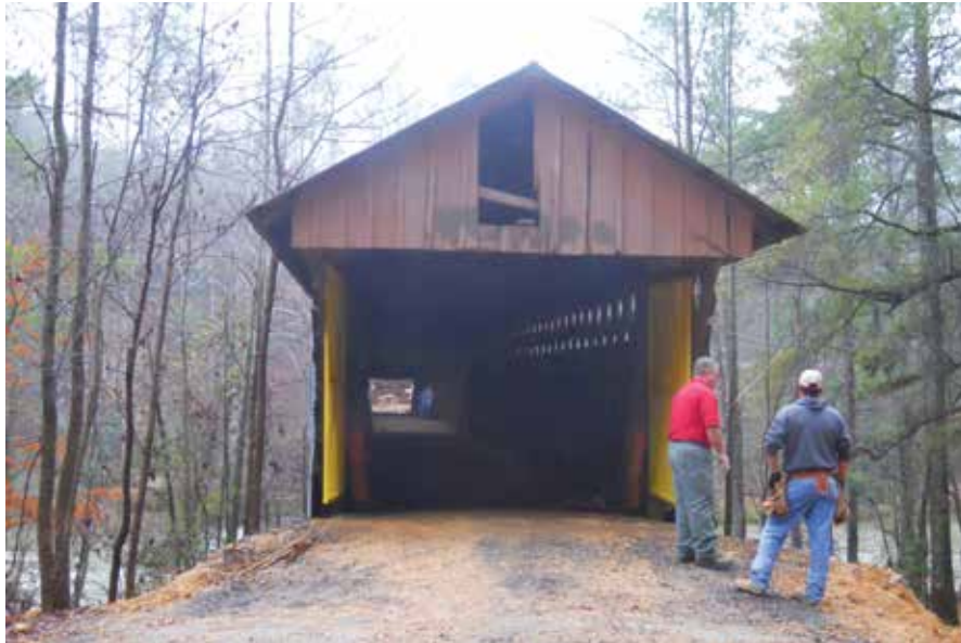
Figure C11.8 Abutment 1 showing gable with missing boards. TranSystems, 2012.
