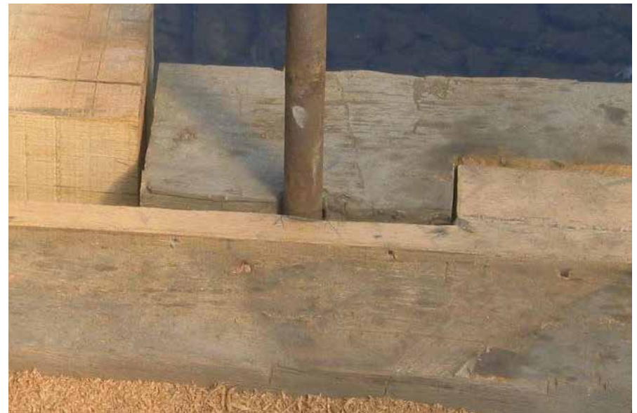
Figure C8.13 Joggle splice repair. SCLA.
