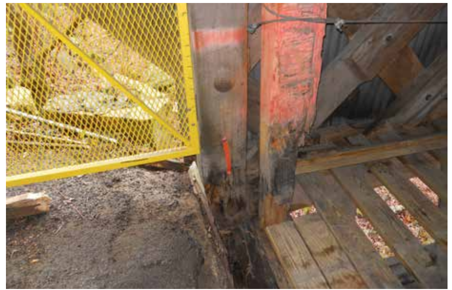
Figure C11.13 Right vertical post is rotted at abutment 4. TranSystems, 2012.
