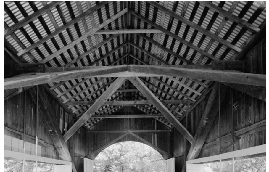
Rafters supporting purlins and sheet metal roofing. A collar tie braces every third pair of rafters.
