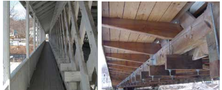
Figure C1.6 Exterior sidewalk showing bolster blocks and rod clamp system on right; original 4" x 5" molded handrail on left. Scott Wagner, 2005.
