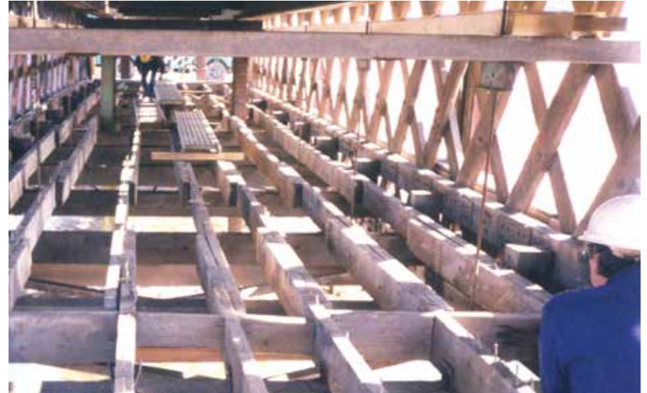
Figure C4.5 The 1976 floor system has been partially removed. The near edge of the floor is the transverse nail laminated decking. The longitudinal stringers are obviously not uniformly spaced. DCDPW.
