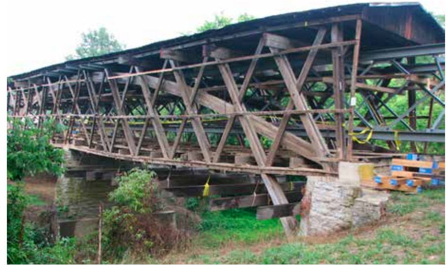
Figure C7.5 View of shoring system, with steel truss through bridge, with horizontal needle beams supporting the top chord. Note negative camber, which measured up to 21." William Caswell, 2007.
