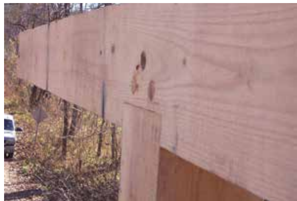
Figure 2.4a-b Top, a very poorly crafted, old but non-original housed mortise-and-tenon joint between a post and upper chord. Below, a finely crafted, tight fitting similar joint in the same bridge.
