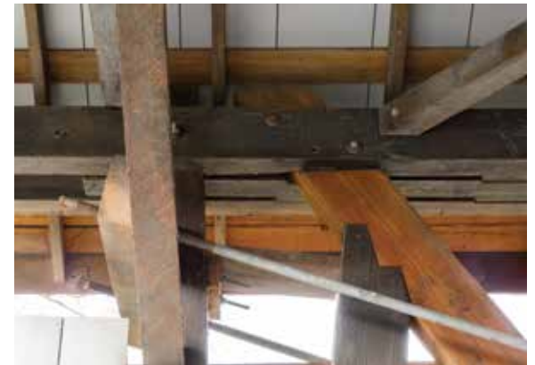
Figure 2.5e-f An example of a loose diagonal brace with traditional stepped notches in need of adjustment. Below, a replacement tension diagonal matches the double-stepped connection of the original post in a Smith truss at Rinard Bridge, OH.
