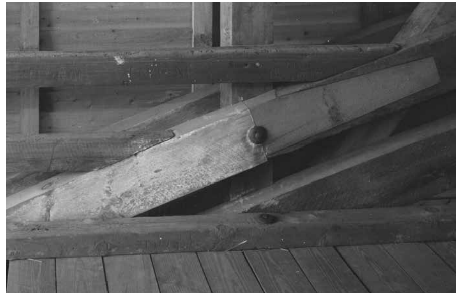
A splayed scarf joint repair abuts a replacement arch leaf. Both Burr-arch segments are secured with a single through bolt.
