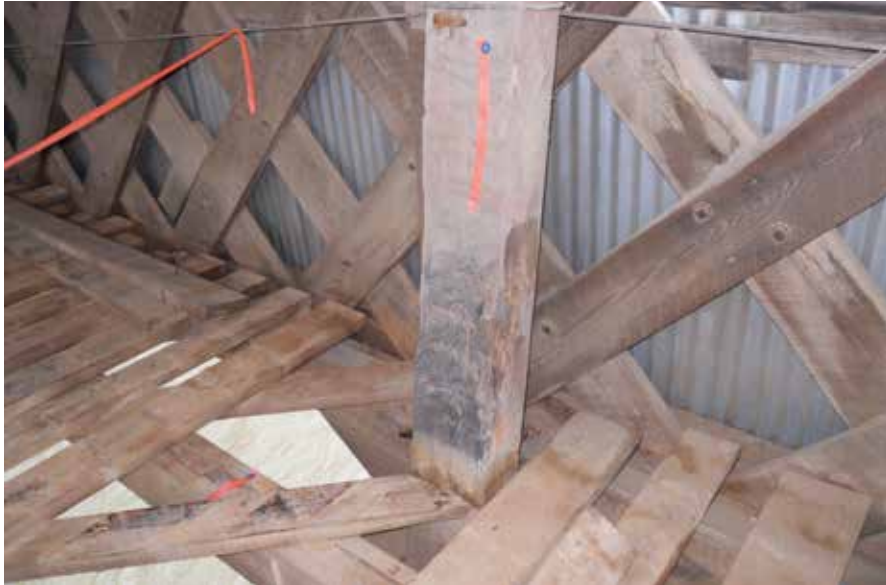
Figure C11.10 Vertical post at Pier 2 revealed deterioration on south side. TranSystems, 2012.
