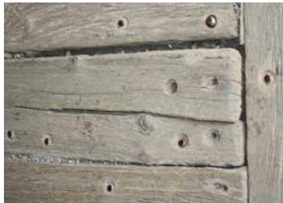
Figure 2.6c-d Newly installed longitudinal decking (running plank) at Forsythe Bridge, IN. Below, even a weathered and worn floor system should be inspected carefully to see if it could perform as required. Repairs and/or additional fasteners might preserve the floor's rich visual record of service.
