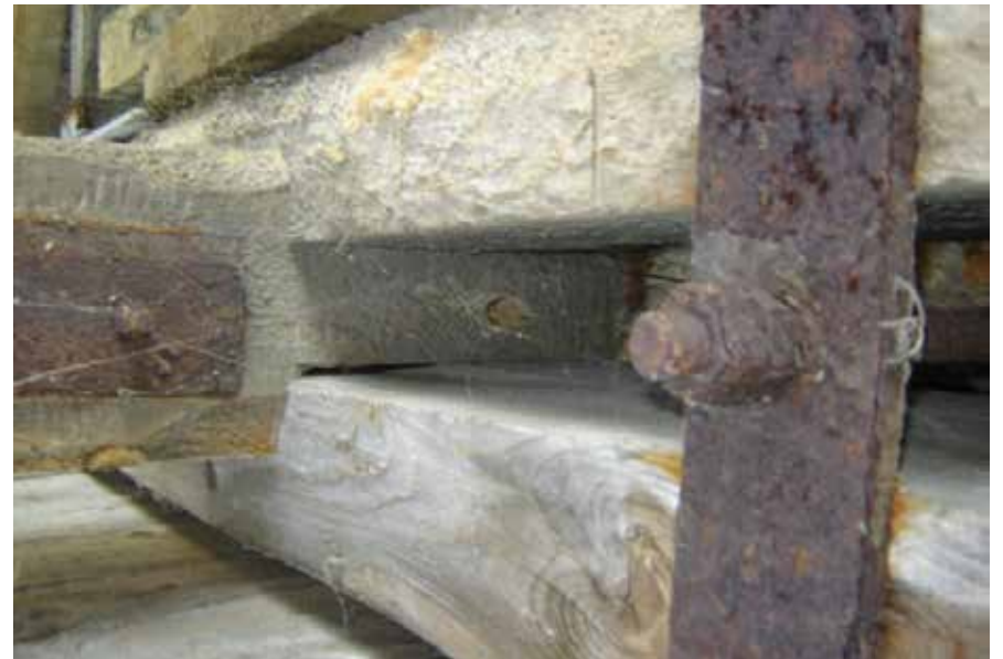
Figure C10.8 Notched end of vertical at connection with bottom chord at Node N4 (north truss).
