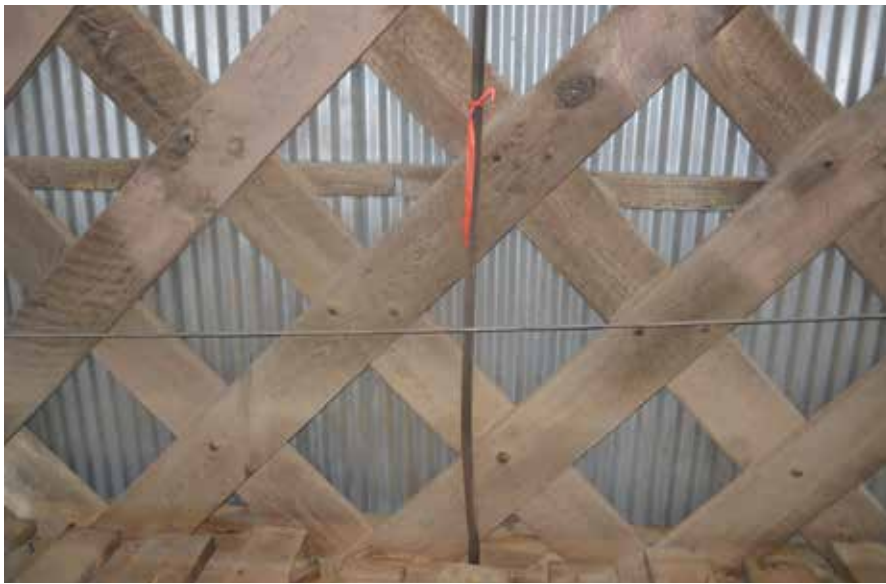
Figure C11.11 Span 3, south (right) side with bent hanger rod 1. Condition also observed at north hanger rod at floor beams 5 and 6. TranSystems, 2012.
