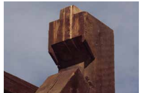
Figure 2.4e-f The repair of the jowl of this low-stressed post incorporates salvaged, in kind material at Gilpin's Falls, MD. Multiple close-fitting pieces of wood were used in the repair process, as was waterproof glue.
