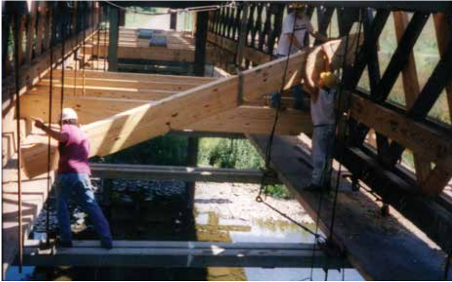
Figure C4.6 New transverse glulam floor beams were carefully threaded through the lattice opening-s atop the lower bottom chord. DCDPW.
