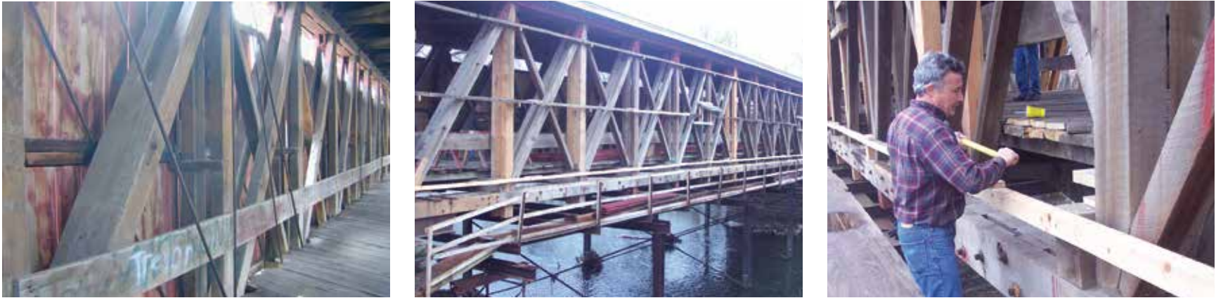
Figure 0.9a-c The 2005 rehabilitation work on the Eldean Bridge in Ohio is a good example of repairing and replacing missing historic character-defining features, and reversing an earlier inappropriate intervention. The 1960s reinforcing rods were removed on the 1860 Long truss, and replaced with wooden wedges driven in at the base of the diagonal counterbraces, thus prestressing the truss as prescribed by Stephen Long.
