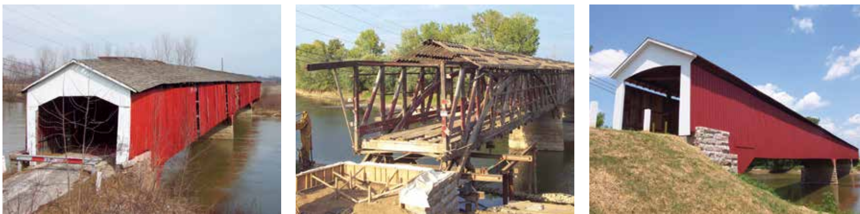
Figure 0.6a-c Before/During/After photos of Medora Bridge, IN. A complete rehabilitation was necessary due to failing abutments and a deteriorated roof causing decay in truss members. The crew carefully took apart the abutments, poured a new reinforced concrete slab, and put the original stones back in place.
