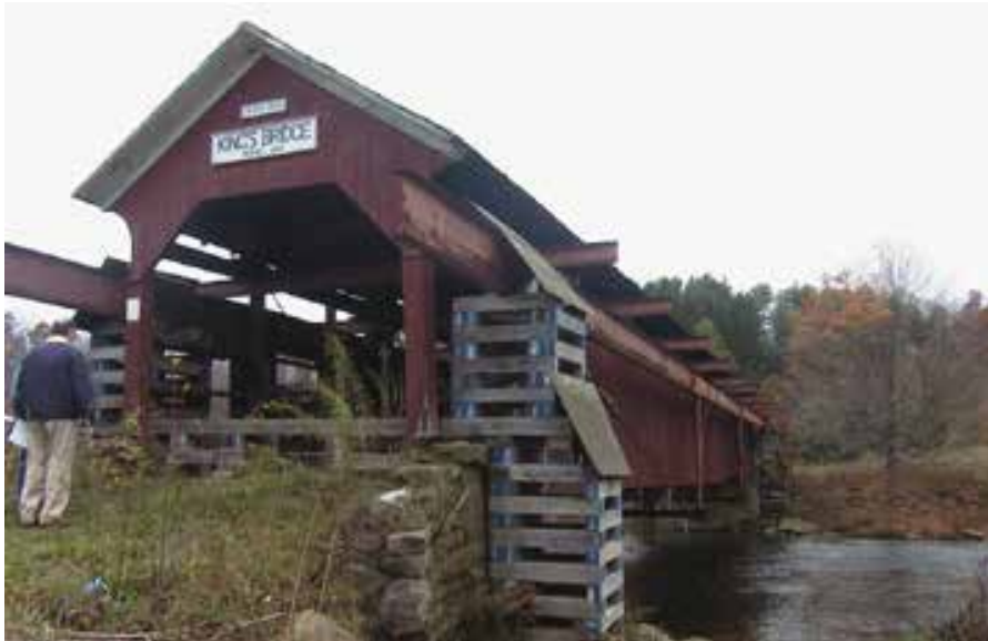
Figure C8.2. Bridge before rehabilitation with stabilization falsework in place at east portal. SCLA.
