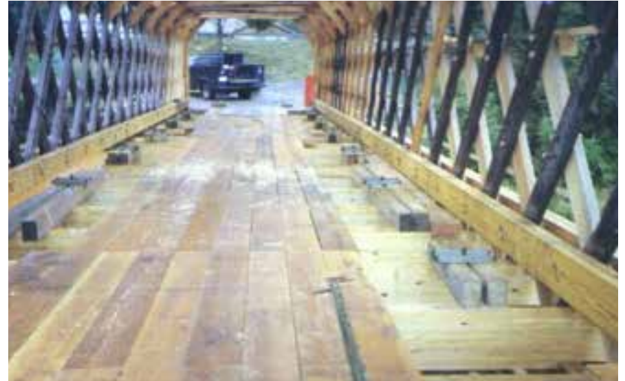
Figure C4.7 Staggered longitudinal deck planks have been installed; these were then covered with hardwood running planks. Note the darker lattice elements, which are original. DCDPW.
