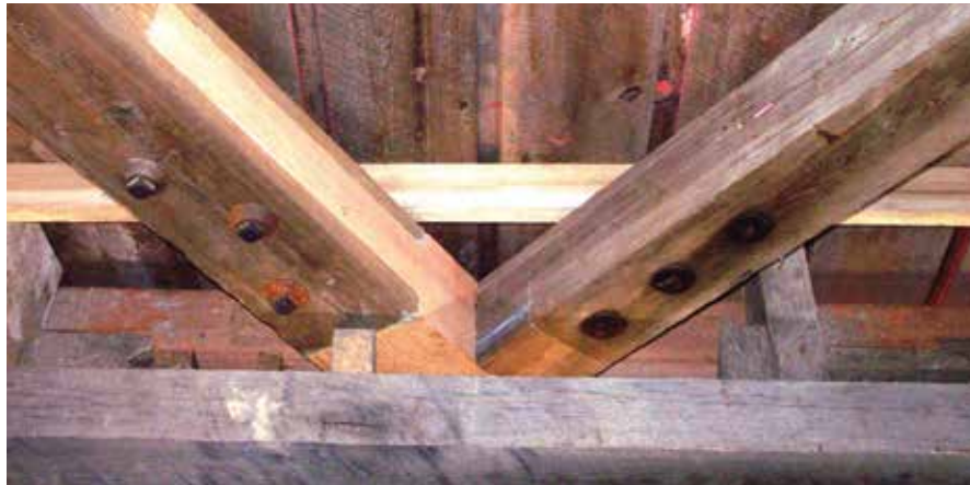
Figure C2.7 Timber repairs using new Douglas fir (left) were conspicuous. Those using salvage from original timbers (right) were nearly invisible. The Douglas fir repairs, having weathered a few years, are now less noticeable. J. A. Barker Engineering, 2004.
