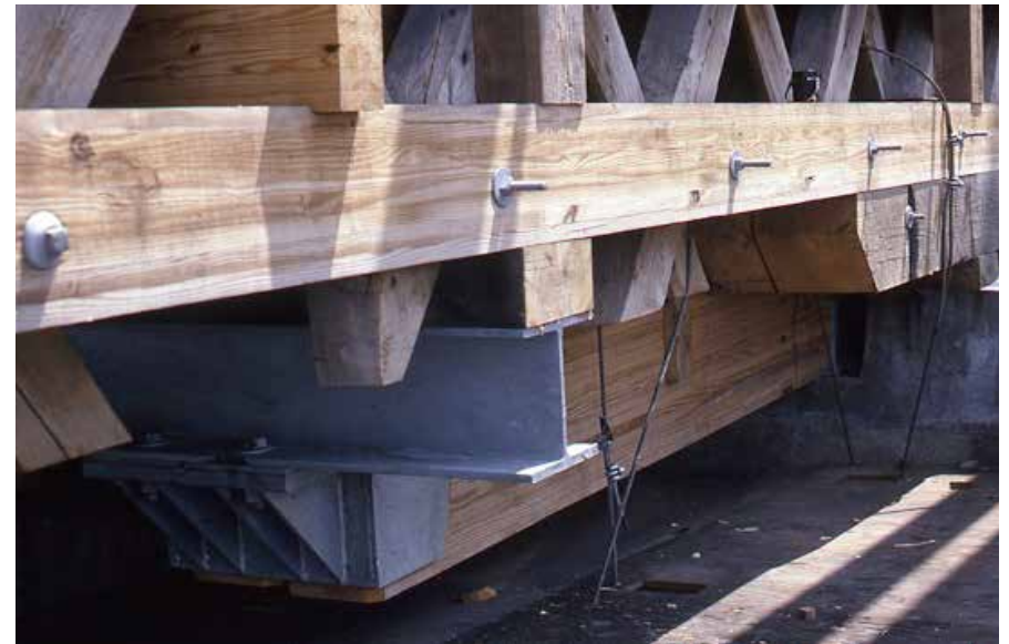
Figure C3.8 White oak bed timber and glulam bolster beam in new concrete footing, supporting truss. James L. Garvin, June 1989.
