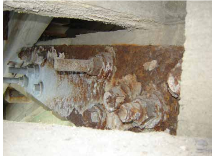
Figure C10.5 Severely corroded splice plate of interior truss at west span. Josif Bicja, August 2007.
