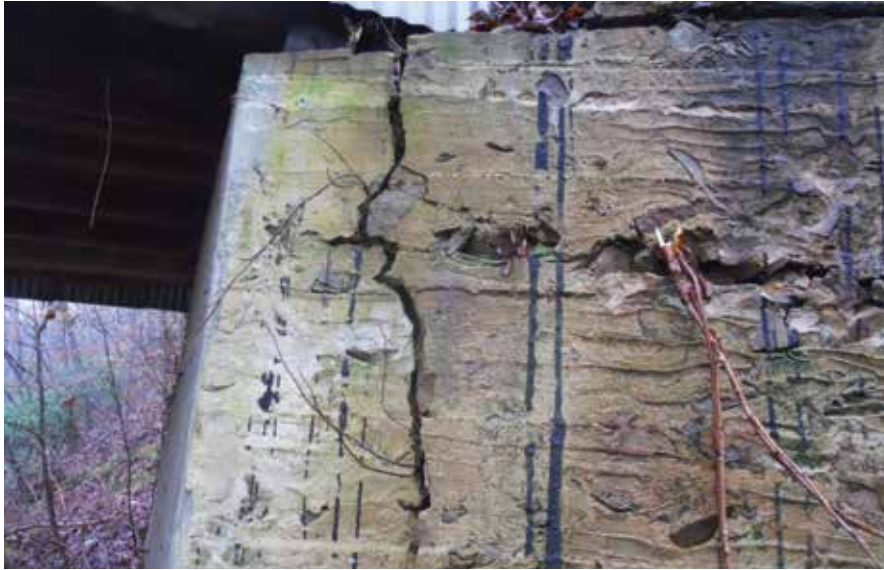
Figure C11.14 Wide crack in abutment 4 breastwall. TranSystems, 2012.
