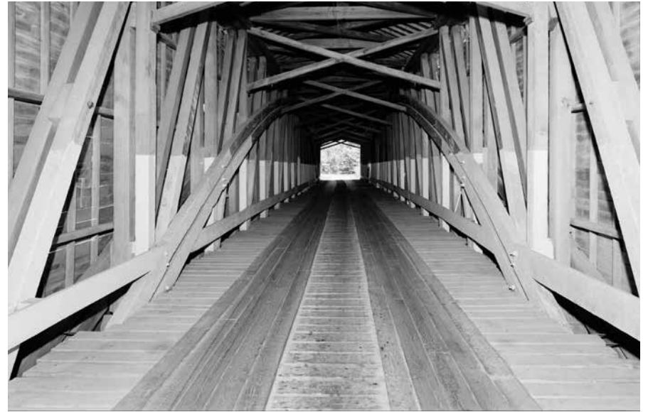
Running planks laid atop transverse decking provide an added layer as a wearing surface.
