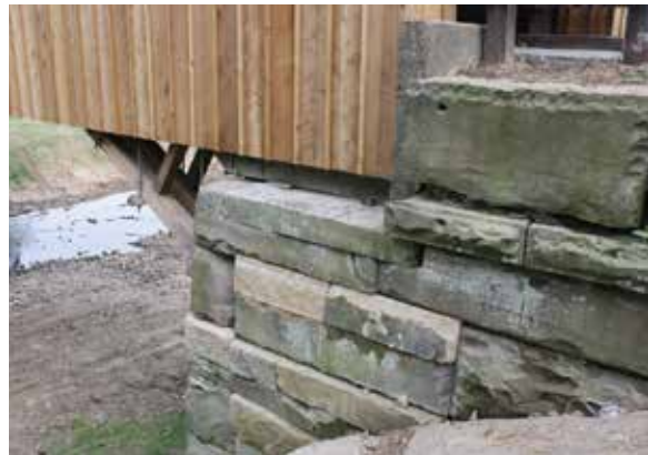
Figure 3.3a-b The timber bearing seat was rotted at Otway Bridge, OH, and replaced by a solid new timber bearing seat (bolster beam, below). Several stones were kept in place in the abutment, while some were replaced in kind.
