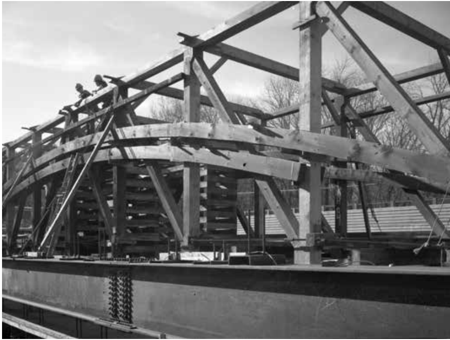
Figure C5.7 Cross chains installed to straighten the bridge in plan. Also note the deck planks are laid diagonally. The diagonal configuration was not original, and they were returned to a perpendicular arrangement later in the project. Jeremy Mauro, 2009.
