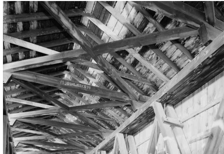
An upper lateral bracing system, with a series of knee braces at every tie beam.
