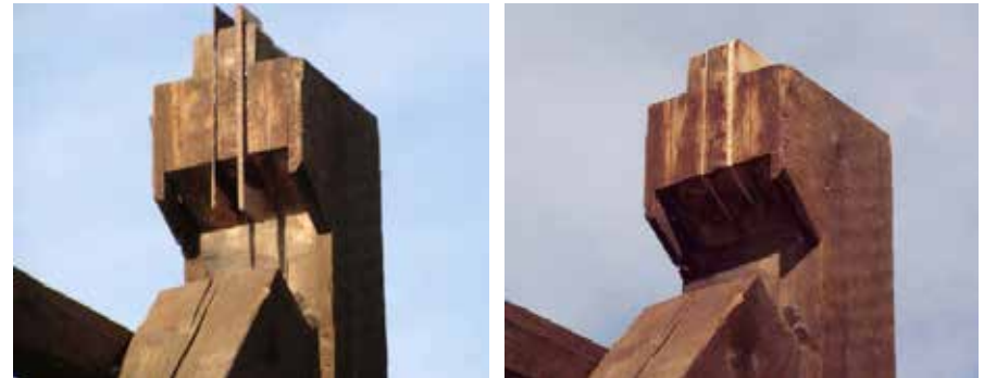
Figure C5.11 and Figure C5.12 The repair of this post required three stages of glueing to create a tight fitting Dutchman for this complex timber joint. Timothy Andrews, 2009.
