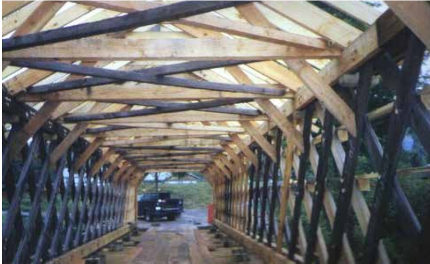
Figure C4.8 Most of the original upper lateral members were retained, but the tie beams and knee-braces were replaced with stronger components. Traditional wooden peg connectors and matching timber wedges were used, similar to those in the original construction. The darker upper lateral members are original. DCDPW.
