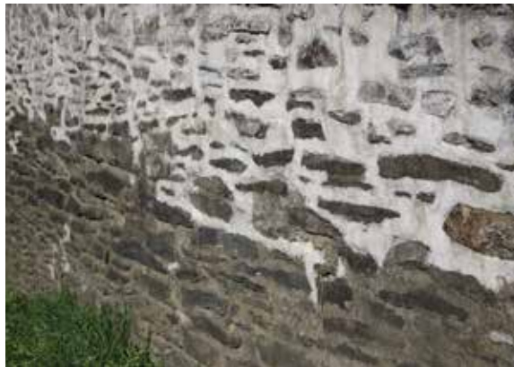
Figure 3.3c-d The reconstructed wingwall at Eldean Bridge, OH, while being cleaned of all loose mortar and being prepared for repointing. Figure 3.3d Not recommended: Mortars should be analyzed to determine compatibility with the surrounding masonry components. Mortar repairs should match both the color and strength of the historic material.
