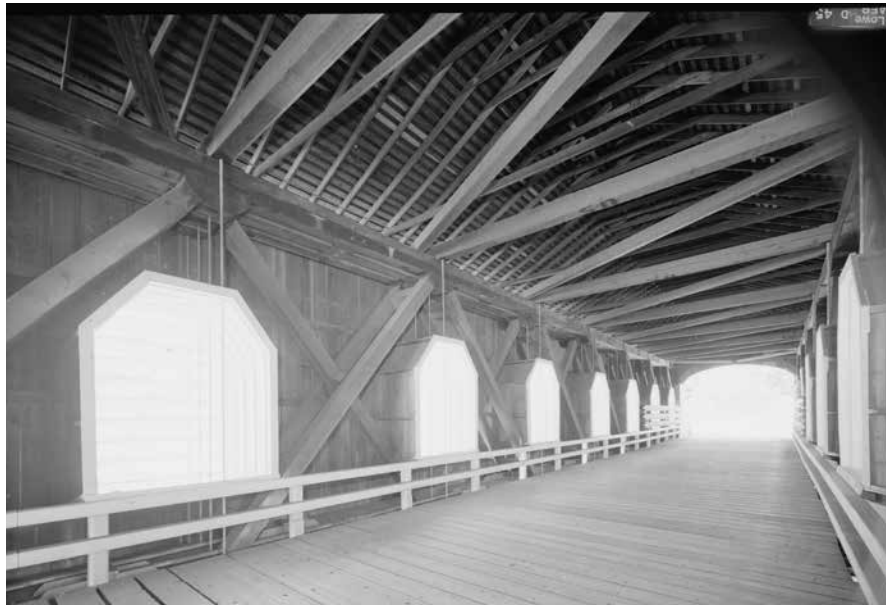
Figure C6.4 Interior of bridge showing center spans of Howe truss and boxed windows prior to rehabilitation. HAER OR-136-7, Jet Lowe, 2004.
