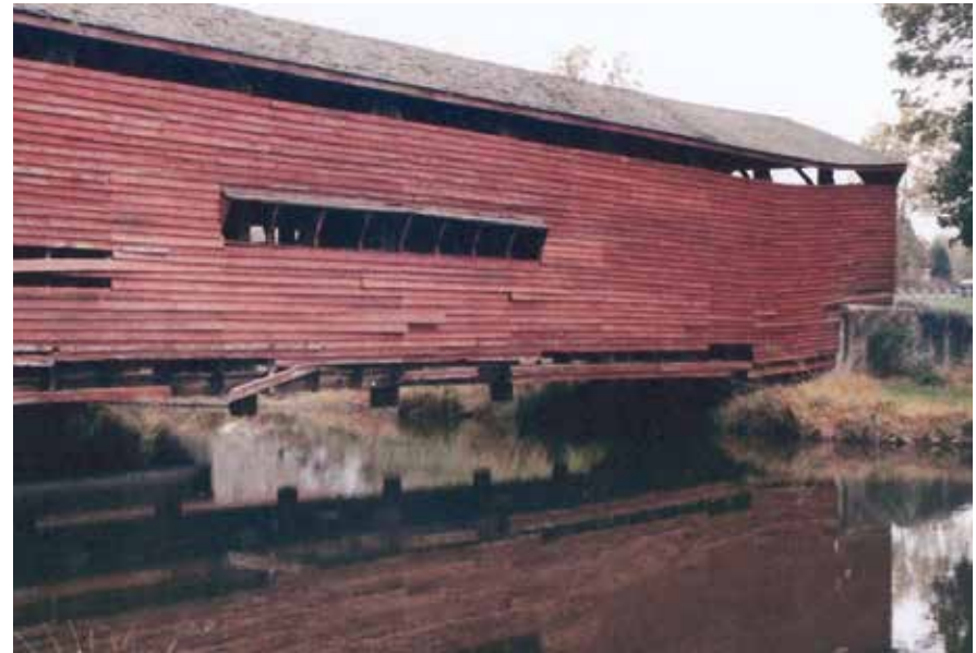
Figure C5.4 View of the bridge four years before the rehabilitation project. Failures in the lower chord contributed to the noticeable negative camber. W. Earl Simmers, 2005.
