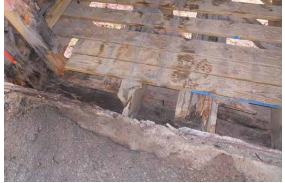
Figure C11.12 Abutment 4 showing deteriorated ends of stringers. TranSystems, 2012.
