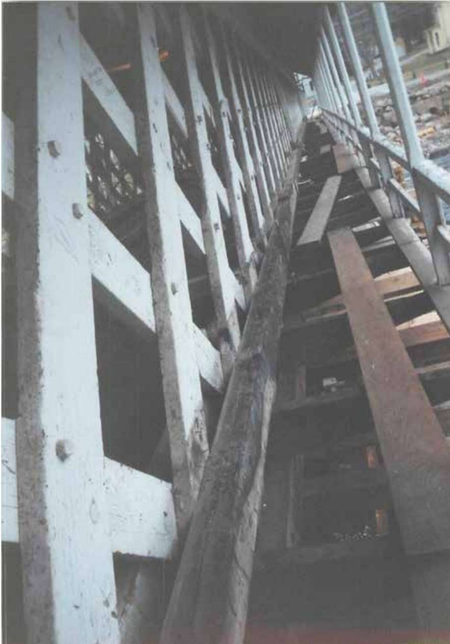
Figure C1.10 Previous fire damage of lower chord. Sean T. James, 1998.
