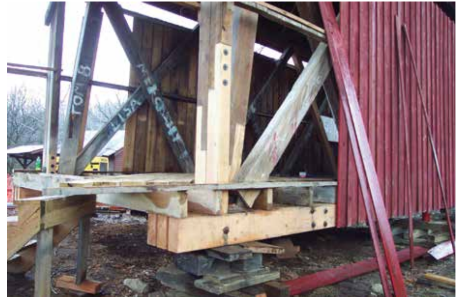
Figure C2.8 Decay at the bearings required extensive reconstruction. At the southwest corner, shown here, the two shorter lower chord timbers were replaced, while new ends were spliced onto the longest chord timber, both end posts, and a diagonal. J. A. Barker Engineering, March 2004.
