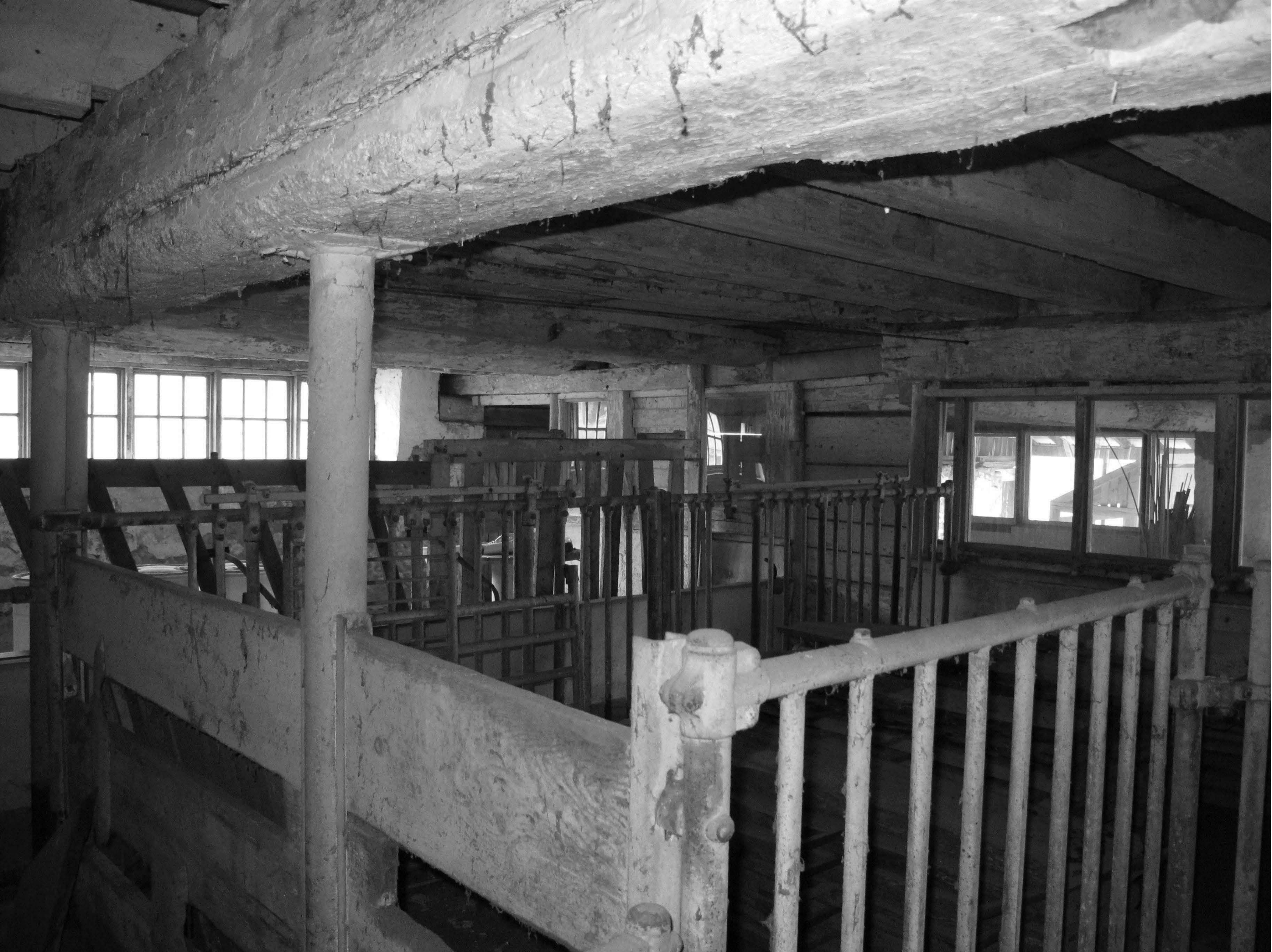
Cox-Phillips-Mitchell Agricultural Complex_New Castle County_DE Dairy barn interior lower level looking east
