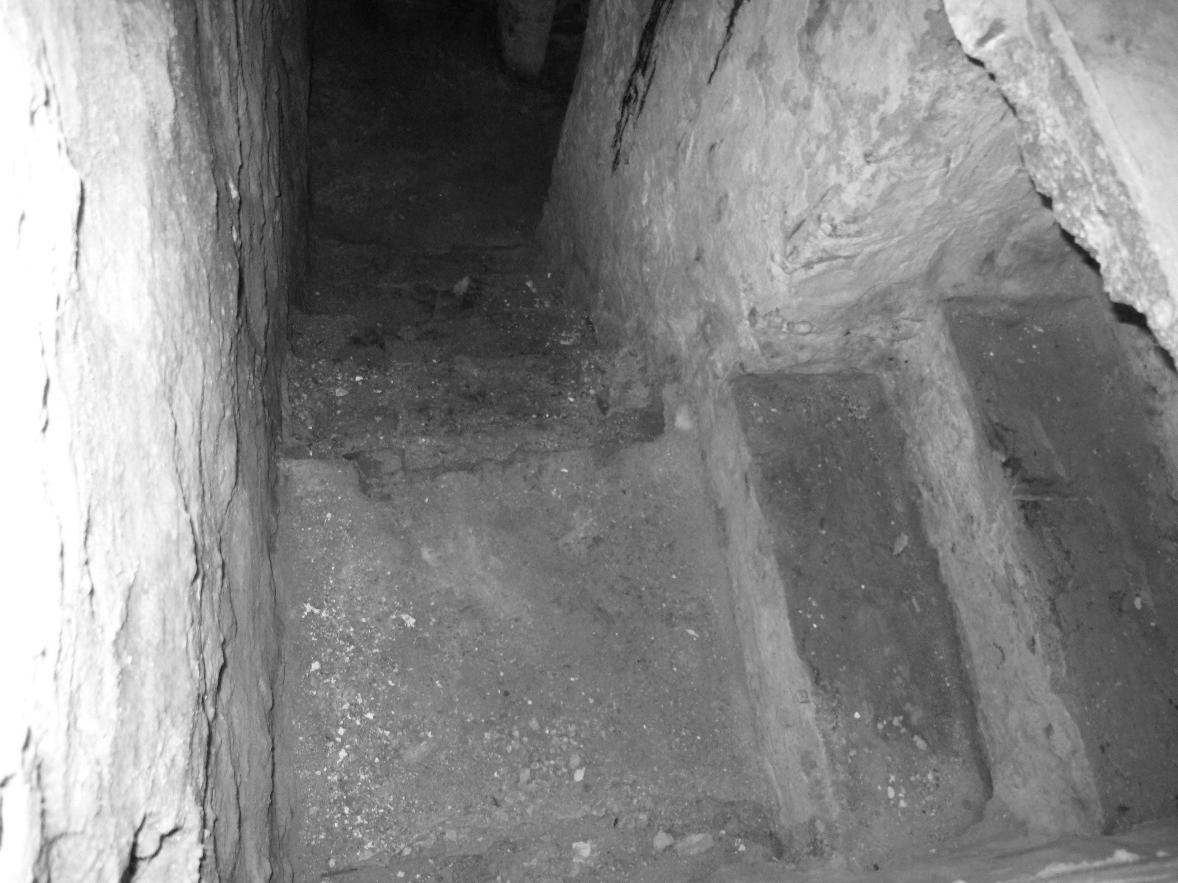
Cox-Phillips-Mitchell Agricultural Complex_New Castle County_DE Basement interior looking down the stairs into the subterranean vault looking northeast
