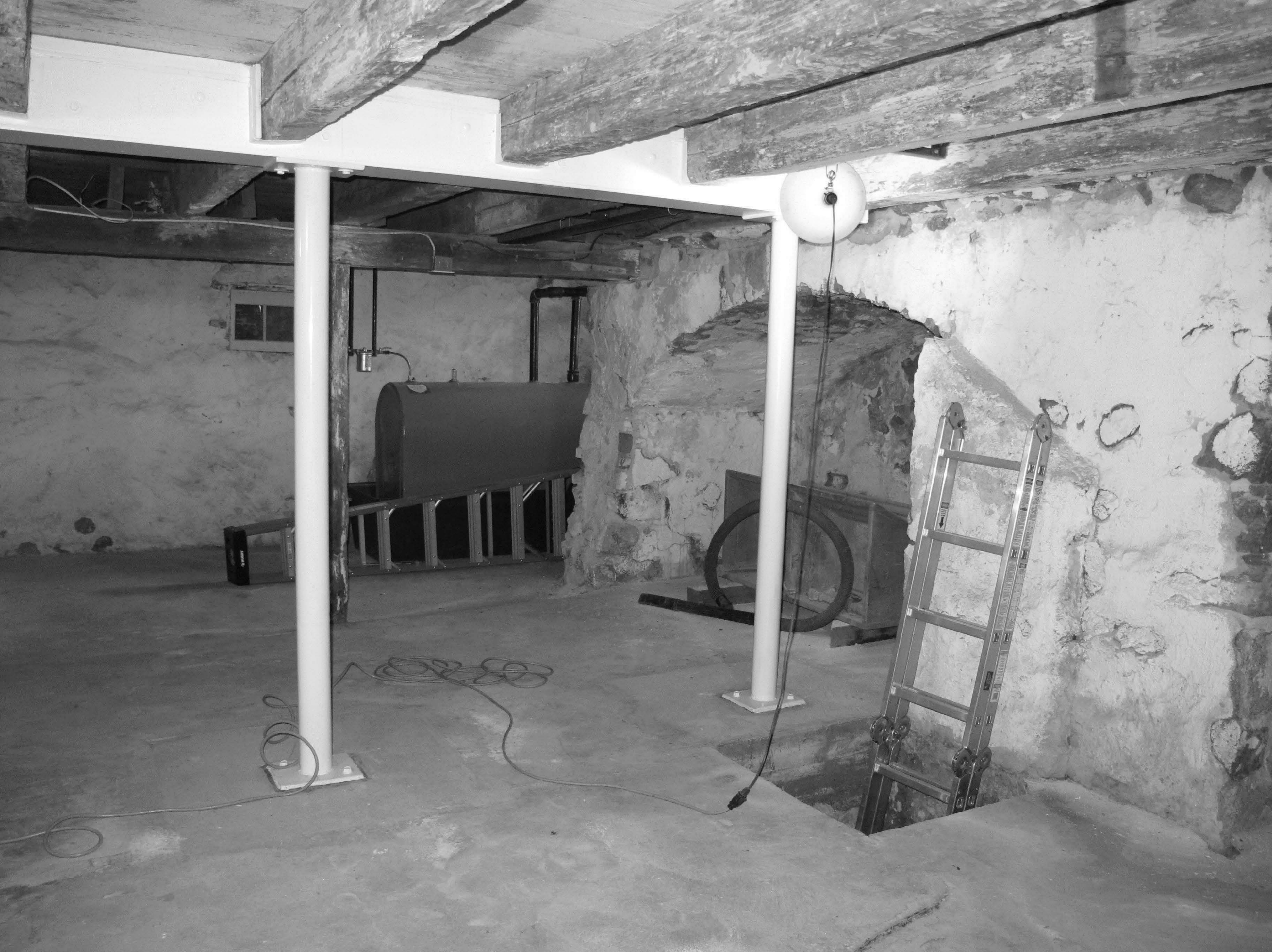
Cox-Phillips-Mitchell Agricultural Complex_New Castle County_DE Basement interior view of southwest wall, relieving arch on northwest wall, and floor opening to subterranean vault looking west
