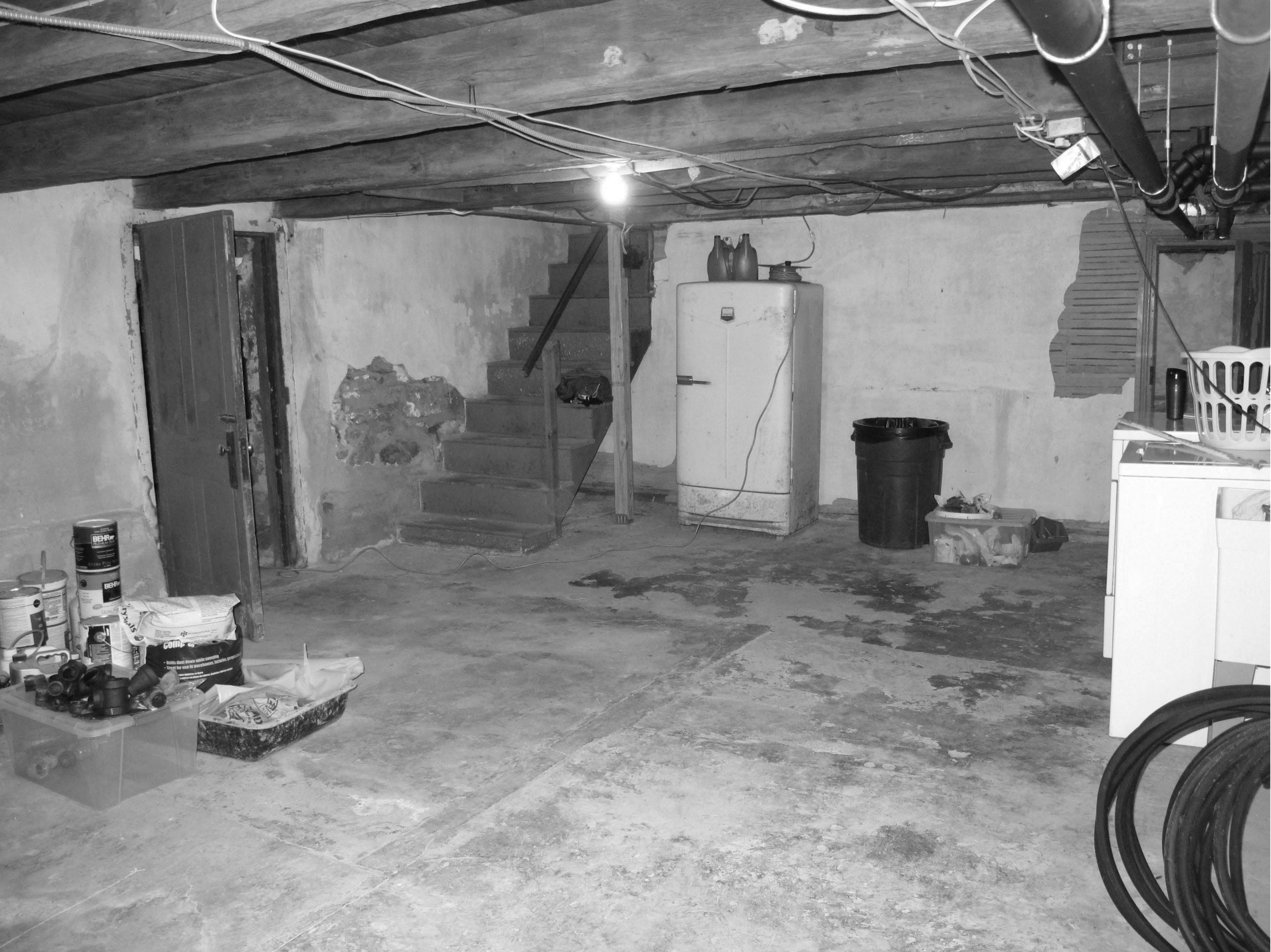
Cox-Phillips-Mitchell Agricultural Complex_New Castle County_DE Basement interior view of northeast and northwest walls showing stairs looking north
