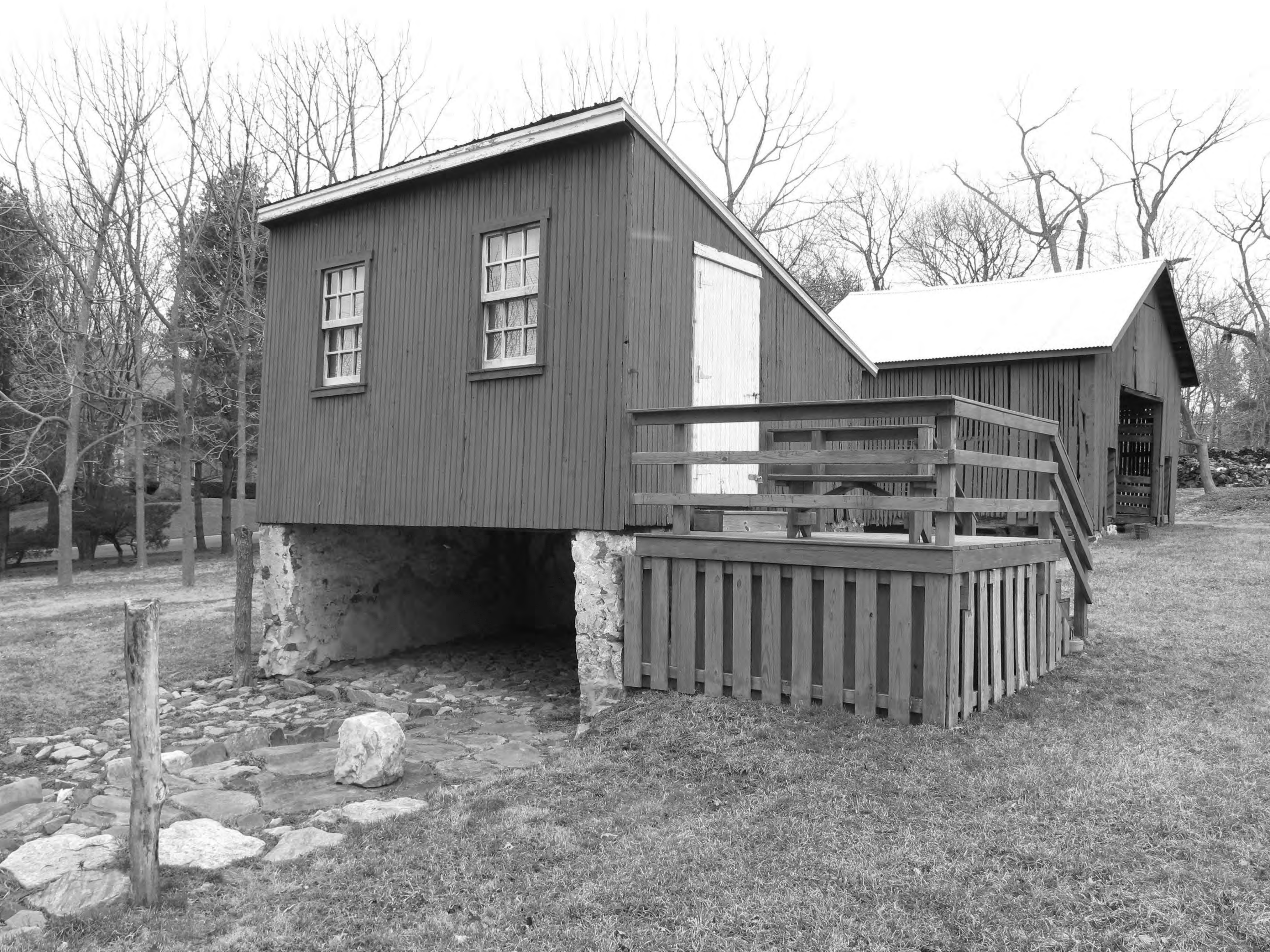
Cox-Phillips-Mitchell Agricultural Complex_New Castle County_DE Perspective view of piggery showing southwest and southeast elevations looking north
