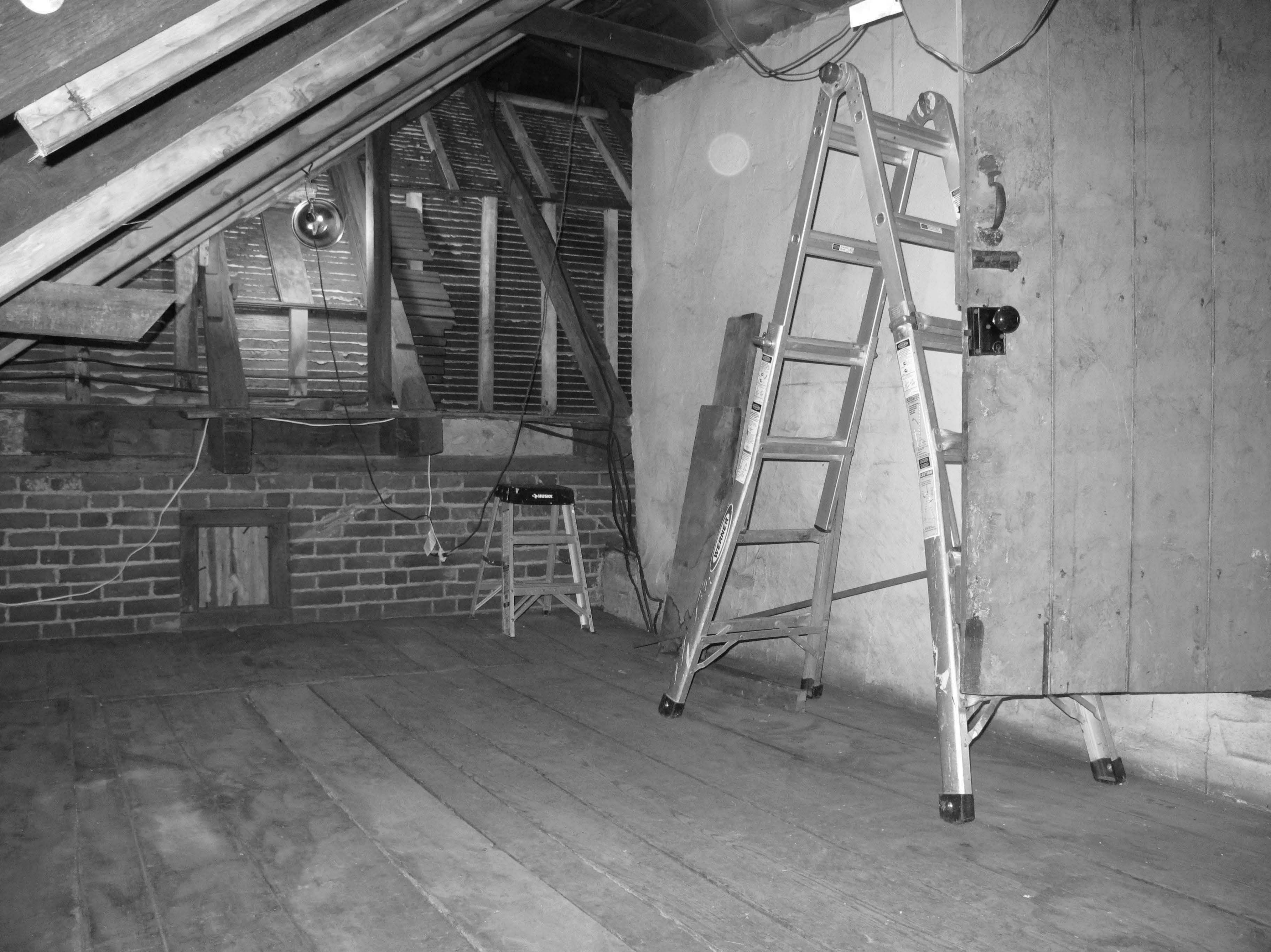
Cox-Phillips-Mitchell Agricultural Complex_New Castle County_DE Attic interior showing Period I roof framing system, looking south
