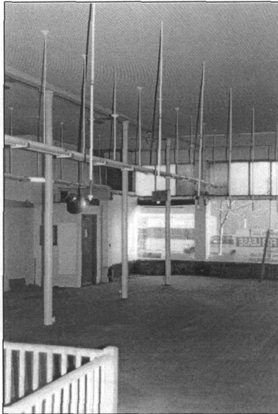
Figure 17: Tapered cast iron columns on centerline of 520-522 East Grand, view southeast (photo by James Jacobsen, February 2007)
