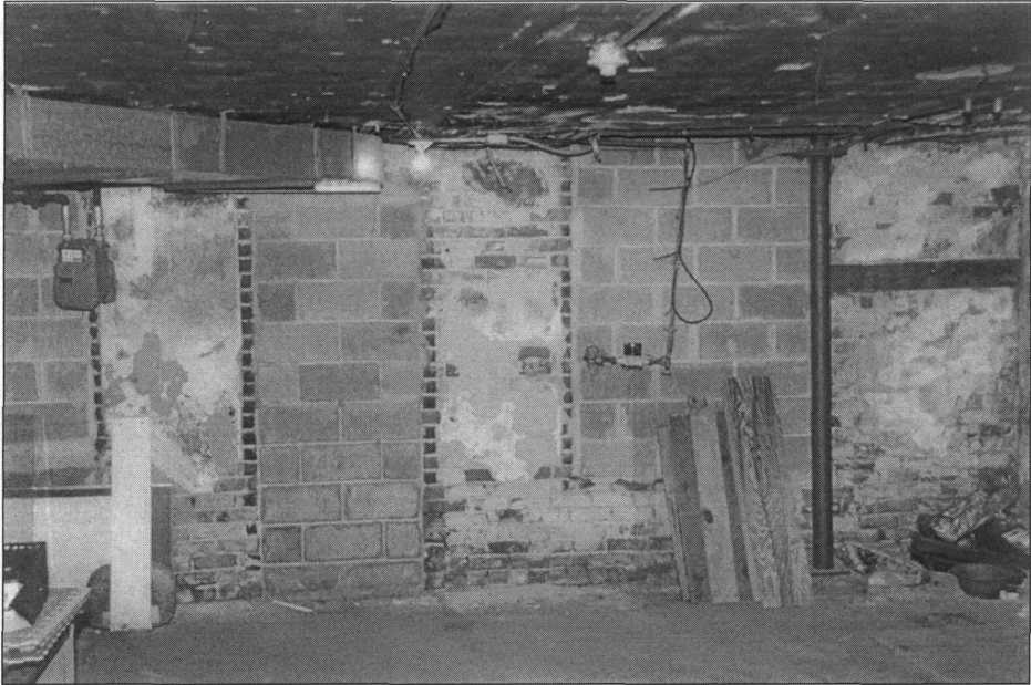
Figure 2: Brick filled windows and doorways in 516 East Grand, south wall, view southeast (photo by James Jacobsen, February 2007)
