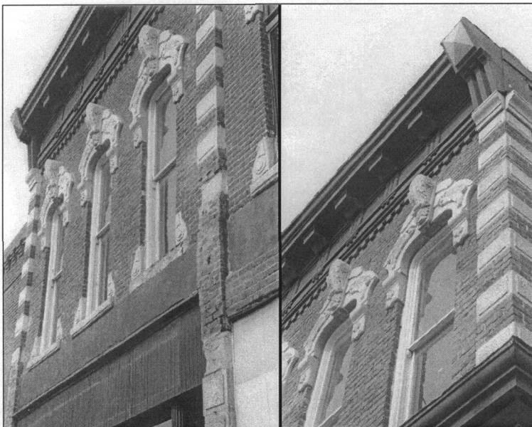
Figures 4-5: Details of upper façade levels, 516 and 526 East Grand Avenue, respectively (photo by James Jacobsen, February 2007)
