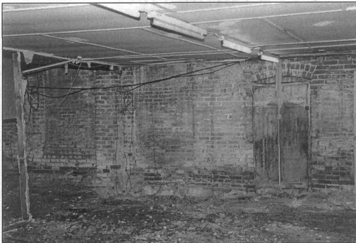
Figure 3: Brick filled windows and doorways in 520-522 East Grand, south wall, view southeast (photo by James Jacobsen, February 2007)
