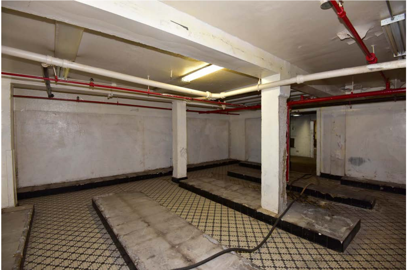
Figure 13: Second Floor, Block A, historic men's locker room; note raised areas from locker rooms. Source: Brad Finch, f-stop Photography, 2015.
