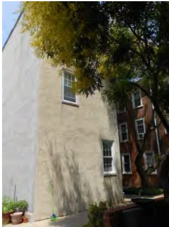
Photograph 20: 719 N. 8 th St. – Single Townhouse – Courtyard Elevation – Facing W (PFA, 2014) PA_Philadelphia_Friends Housing Cooperative_0020
