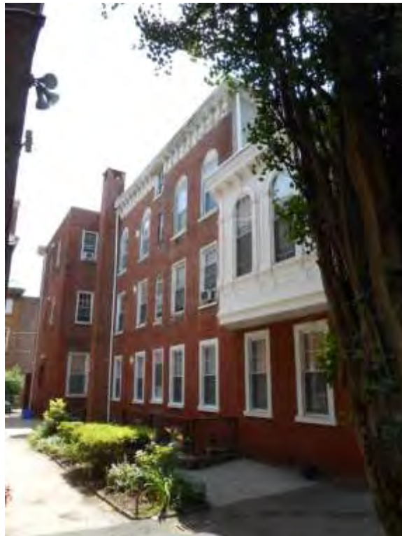
Photograph 14: 704-706 Franklin St – Alley Elevation from Courtyard- Facing SE (PFA, 2014) PA_Philadelphia_Friends Housing Cooperative_0014
