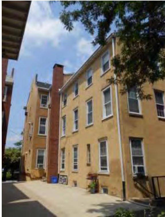
Photograph 17: 705-707 N. 8 th St – South Alley Elevation from Courtyard - Facing NW (PFA, 2014) PA_Philadelphia_Friends Housing Cooperative_0017
