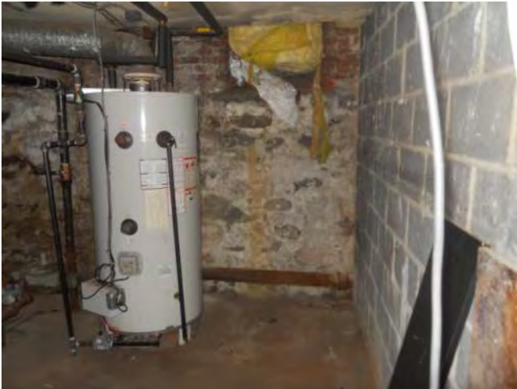
Photograph 36: Basement – Typical Boiler Room (PFA, 2014) PA_Philadelphia_Friends Housing Cooperative_0036
