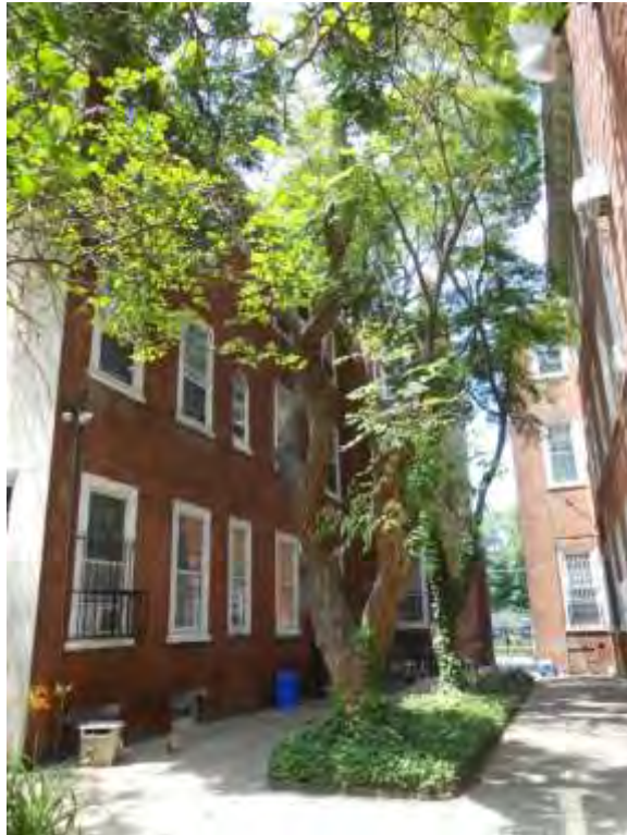
Photograph 22: 719 N. 8 th St. – Single Townhouse – North Alley Elevation – Facing SW (PFA, 2014) PA_Philadelphia_Friends Housing Cooperative_0022
