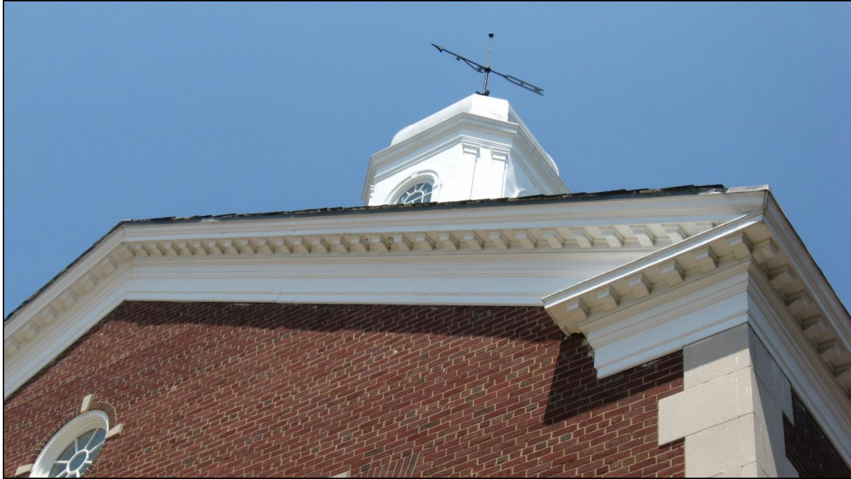
Photo 5: Detail of Cornice on Central Block, Looking Northeast EHT Tracerics, Inc., June 2014
