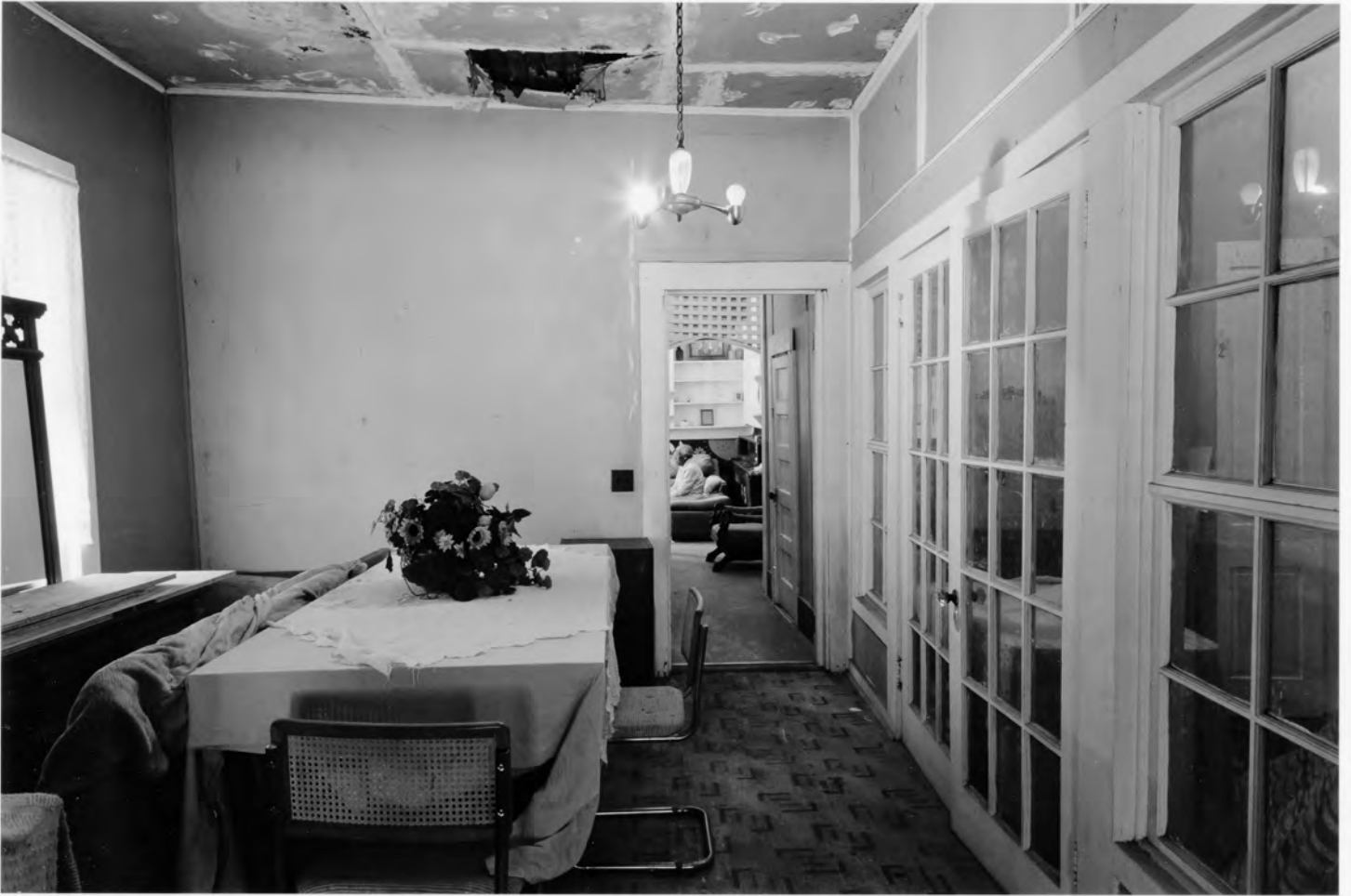
Georgia Williams Nursing Home Mitchell County, Georgia Photograph 13 of 22
