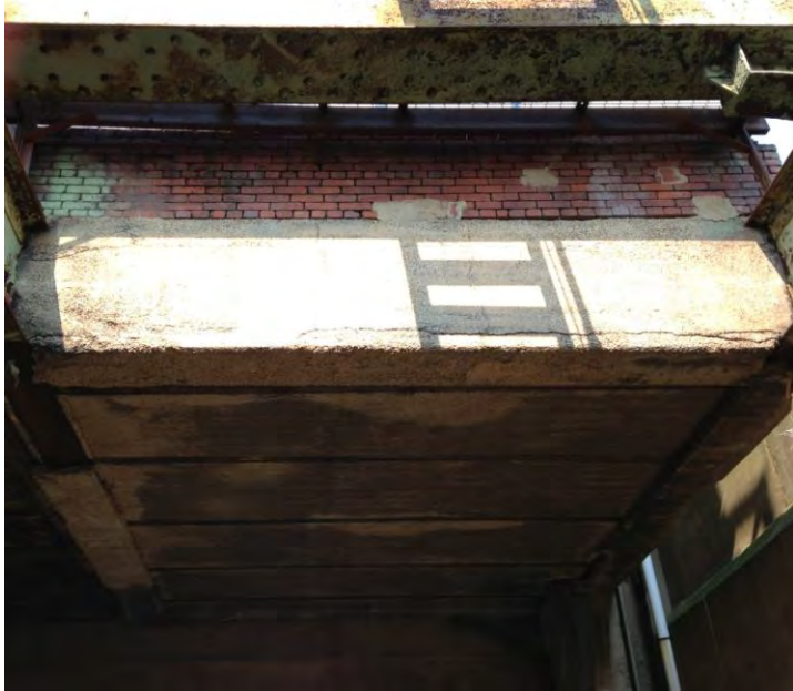
Figure 2. Steel girder and concrete platform under Control Tower and its exterior basement wall.
