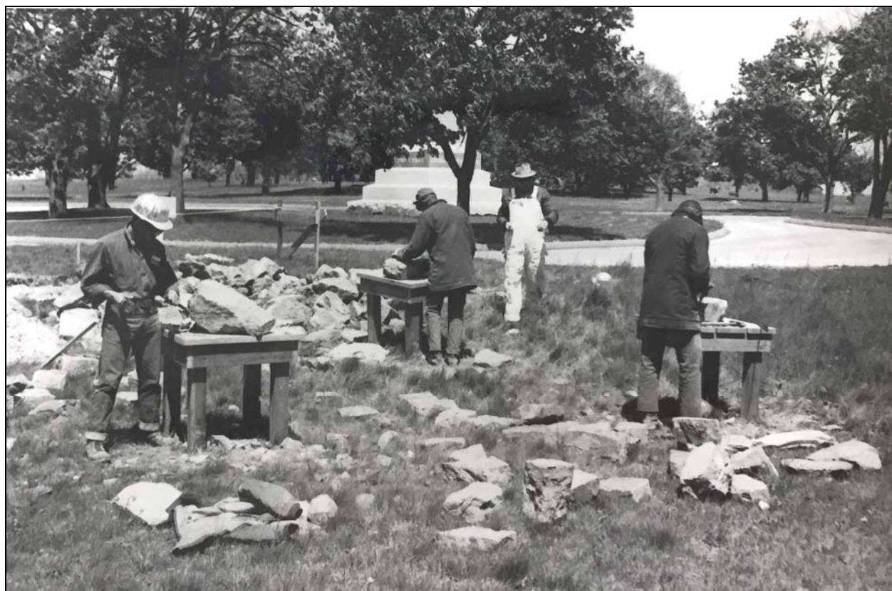
Figure 22. Construction of the interpretive exhibit at Philadelphia Brigade Park by the Harpers Ferry Job Corps, 1967. Source: Antietam National Battlefield Archive.
