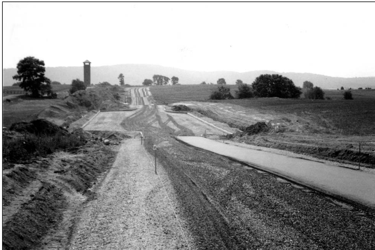
Figure 20. Realignment of Richardson Avenue and the construction of the Bloody Lane Overlook Parking Area, 1966. Source: Antietam National Battlefield Archives.
