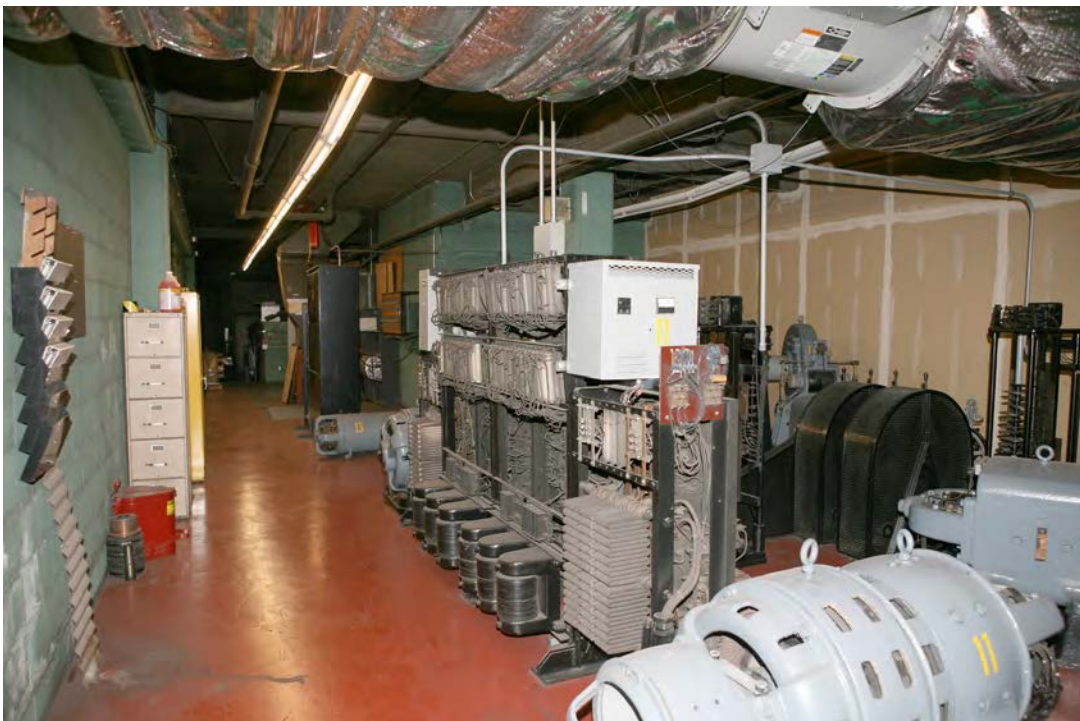
22 of 27. Bon Marche Building, penthouse mechanics.
