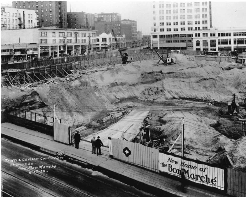
Historic Photograph 4. June 17, 1928. Excavation of Bon Marche Building site. Source: Museum of History and Industry.
