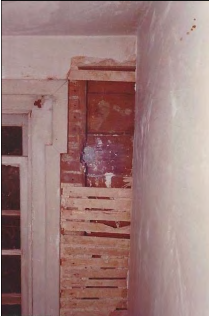
Historic Photo 5 of 5 Detail of corner, second-story bedroom: damaged post and lath, hole in weatherboarding caused by 1865 shelling.
