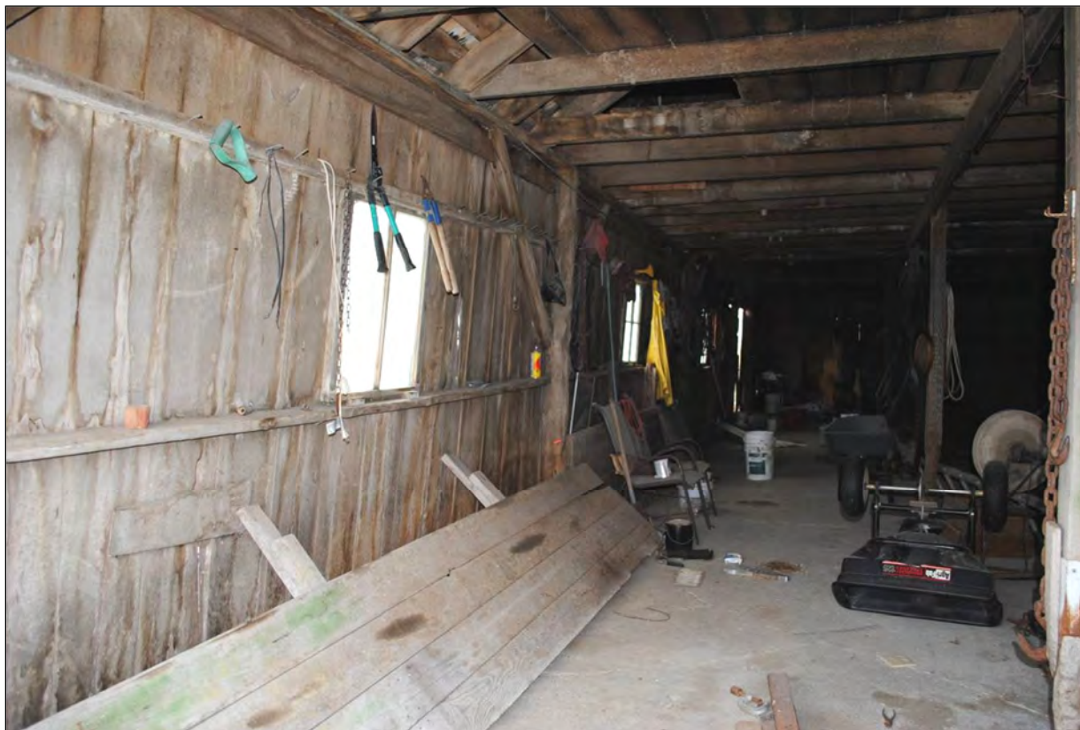
Figure 11. Interior view of the Middle Barn's west wall and alley looking north. The vertical posts along the exterior of the alley walls are debarked poles. Photograph taken by Tallgrass Archaeology LLC, 04/13/2018.
