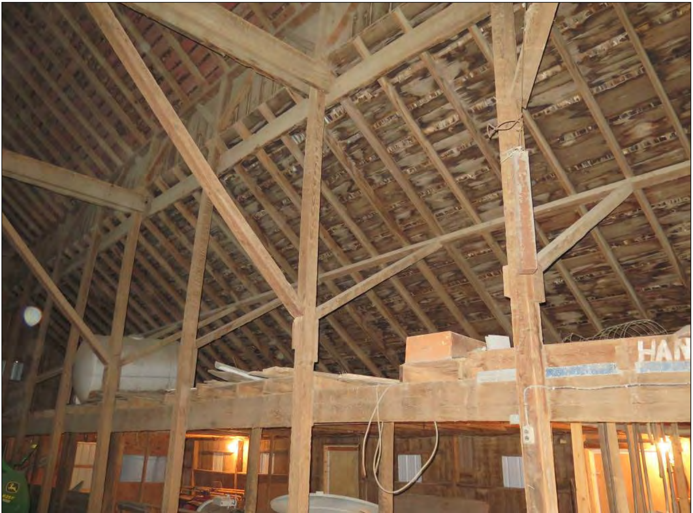
Figure 35. Interior framing of North Barn looking NW towards the loft space on the north side of the barn.
