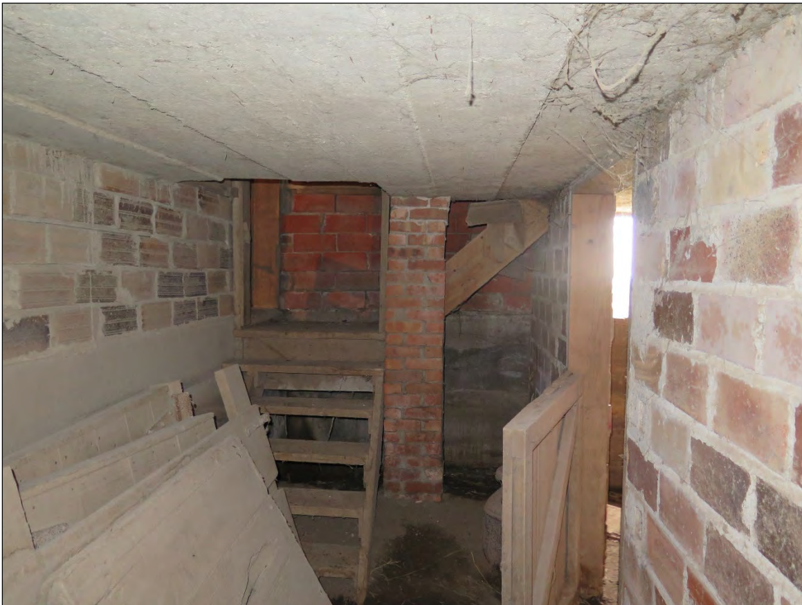
Figure 22. Interior of basement alley looking south at the wooden stairs and landing that lead down to the basement alley and up to the ground level of the main barn. Note the brick pier that supports the concrete ceiling above and to which the staircase is fixed. Photograph taken by Tallgrass Archaeology LLC, 04/13/2018.
