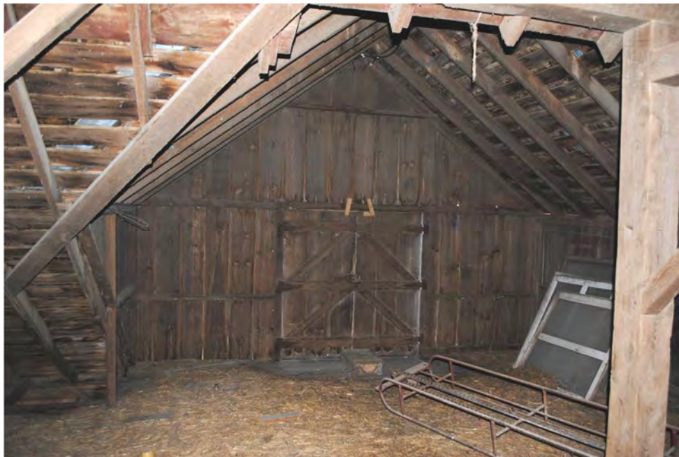
Figure 16. Interior of the gabled dormer in the Middle Barn's hay mow. Photograph taken by Tallgrass Archaeology LLC, 04/13/2018.
