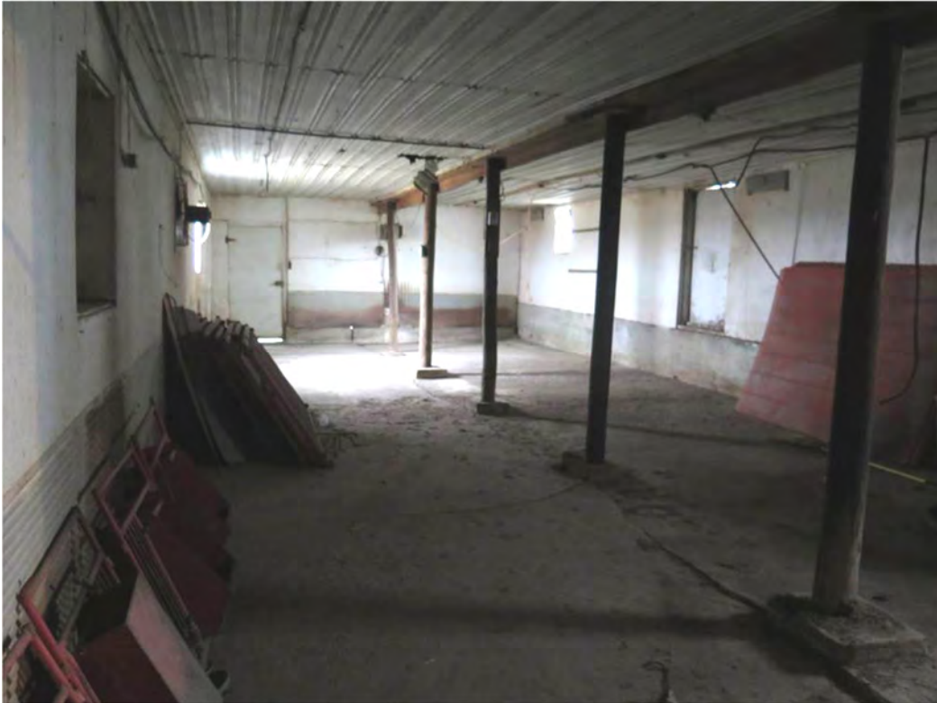
Figure 25. Open interior of the south wing of the South Barn looking south. Here the center poles are wooden. Photograph taken by Tallgrass Archaeology LLC, 04/13/2018.
