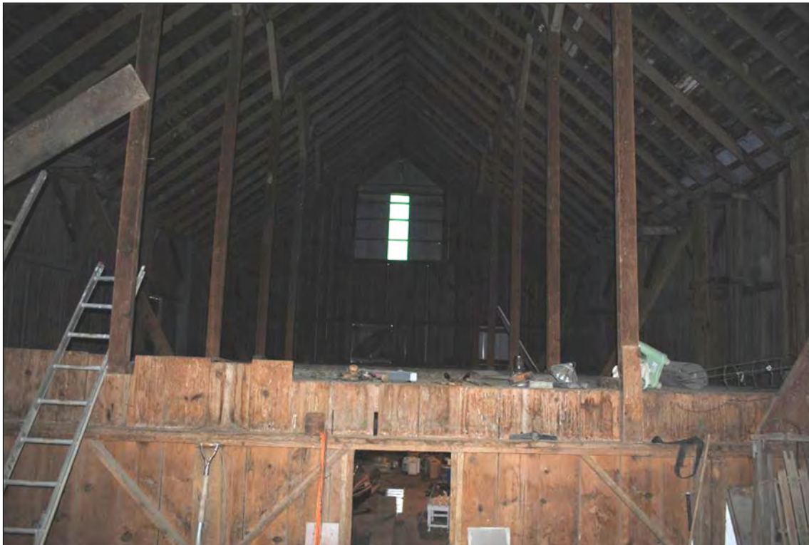
Figure 26. Hay mow above the main body of the barn looking west into the loft from the lower loft of the wings. The small portal visible in the east wall just below the loft opening is the current access from the ground level of the front-gabled barn to the loft. Photograph taken by Tallgrass Archaeology LLC, 04/13/2018.
