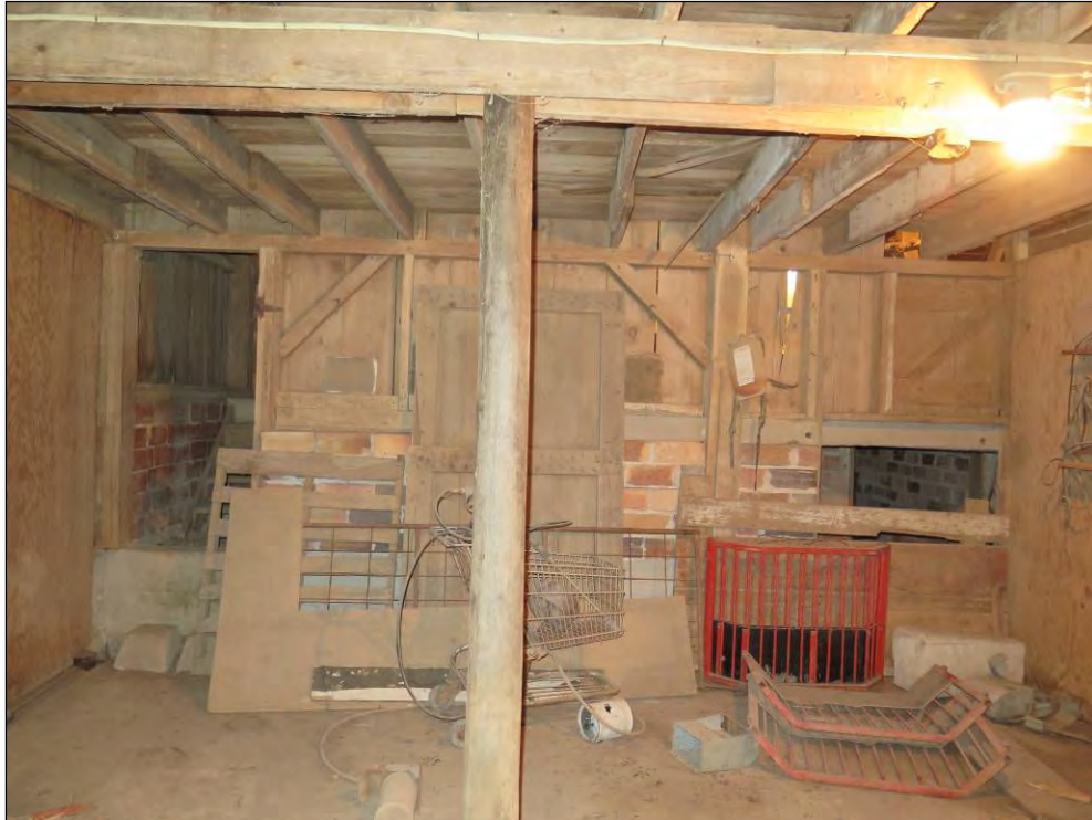
Figure 23. Center room of the South Barn off the east end of the front-gabled barn and connecting the north and south wing additions looking west. Beyond that wall is the main part of the barn, the north and south wings can also be accessed from this room, to the right and left of this room. Photograph taken by Tallgrass Archaeology LLC, 04/13/2018.
