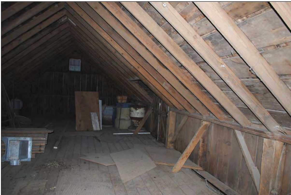
Figure 28. Loft above the south wing looking south. Photograph taken by Tallgrass Archaeology LLC, 04/13/2018.
