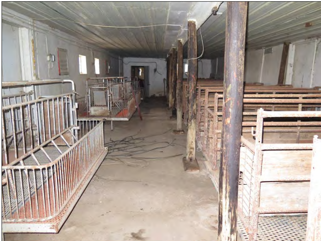
Figure 24. Main level of the north wing of the South Barn looking south. The wing is lined with metal farrowing pens for the later hog operation. Here the center poles are metal. Photograph taken by Tallgrass Archaeology LLC, 04/13/2018.
