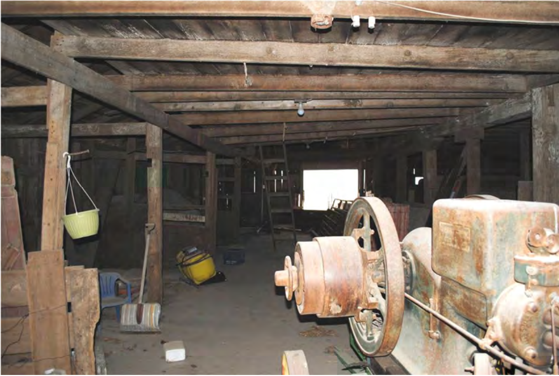
Figure 12. One of the interior alleys of the Middle Barn, where animals were often showed. A variety of joining methods were used in the construction of this barn. Mortise-and-tenon can be seen with some of the heavier framework, whereas simple nails hold some of the cross-beams together, here to add support to the loft floor from underneath. Photograph taken by Tallgrass Archaeology LLC, 04/13/2018.
