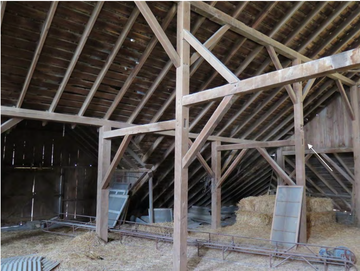
Figure 15. Interior framing of the loft in the Middle Barn's looking NW. Note the gabled dormer at the left in this photograph. White arrow points to a location where the cross beam is now missing between the center set of posts.
