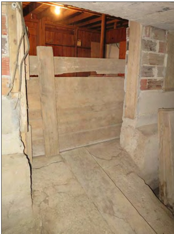
Figure 20. Ramp that descends into the basement alley below the main barn connecting to the middle room of the winged east sections of the barn. Photograph taken by Tallgrass Archaeology LLC, 04/13/2018.
