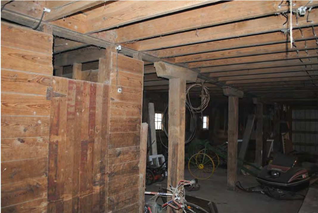
Figure 18. Main level of the South Barn's front-gabled original section looking WSW. Four rows of posts support the hay mow above. The oat bin is to left, with horse stalls to the west. Photograph taken by Tallgrass Archaeology LLC, 04/13/2018.
