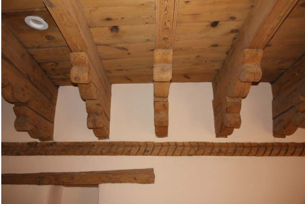
15 of 16. Interior, vigas and corbels above the choir loft, photographer facing south.
